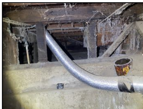
Flexible vent under structure - needs to be serviced
