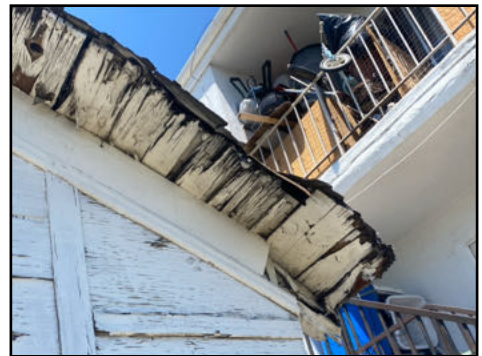
Heavily damaged - needs to be replaced
