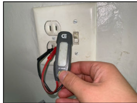
Non-energized (dead) outlet(s) - needs to be serviced
