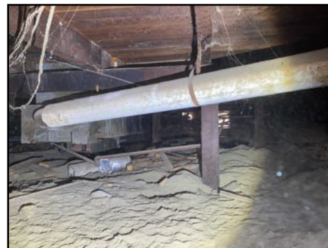
Older cement (AKA transite) flue pipe present - it is recommended to upgrade these areas
