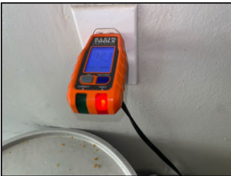
Outlet hot wired in reverse with neutral - needs to be serviced
