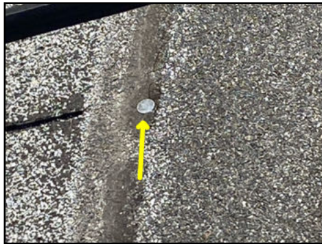
Exposed nails/staples/screws on roofing material - recommend sealing all fastener heads
