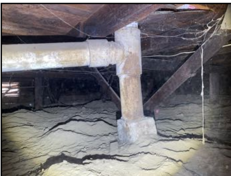
Older cement (AKA transite) flue pipe present - it is recommended to upgrade these areas
