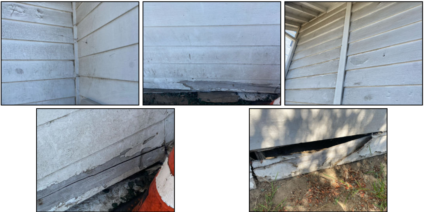
Cracking/chipping/holes more than typical - needs to be serviced
