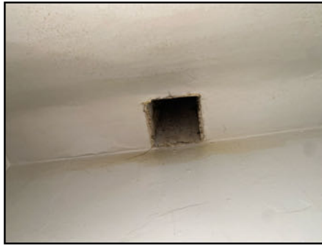
Greasy/dirty unit - recommend cleaning
