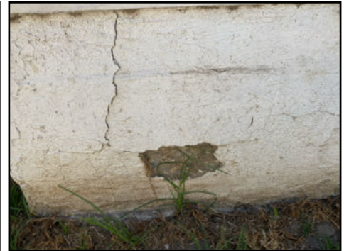
Blistered due to unknown reason - needs to be serviced
