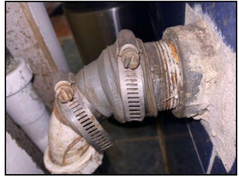
Rubber drain connections present - these are not for long term use - recommend upgrading connections
