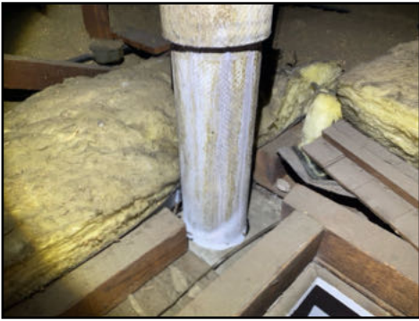
Masonry/cement/transite type vent pipe in the attic - needs to be serviced and possibly upgraded to newer style vents
