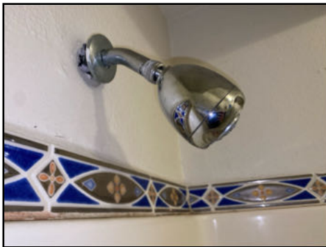
Diverter does not properly divert water to shower head - needs to be serviced (hall south)
