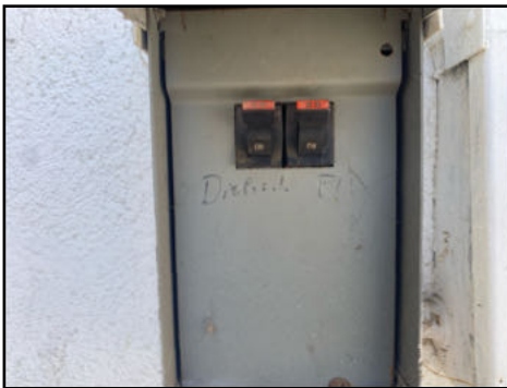
Manufacture of panel a brand (Federal Pacific) known for frequent issues - recommend further evaluation by a licensed electrician
