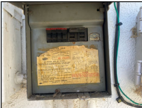
Manufacture of panel a brand (Federal Pacific) known for frequent issues - recommend further evaluation by a licensed electrician
