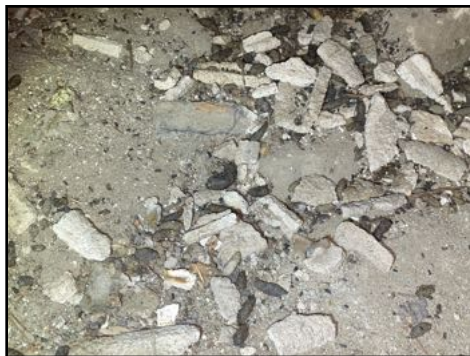
Evidence of rodent/pest activity in the crawlspace - recommend further evaluation by pest services company
