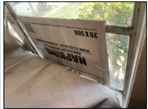
Hole in glass- needs to be serviced
