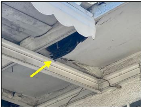
Heavily damaged - needs to be replaced
