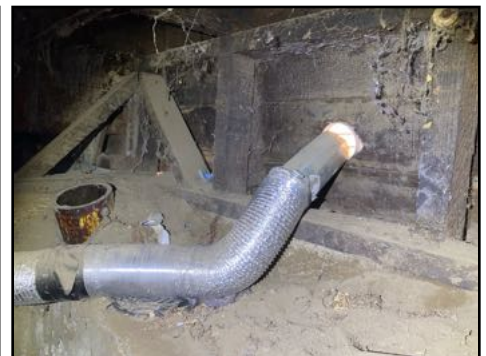
Flexible vent under structure - needs to be serviced
