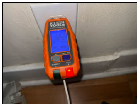
Outlet hot wired in reverse with neutral - needs to be serviced
