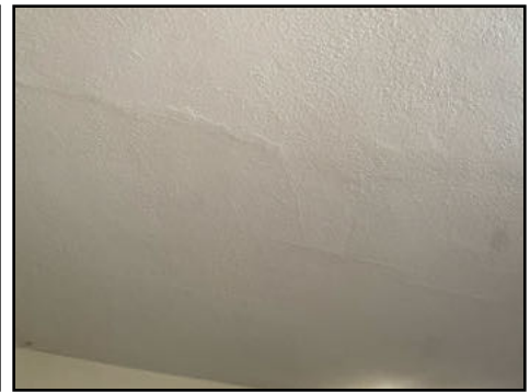
Patched/partial painted areas present - consult seller regarding patched areas
