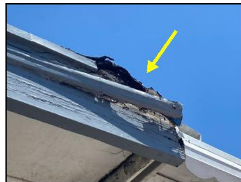
Cracking/deterioration - more than normal - needs to be serviced
