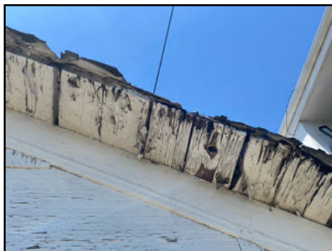
Heavily damaged - needs to be replaced
