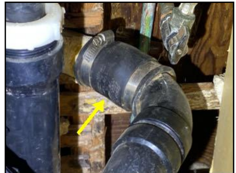
Rubber drain connections present - these are not for long term use - recommend upgrading connections
