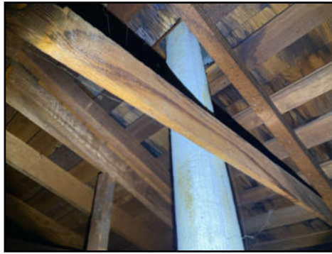
Masonry/cement/transite type vent pipe in the attic - needs to be serviced and possibly upgraded to newer style vents
