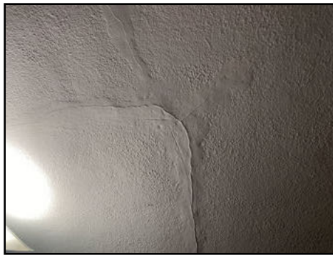
Patched/partial painted areas present - consult seller regarding patched areas
