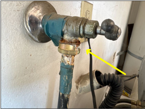
Supplies corroded – service recommended
