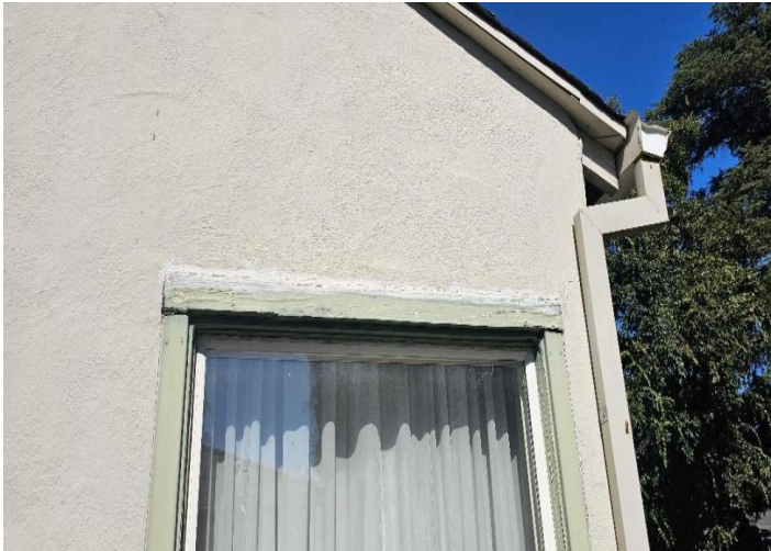
3B - Damaged window members.
