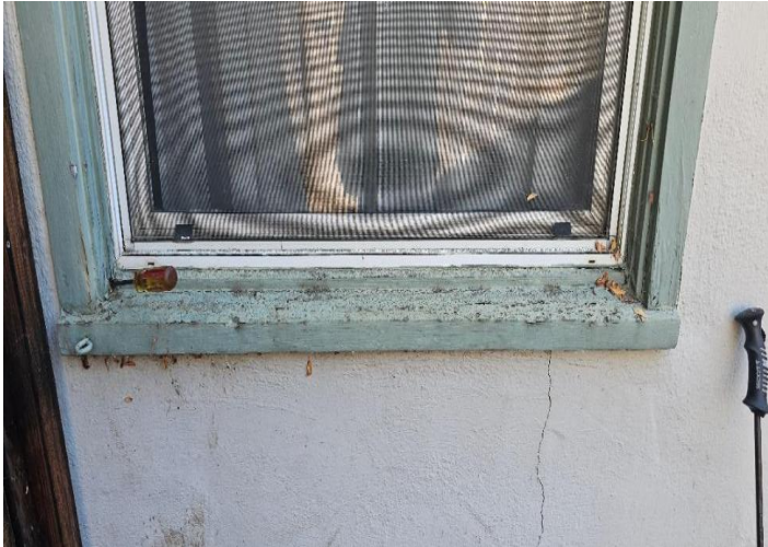
3B - Damaged window members.
