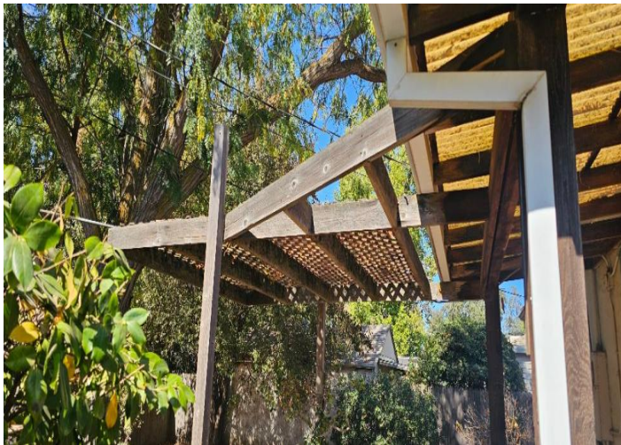
3C - Damaged arbor assembly.
