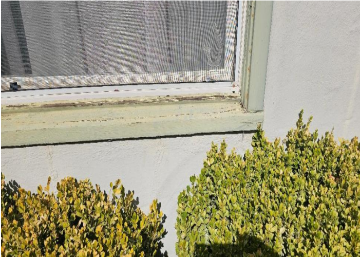
3B - Damaged window members.
