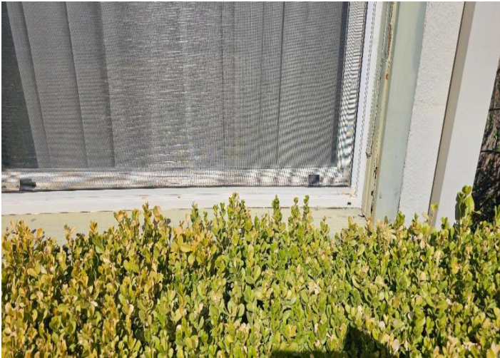
3B - Damaged window members.
