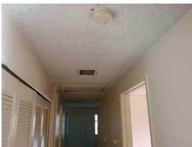
Sub CO Monitor/Smoke Alarm
