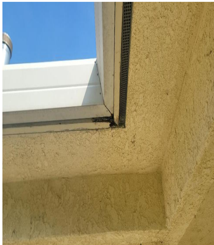
3C - Damaged roof fascia from leaking gutters.
