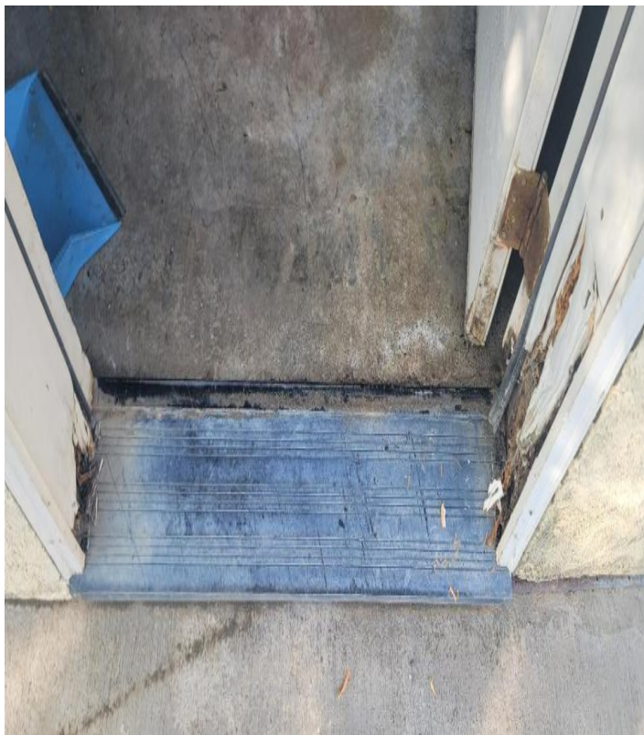
3B - Damaged door, door jambs, frame and trim on the detached shop.
