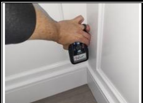
There is elevated moisture on the north wood panel wall in the NE corner.
