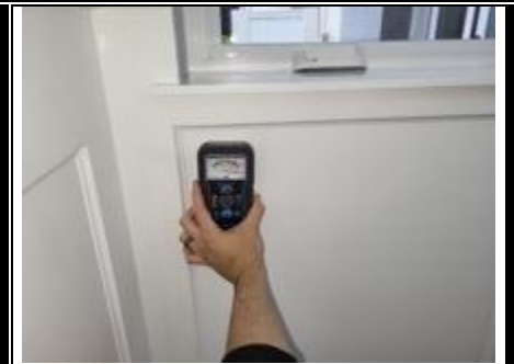
There is elevated moisture on the east wood panel wall under the east window.
