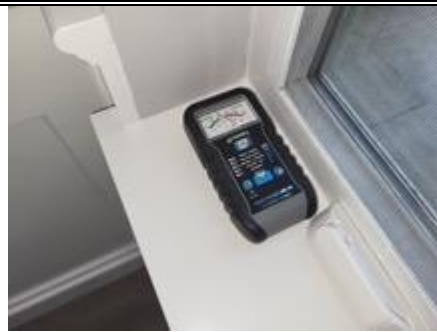
There is elevated moisture on the base of the east window.
