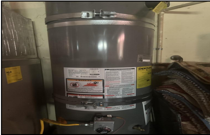
STRAPPED WATER HEATER
