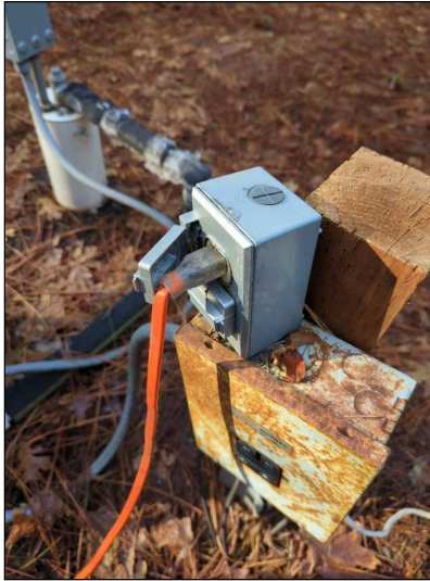
Not GFCI protected.
