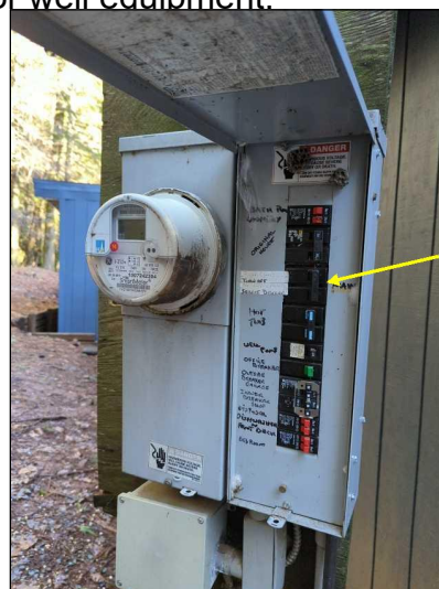
Main power disconnect.
