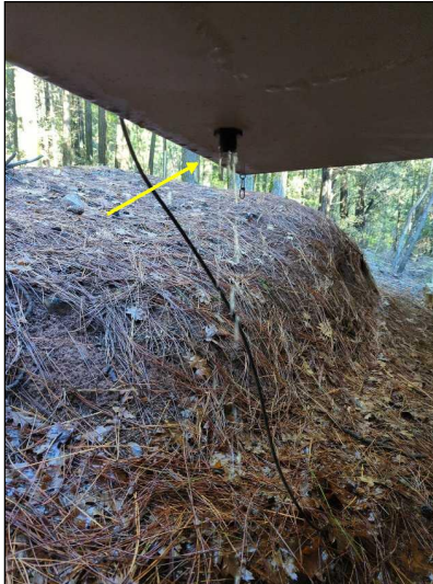
Float may be stuck at swamp cooler.
