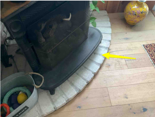
Undersized hearth extension over combustible materials
