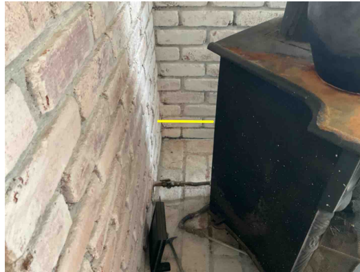
Inadequate clearance to the wall
