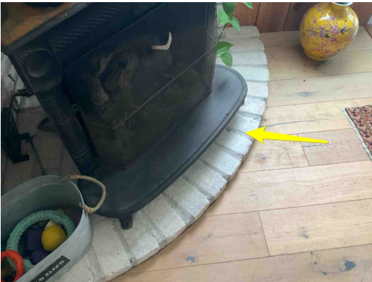
Undersized hearth extension over combustible materials
