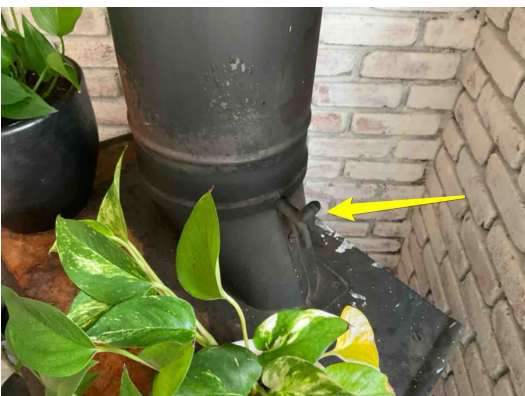
Functional damper on a fuel burning appliance
