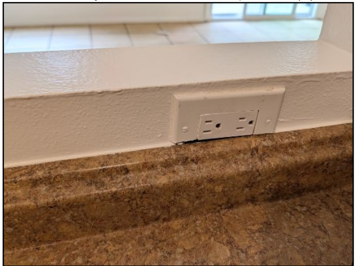
Outlet cover plates at the sink side countertop have been altered. The electrical boxes are partially obstructed by the laminate backsplash. * (5)
