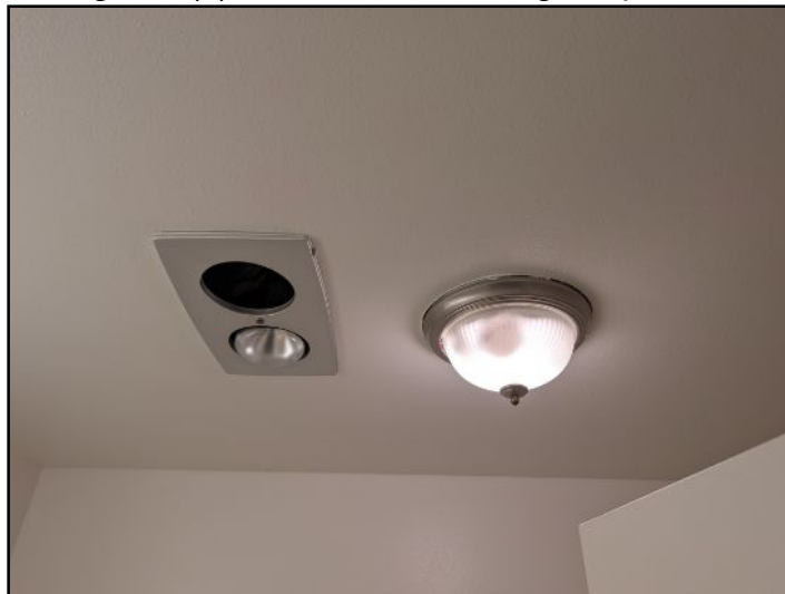
Missing bulb(s) noted at the heating lamps/fans. *
