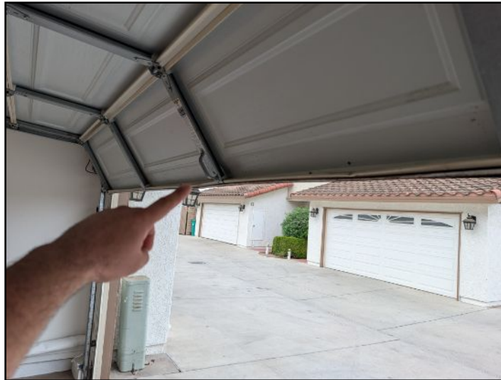
Damaged and/or warped panels noted at the garage vehicle door. *
