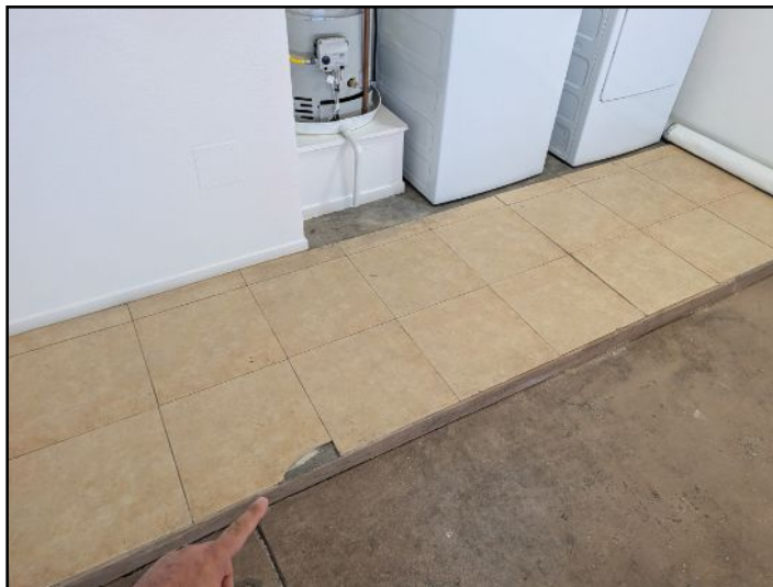
Cracked floor tile noted in garage. * (5)
