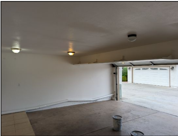
A garage light fixture is not operational or needs bulb replaced. (2)
