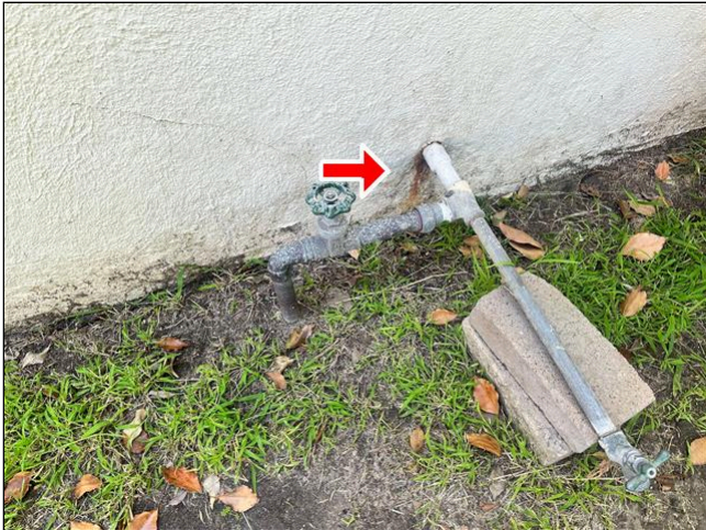
Item 6 - Item 1 (Picture) Plumbing System
