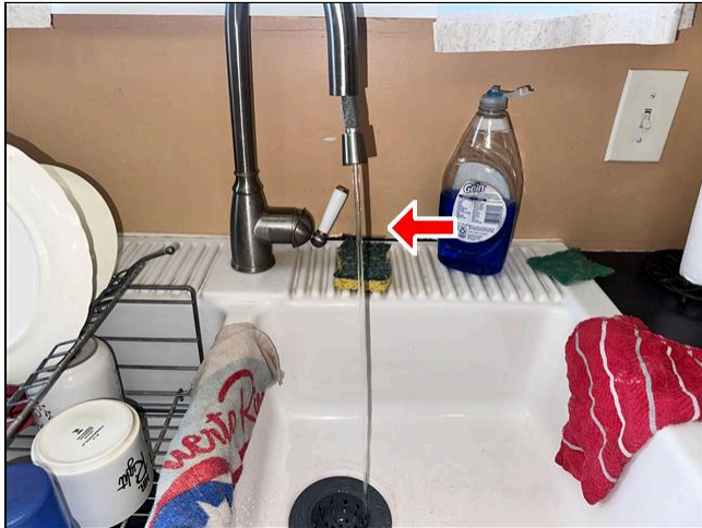
5.1 Item 4 (Picture) Plumbing System
