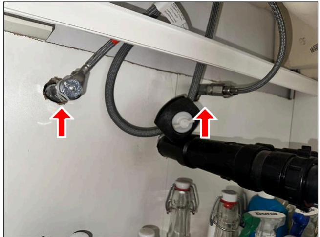
5.1 Item 3 (Picture) Plumbing System
