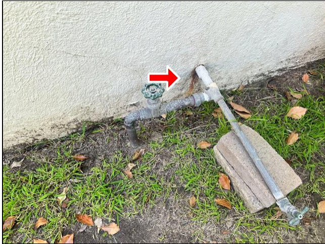
5.1 Item 1 (Picture) Plumbing System
