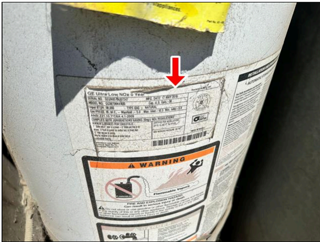
Item 10 - Item 1 (Picture) Plumbing System
