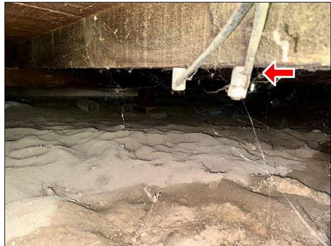
Item 12 - Item 2 (Picture) Electrical System
