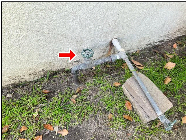
5.1 Item 5 (Picture) Plumbing System
