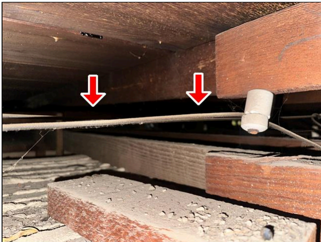
Item 12 - Item 1 (Picture) Electrical System
