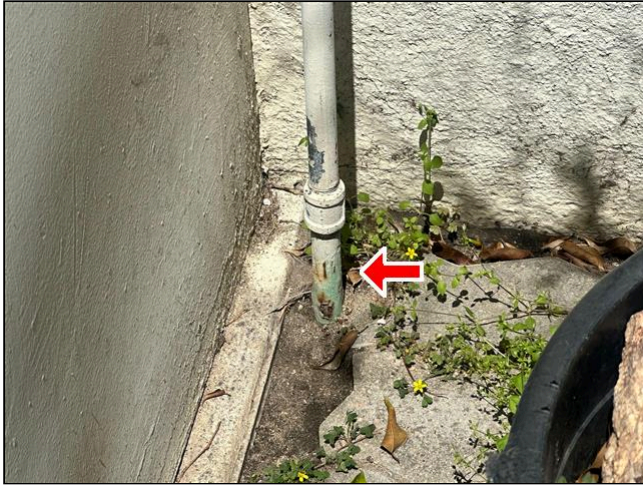
Item 11 - Item 1 (Picture) Plumbing System
