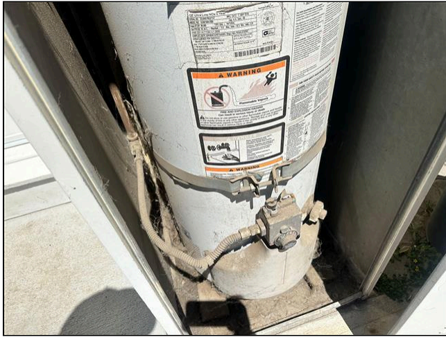
5.4 Item 2 (Picture) Plumbing System
