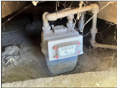
5.5 Item 2 (Picture) Plumbing System
