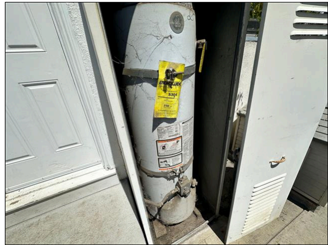
Item 10 - Item 2 (Picture) Plumbing System
