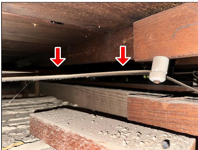
6.1 Item 1 (Picture) Electrical System
