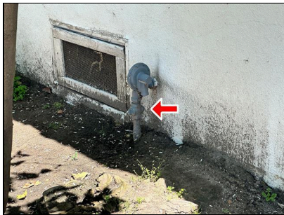
5.5 Item 1 (Picture) Plumbing System
