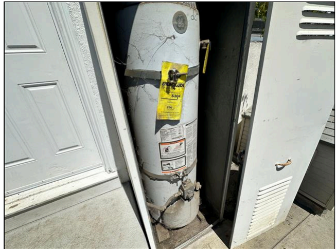
5.2 Item 3 (Picture) Plumbing System
