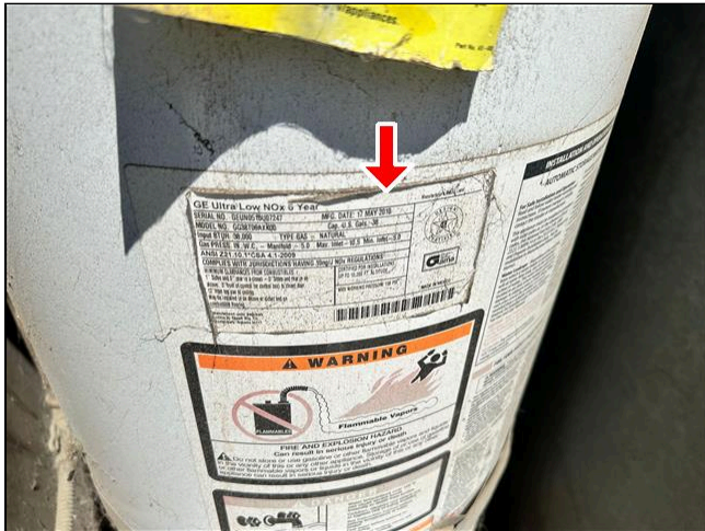
5.2 Item 2 (Picture) Plumbing System
