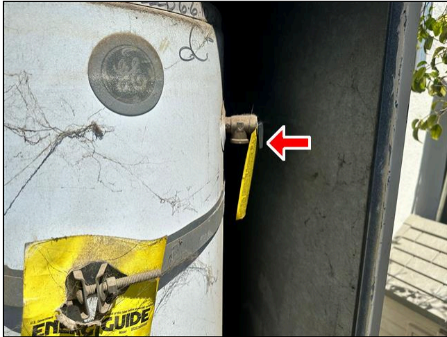
5.2 Item 1 (Picture) Plumbing System
