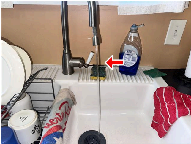
Item 8 - Item 1 (Picture) Plumbing System
