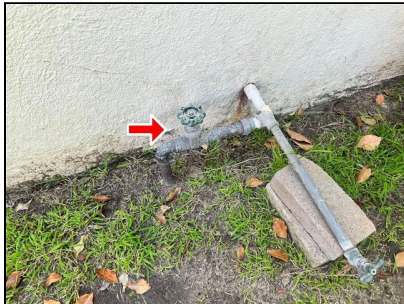
5.6 Item 1 (Picture) Plumbing System
