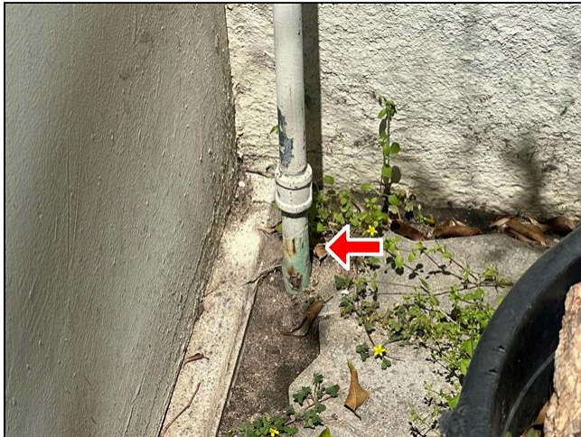
5.4 Item 1 (Picture) Plumbing System
