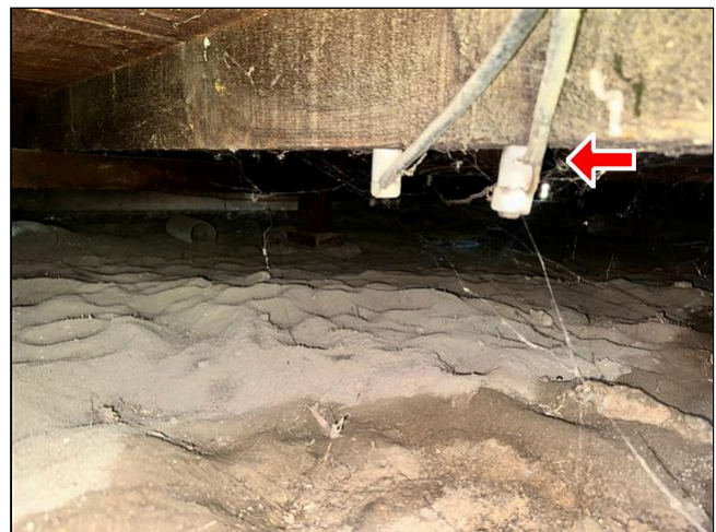
6.1 Item 2 (Picture) Electrical System
