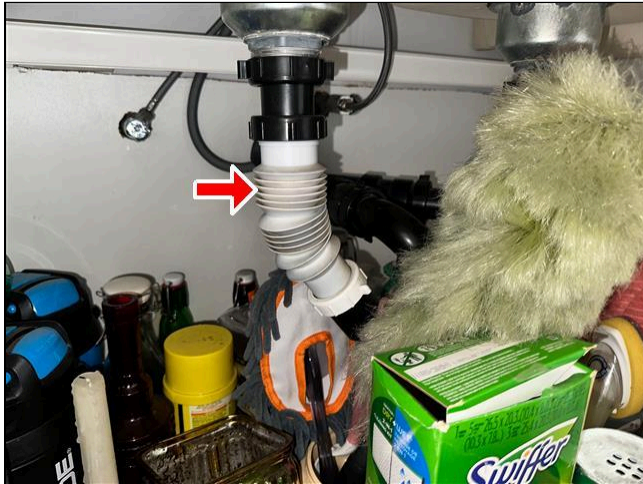
5.0 Item 1 (Picture) Plumbing System
