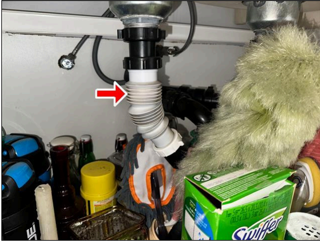
Item 5 - Item 1 (Picture) Plumbing System
