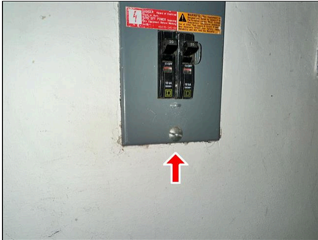
6.0 Item 1 (Picture) Electrical System
