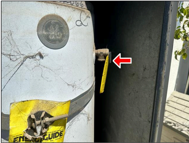
Item 9 - Item 1 (Picture) Plumbing System
