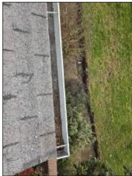
Partial rain gutter present - restricted / clogged with debris - needs to be serviced
