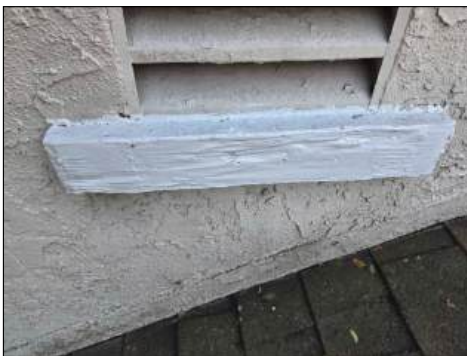
Deteriorated wood - consult termite report - recommend service - at roof area, back yard closet/storage areas
