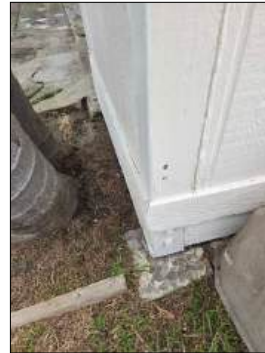
Deteriorated wood observed - recommend servicing
