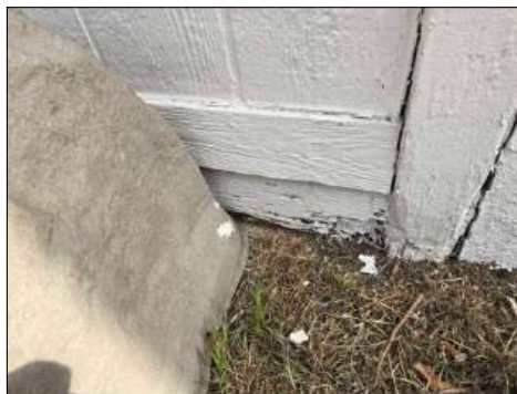
Deteriorated wood - consult termite report - recommend service - at roof area, back yard closet/storage areas
