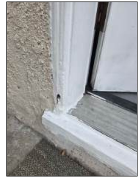
Moisture damage/deteriorated wood at exterior door/door jamb - needs to be serviced - west
