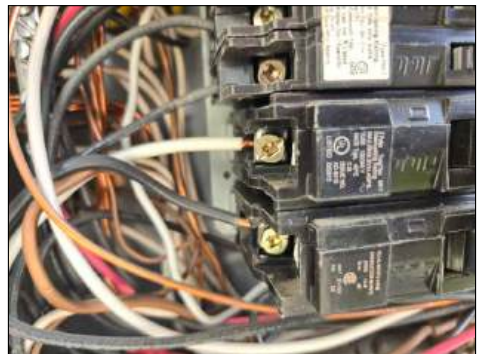
White or green wires at breaker(s) - needs to be serviced/further evaluated by an electrician
