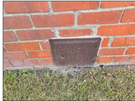
Chimney clean out door worn/rusted/loose - recommend service
