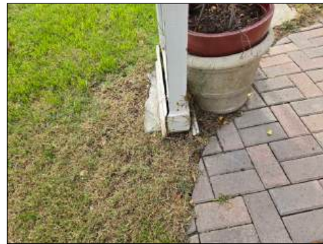
Loose/damaged/missing trim at base - needs to be serviced
