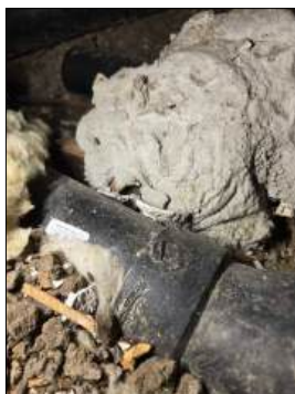
Evidence of rodent/pest activity in the crawlspace - recommend further evaluation by pest services company
