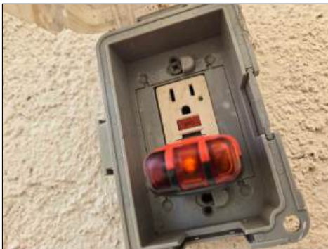
GFCI not grounded - recommend servicing
