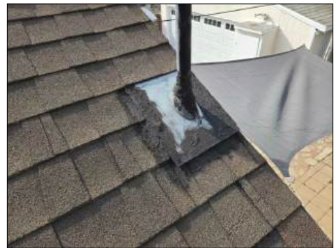
Irregular installation at electrical feeds - needs to be serviced/further evaluated
