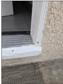
Moisture damage/deteriorated wood at exterior door/door jamb - needs to be serviced - west
