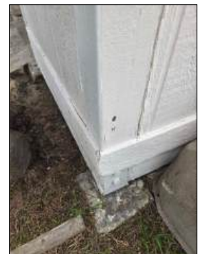
Deteriorated wood - consult termite report - recommend service - at roof area, back yard closet/storage areas
