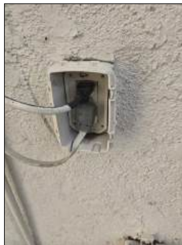
Missing/damaged exterior cover - recommend servicing - by water heater
