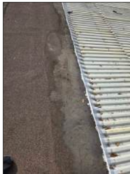
Ponding or evidence of ponding in areas - needs to be serviced
