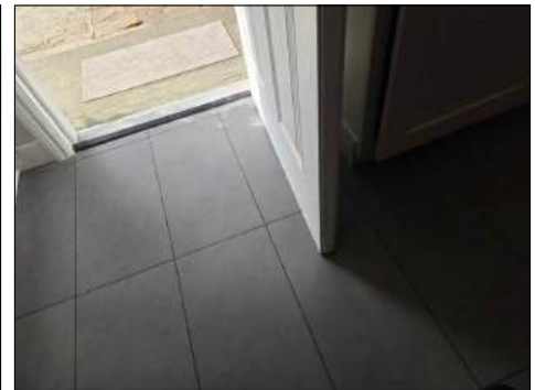
Drags on floor - recommend servicing - at kitchen
