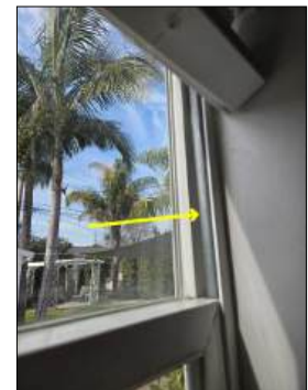
Loose/broken sash springs or cables - possible safety concern - recommend service - at bedroom southeast, master bathroom, living room
