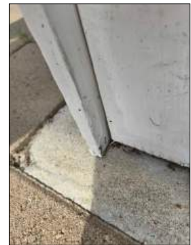
Deteriorated wood at support post(s) - Needs to be further evaluated by a licensed contractor for safety
