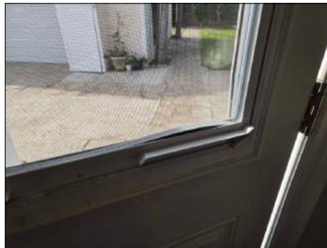
Inner seals at double pane windows are bulging/moving due to heat - recommend servicing - at kitchen
