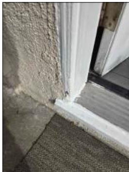
Moisture damage/deteriorated wood at exterior door/door jamb - needs to be serviced - at kitchen
