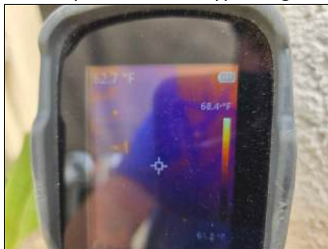
Thermal Image View - Normal temperature readings with no visible signs of overheating at time of inspection
