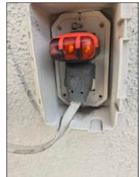
Tested and operational at time of inspection via normal control - southwest
