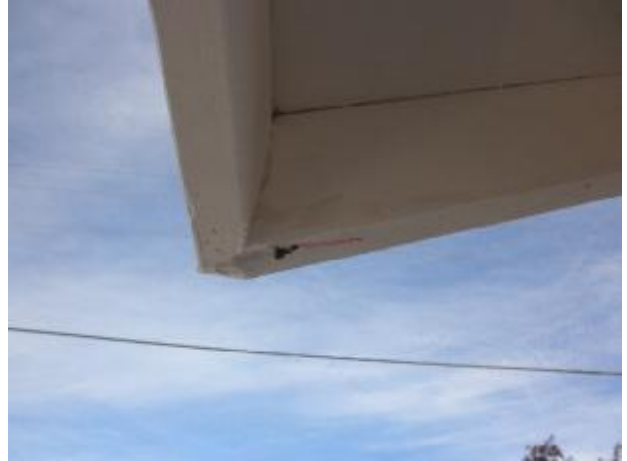
Moisture damage at the fascia boards.
