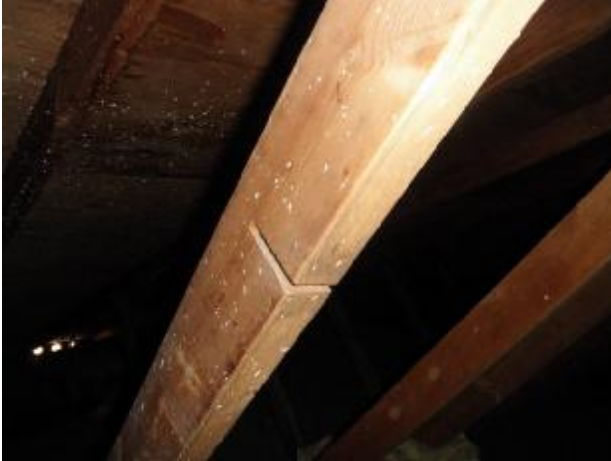
Truss cord cut through in the attic space.
