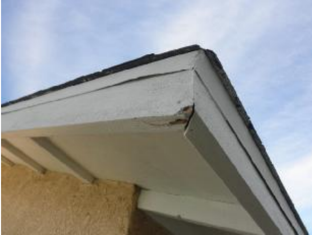
Moisture damage at the fascia boards.
