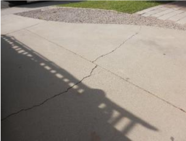
General settlement cracks in the concrete driveway.
