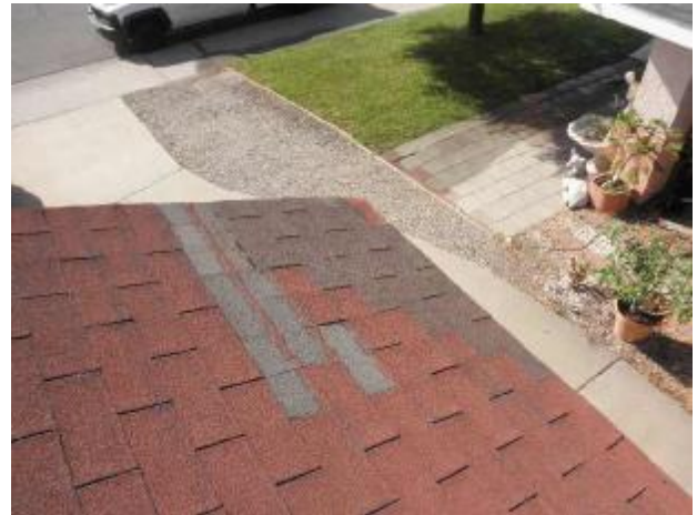
Example of the general deterioration and damaged roof shingles.
