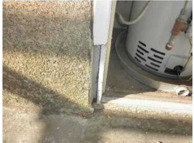
Part of the trim is missing at the water heater closet door.
