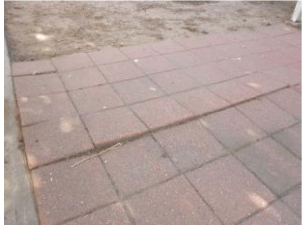
Tripping hazard at the uplifted paver patio.
