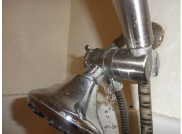
Connection at the shower head leaks.
