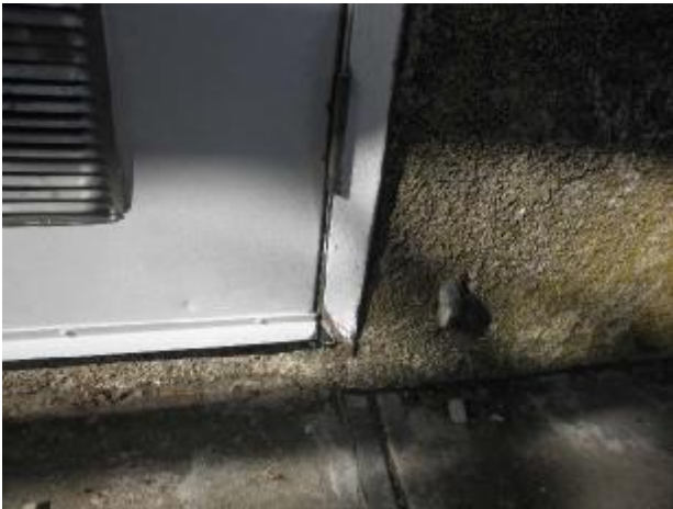
Moisture damage to part of the exterior trim at the water heater closet door.
