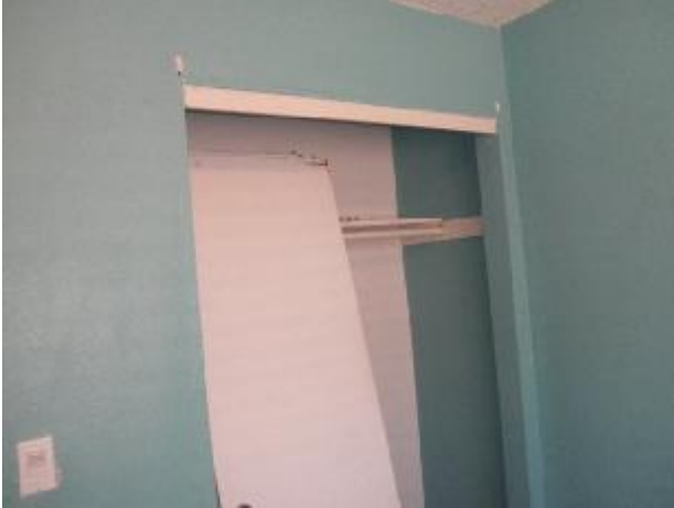
Closet door off the tracks in the west bedroom.
