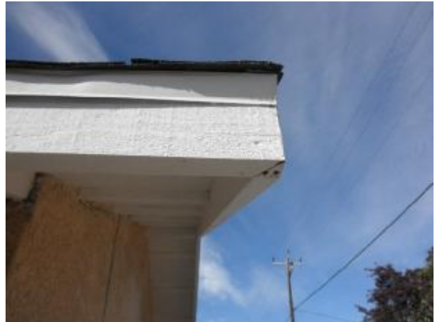
Moisture damage at the fascia boards.
