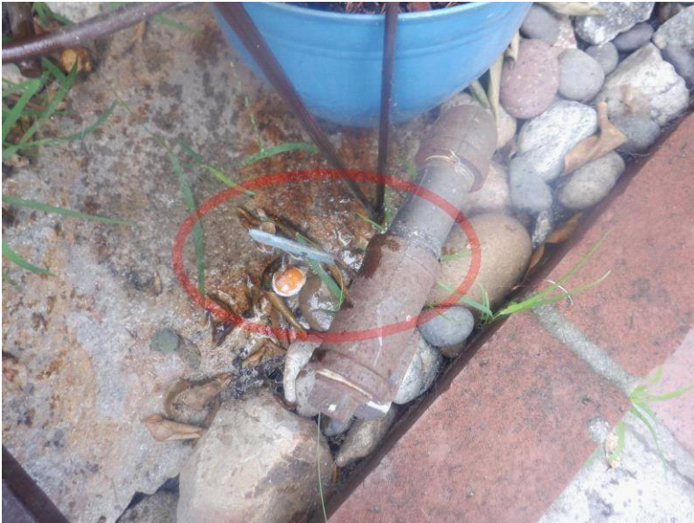
Fire pit gas valve
