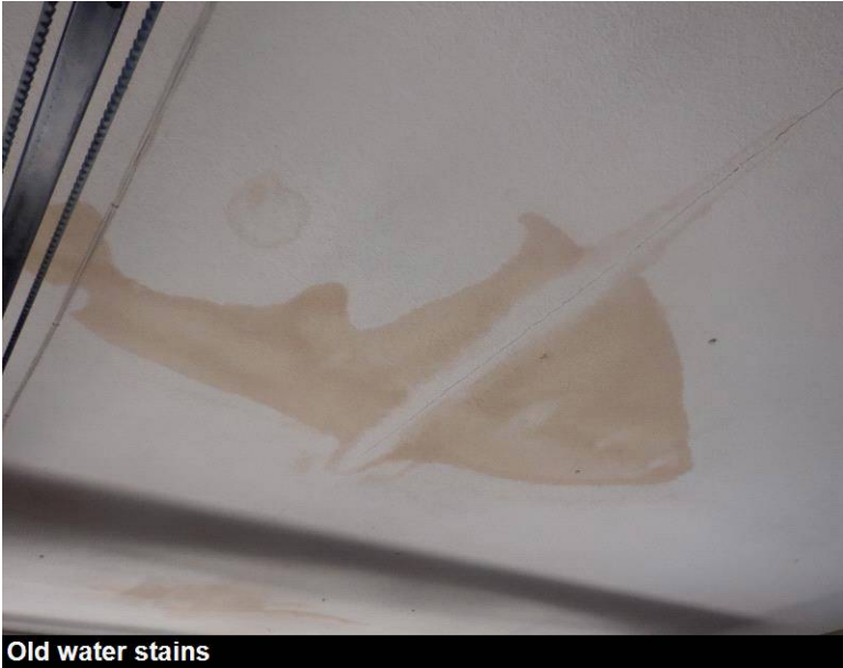
Old water stains
