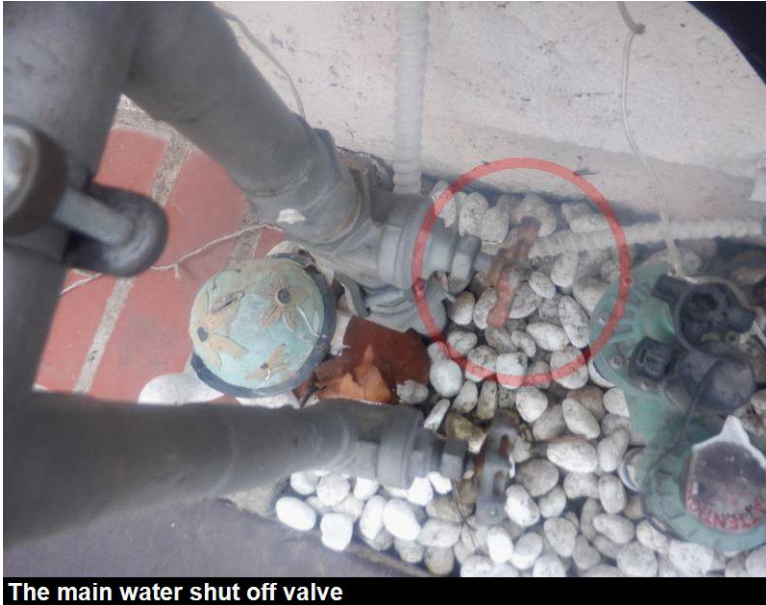
The main water shut off valve
