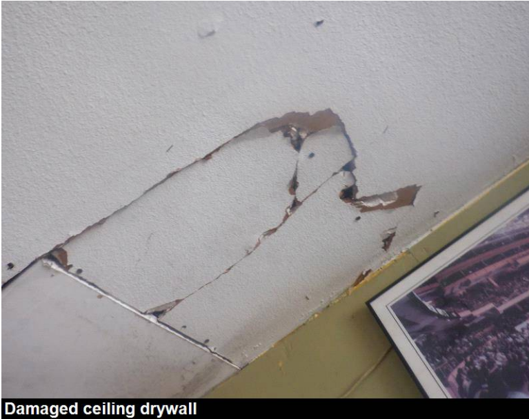
Damaged ceiling drywall
