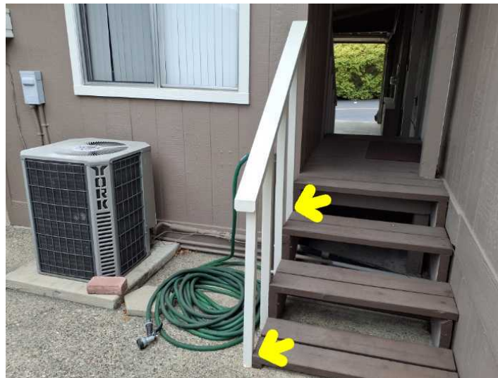
One or more handrails are not secure and should be serviced for optimal safety.
