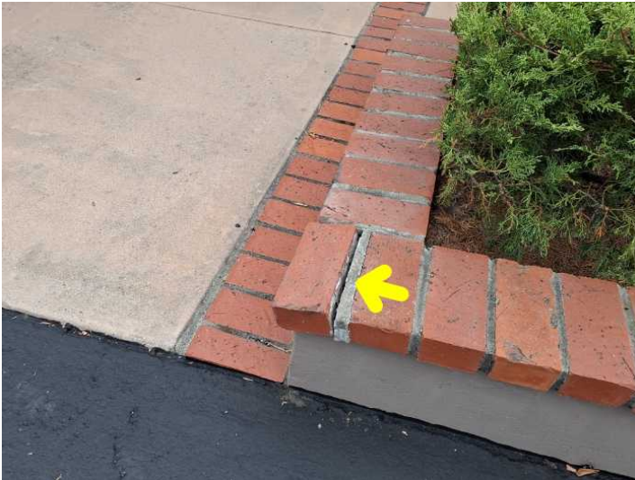
One or more yard wall caps are loose or missing and should be serviced.
