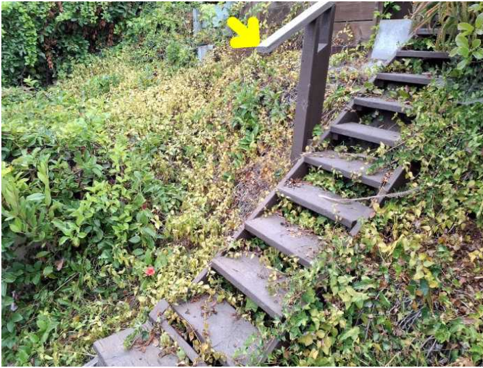
The handrail does not fully extend to the bottom of the rear stairs, which should be serviced for optimal safety.
