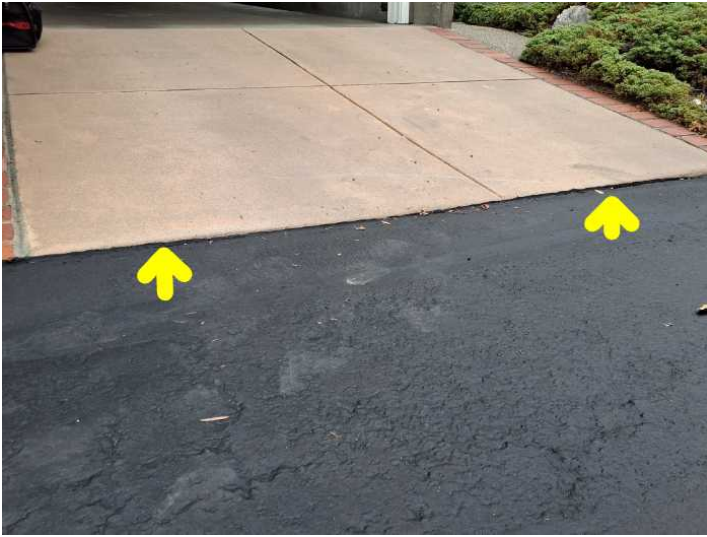
There are one or more offsets in the driveway that could prove to be trip-hazards.
