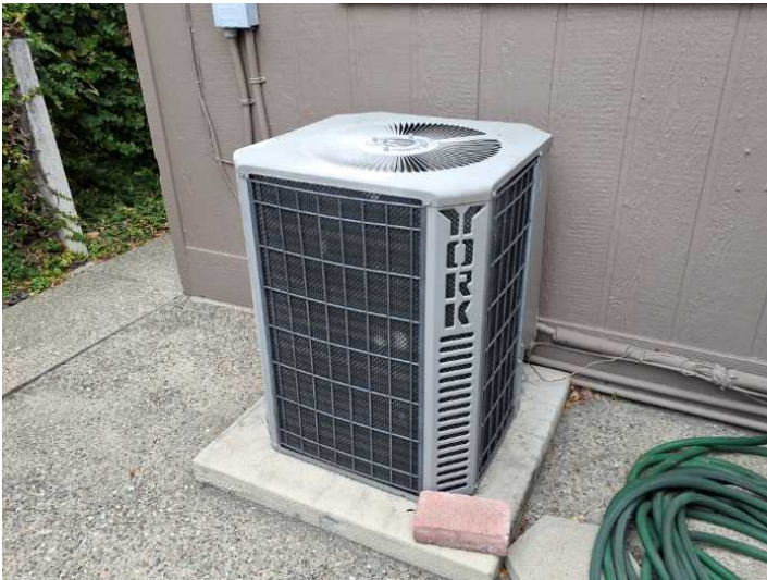
Central heat and air-conditioning are provided by a single split-system, consisting of a furnace with an evaporator coil that is located in the attic and a condensing coil that is located on the exterior.
