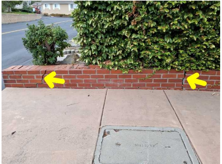
There are typical stress fractures or grout joint separations in the brick yard walls, but they are reasonably firm and do not appear to be in danger of falling at this time.
