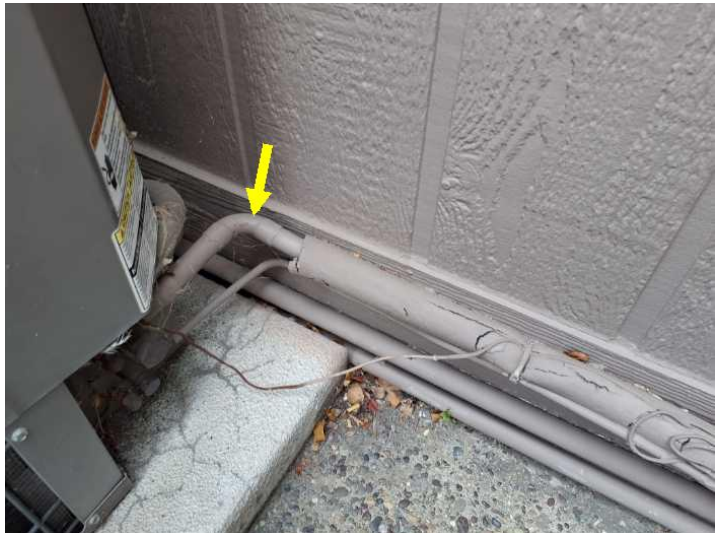
Insulation is missing from the refrigerant lines at the evaporator coil, which will allow condensation to form and drip, and should be installed.
