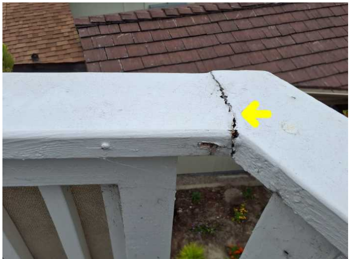
There is damage to one or more guardrails that should be evaluated by a pest inspector.
