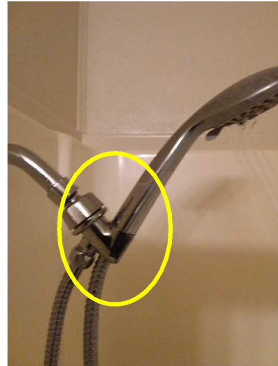
The showerhead leaks and should be serviced/repaired, which may be as simple as tightening it.
