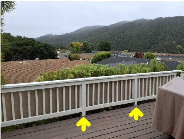
One or more guardrails are not secure, and should be serviced by a qualified specialist.
