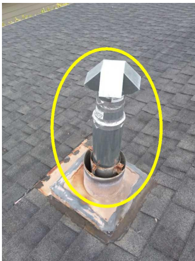
The vent cap on the roof may not be an approved type and should be evaluated and serviced as needed.
