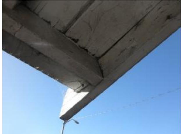
Moisture damage at the SW eave.
