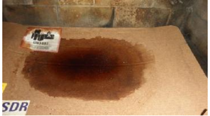
Water leak inside the fireplace.
