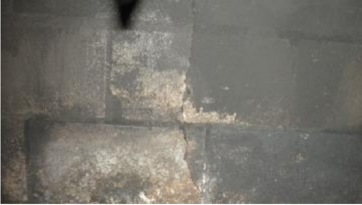
Cracks in the firebox.
