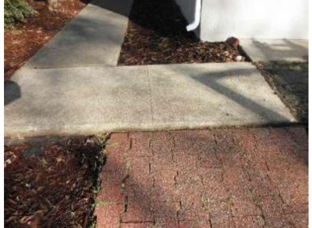
Tripping hazard at the front walkway.
