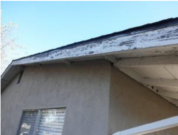
The eaves need to be painted.
