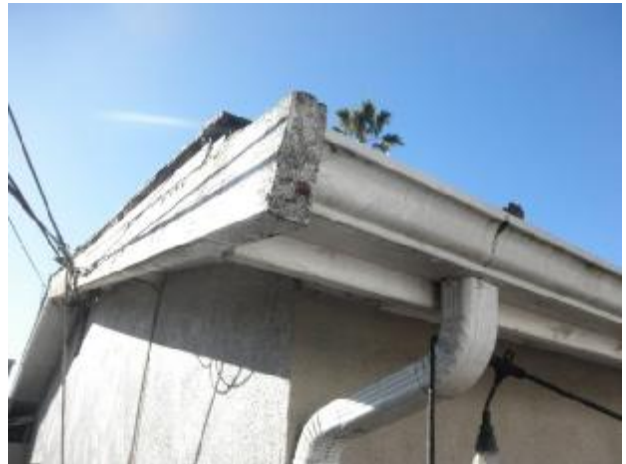
Moisture damage at the NE fascia.
