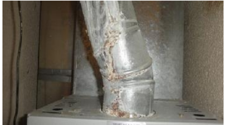
Evidence of leak at the furnace flashing.
