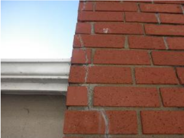
Thermal cracking on the outside brick wall of the chimney.
