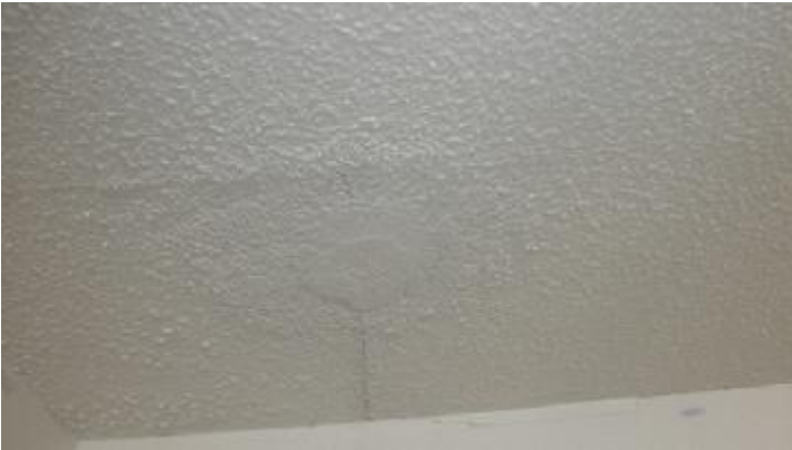
Example of patches at the living room ceiling.
