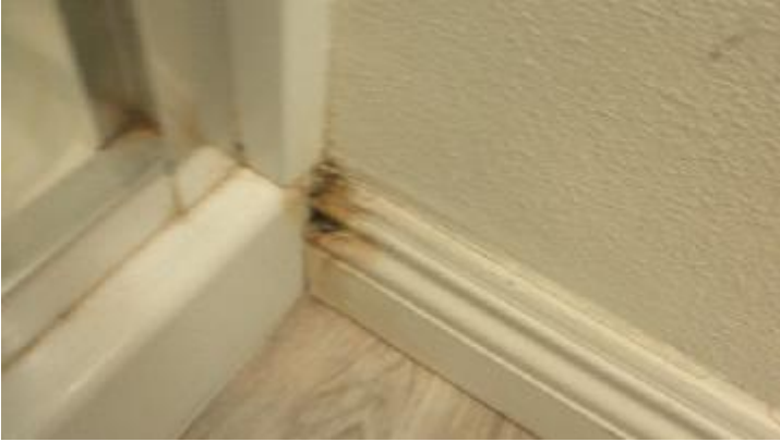
Moisture damage and black mildew like substance at the edge of the master shower.
