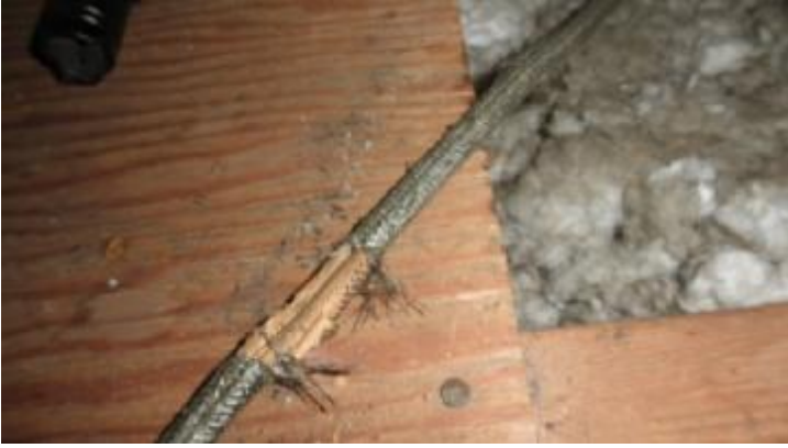
Frayed electrical romex wiring in the attic.
