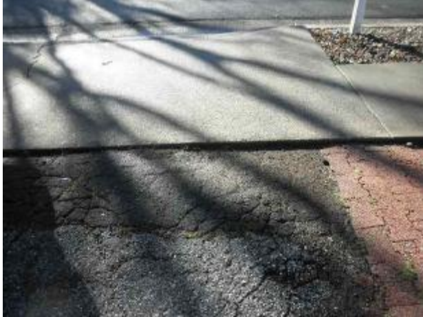
Tripping hazard at the driveway and sidewalk.
