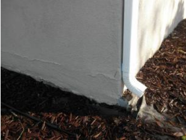
Settlement crack with patching at the SW corner.
