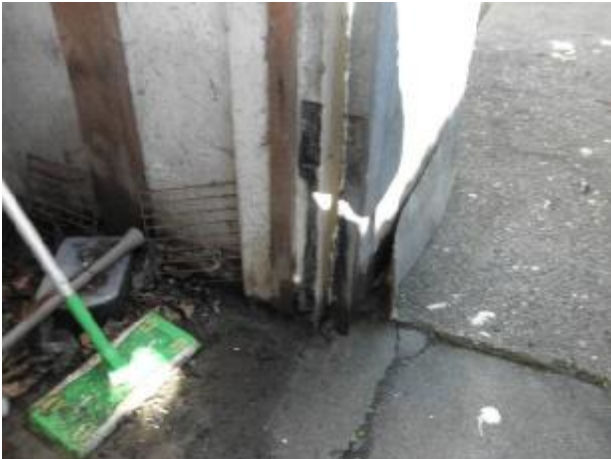
Moisture damage at the water heater closet door.
