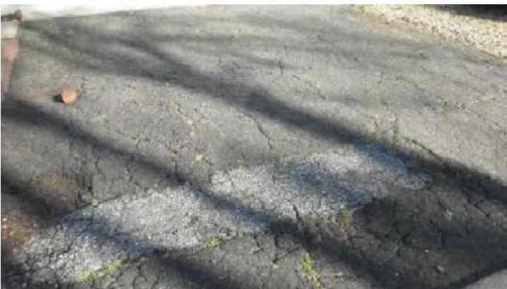
The asphalt driveway needs to be resealed.
