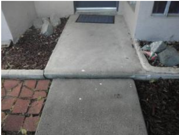
Tripping hazard at the front walkway.
