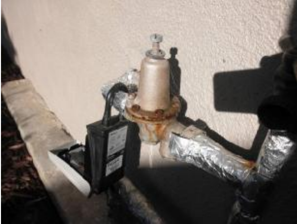
Leak at the pressure regulator at the main water shut off.
