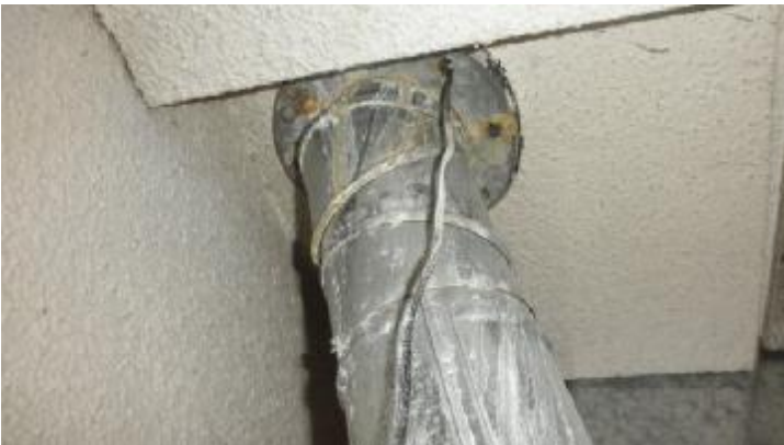
Evidence of leak at the furnace flashing.
