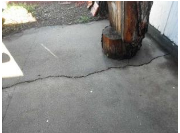
General settlement crack in the concrete driveway at the NW corner of the property.
