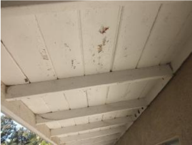
The eaves need to be painted.
