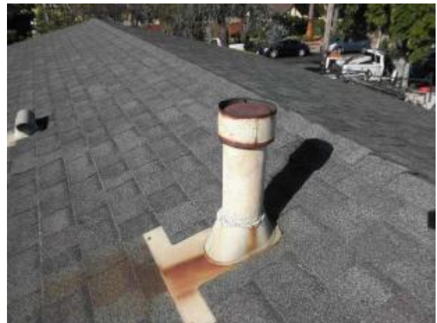
Missing storm collar the furnace exhaust.
