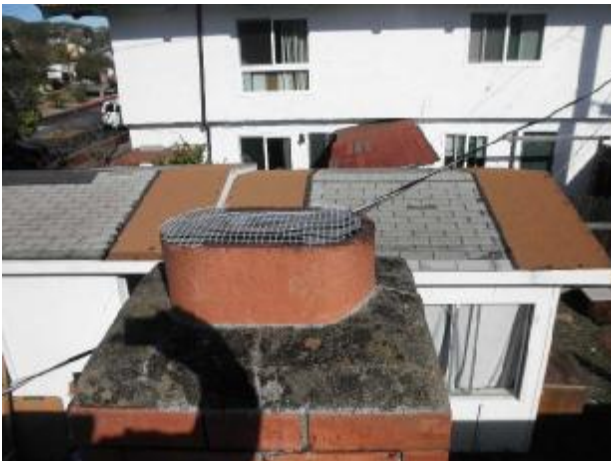
Substandard spark arrester at the chimney.
