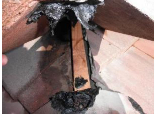
No water proof fabric below the hip and ridge roof tiles.
