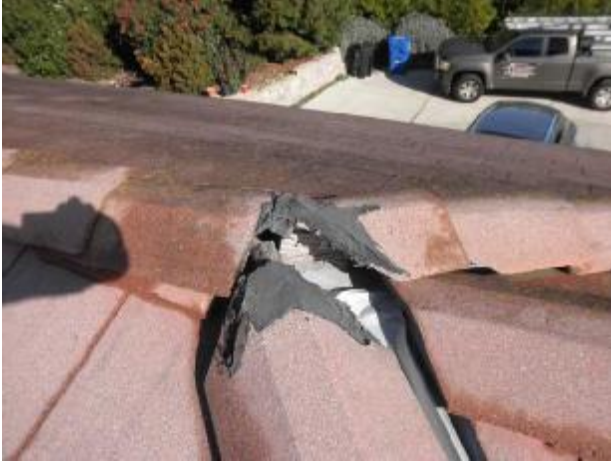
Deteriorated sealant at the top of the hip above the garage.
