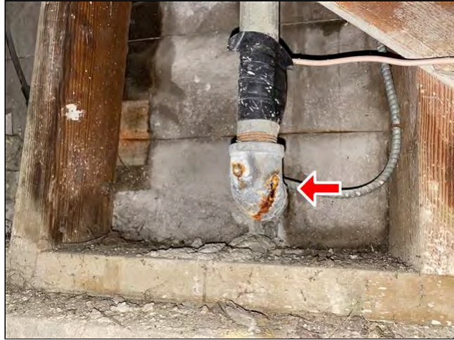
Item 28 - Item 2(Picture) Plumbing System
