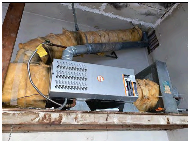
4.0 Item 1(Picture) Heating/Central Air
