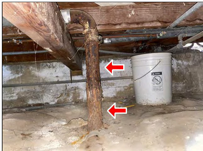
5.0 Item 1(Picture) Plumbing System
