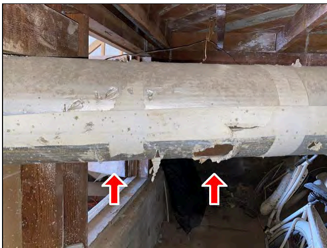
4.5 Item 1(Picture) Heating/Central Air
