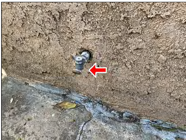
5.1 Item 6(Picture) Plumbing System
