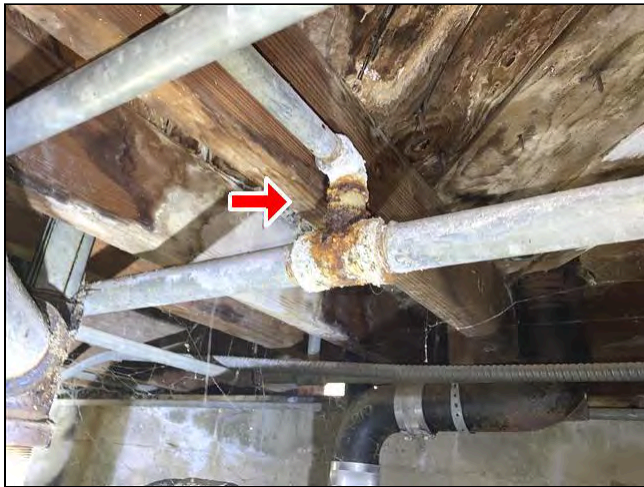
5.1 Item 3(Picture) Plumbing System
