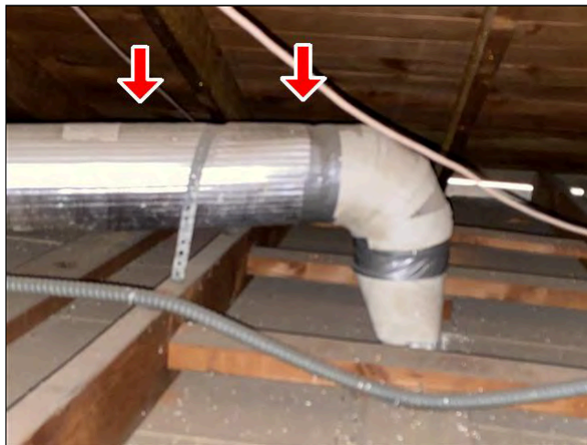
4.5 Item 4(Picture) Heating/Central Air
