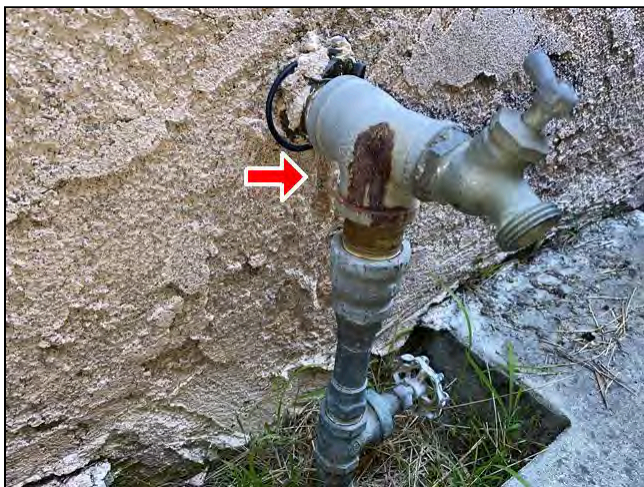
5.1 Item 1(Picture) Plumbing System
