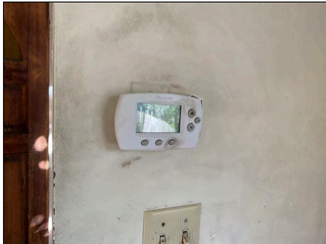
4.2 Item 1(Picture) Heating/Central Air
