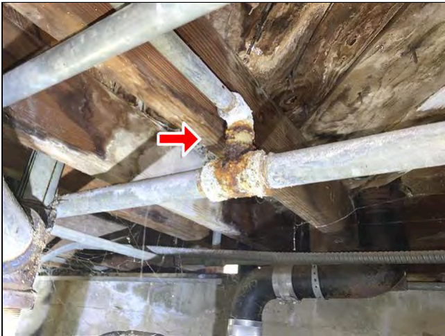
Item 28 - Item 3(Picture) Plumbing System
