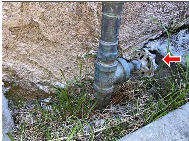
5.1 Item 7(Picture) Plumbing System
