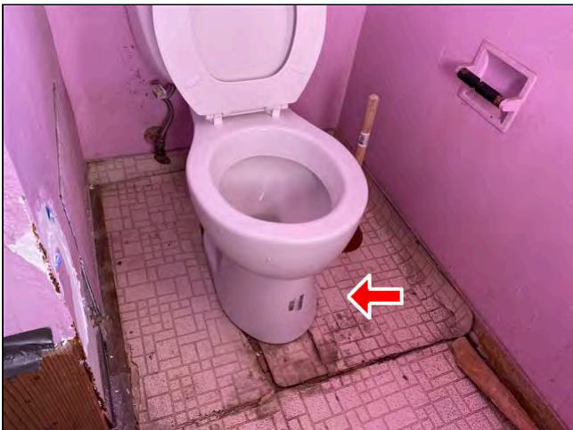
Item 31 - Item 1(Picture) Plumbing System
