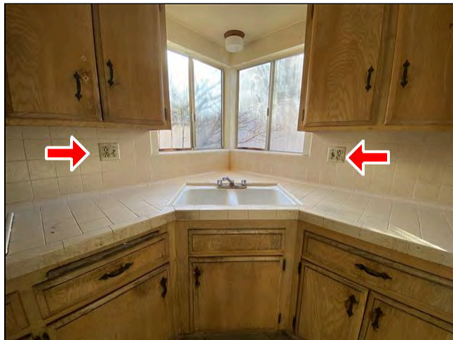
6.2 Item 1(Picture) Electrical System
