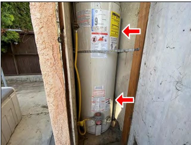
Item 33 - Item 1(Picture) Plumbing System
