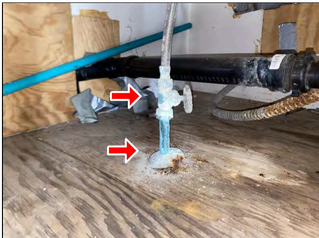
5.1 Item 5(Picture) Plumbing System
