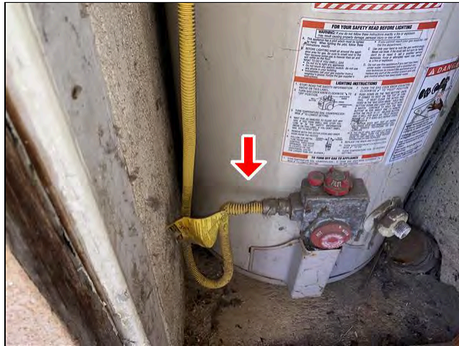
5.4 Item 1(Picture) Plumbing System
