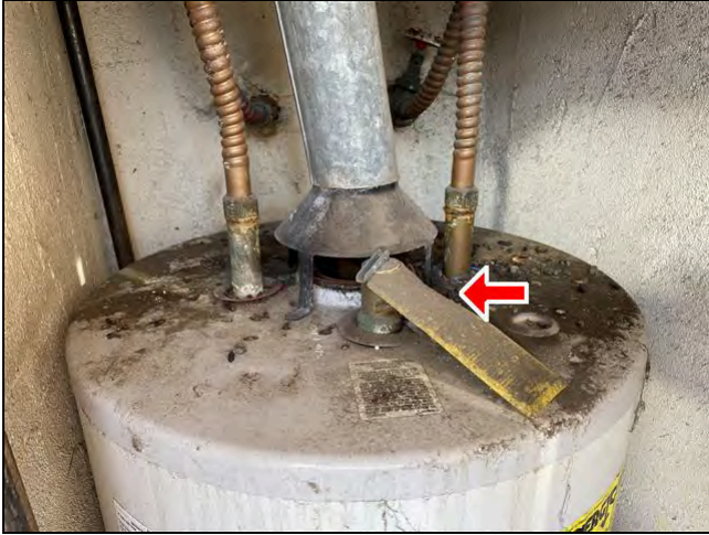
Item 32 - Item 1(Picture) Plumbing System
