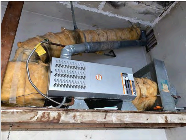
Item 21 - Item 1(Picture) Heating/Central Air Flues and Vents (for gas heating systems)
