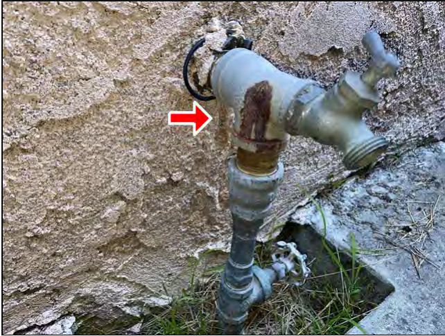
Item 28 - Item 1(Picture) Plumbing System
