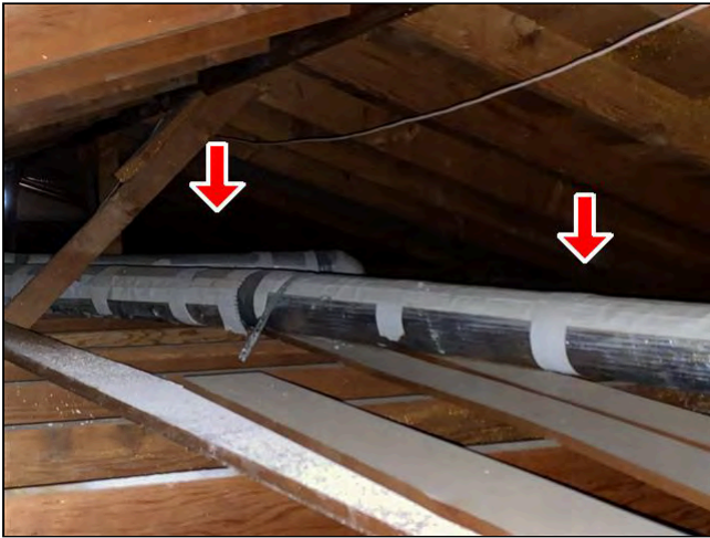
Item 24 - Item 3(Picture) Heating/Central Air Plumbing Drain, Waste and Vent Systems
