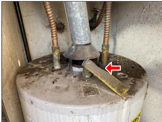
5.2 Item 1(Picture) Plumbing System
