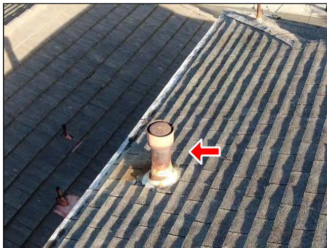
4.3 Item 1(Picture) Heating/Central Air
