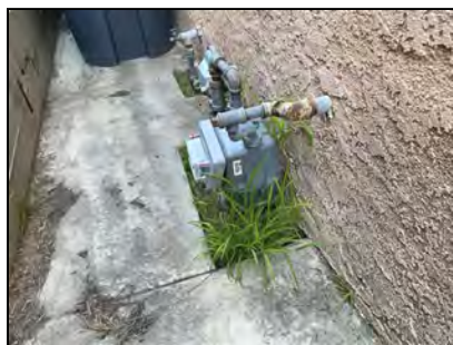
5.5 Item 1(Picture) Plumbing System
