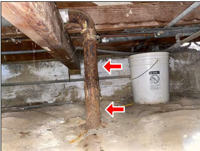
Item 25 - Item 1(Picture) Plumbing System
