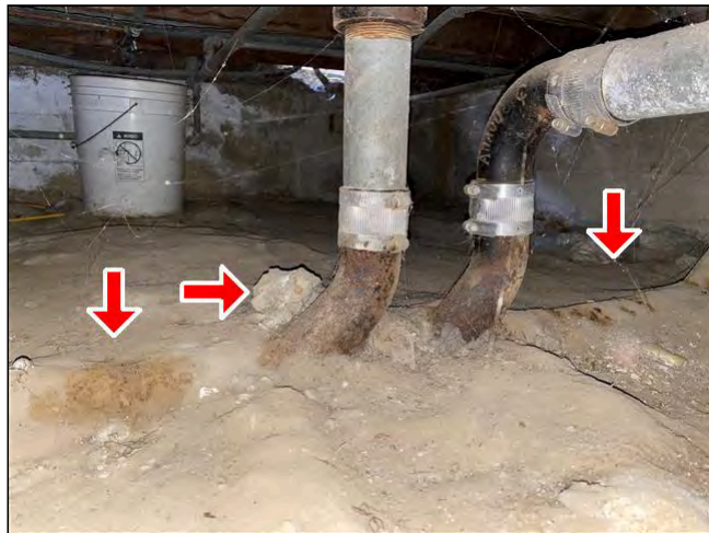
Item 25 - Item 2(Picture) Plumbing System
