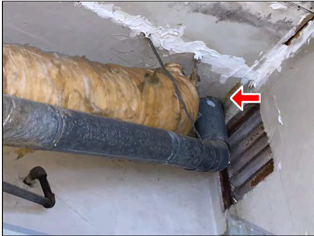
4.3 Item 2(Picture) Heating/Central Air
