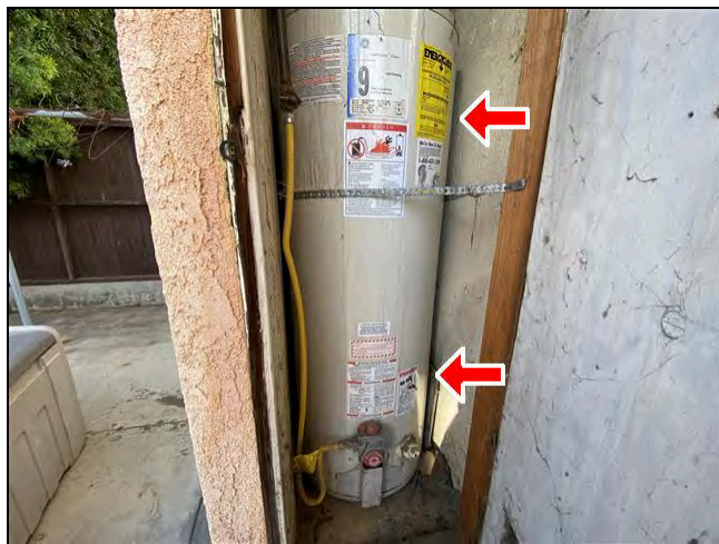
5.2 Item 2(Picture) Plumbing System
