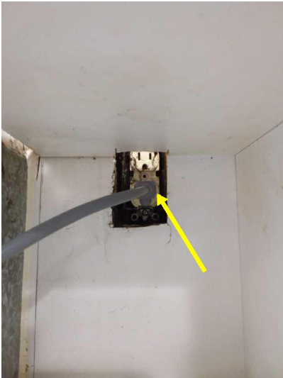
One or more outlet covers is missing or broken and should be serviced.
