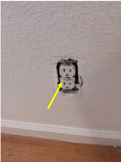
There are outlet or switch covers that are missing and should be replaced.
