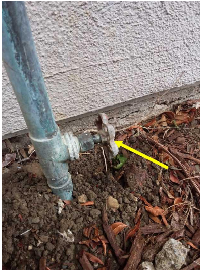
The main water valve is leaking and should be repaired.
