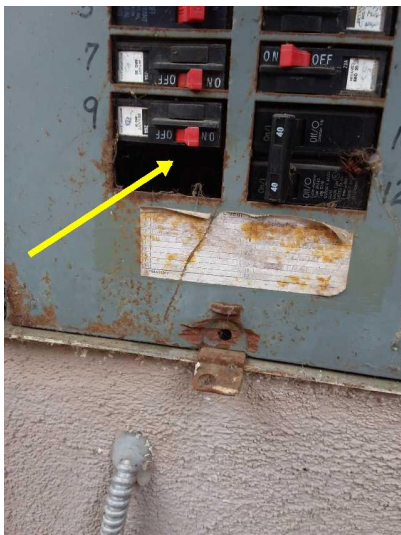
There are voids or open knockouts in the cover of the main electrical panel that should be covered.
