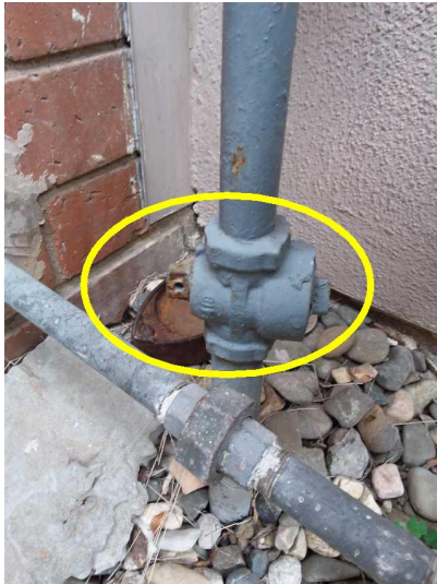
The gas main shut-off is located on left side of the home, unit or building.
