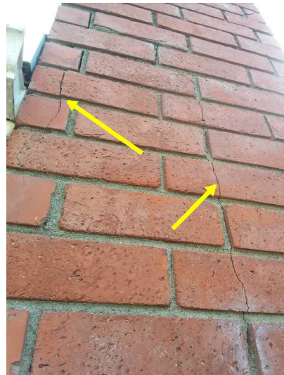
The chimney wall is cracked and should be evaluated by a specialist.
