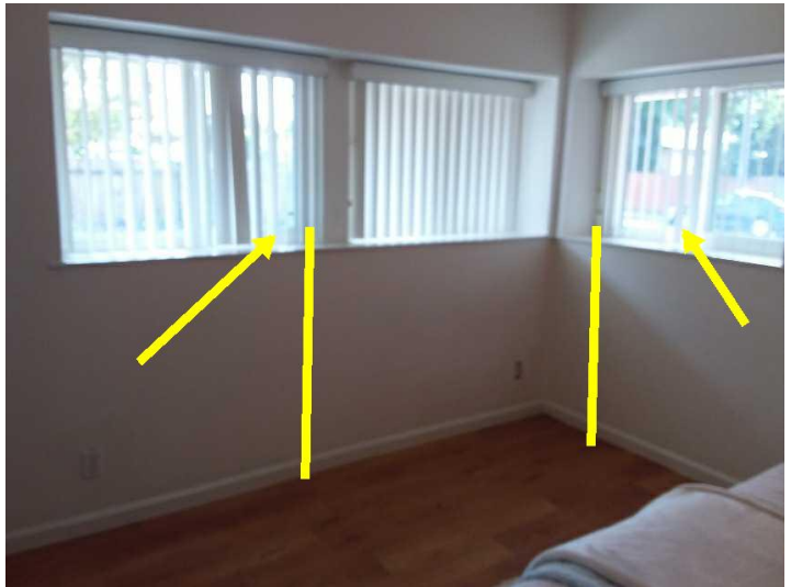
A window is too high or too small to facilitate an emergency exit or egress. Bedroom windows should measure 24" high by 20" wide, with an optimum sill height of 44", to facilitate an emergency exit by the occupant and an emergency egress for a fire person wearing breathing apparatus.
