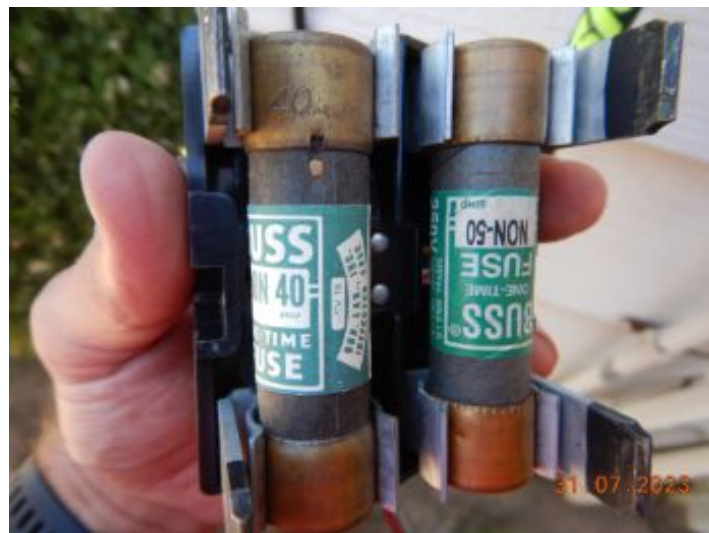
Fuses in for main fuse block
