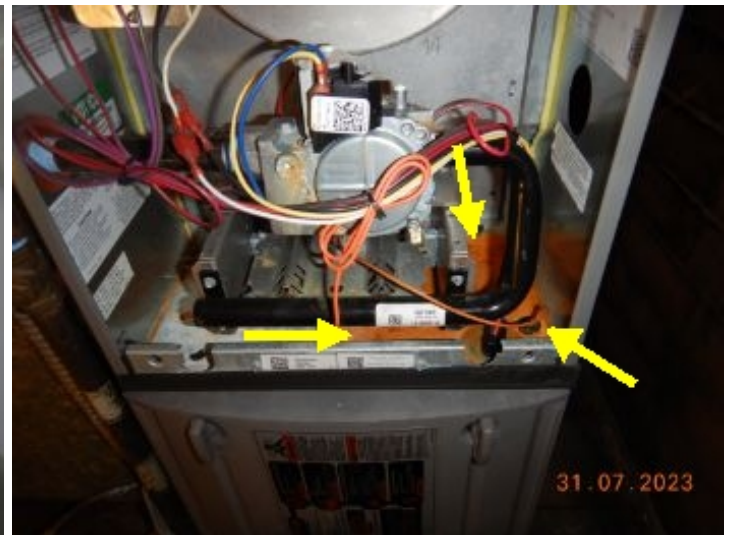
Rust in heater compartment
