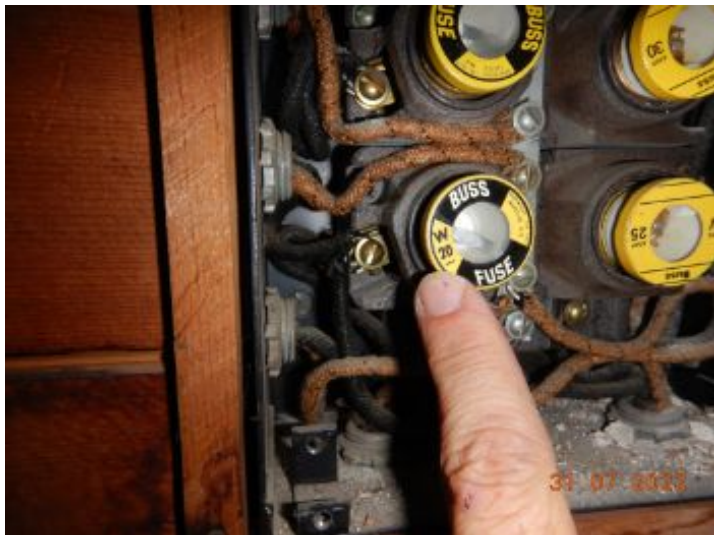
Example of double tapping and aluminum wiring
