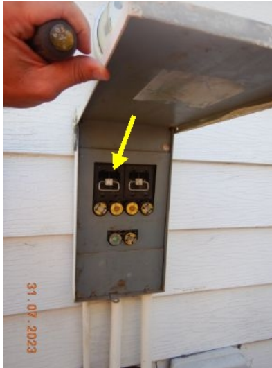
Main fuse block
