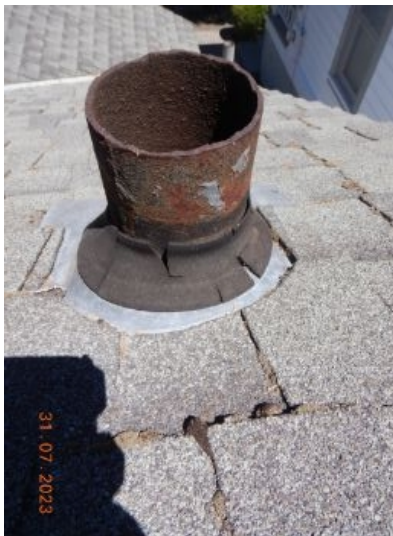
Example of failed seal
