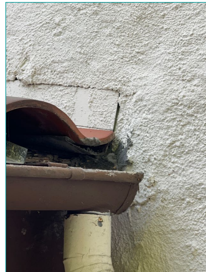
Missing kick-out flashing
