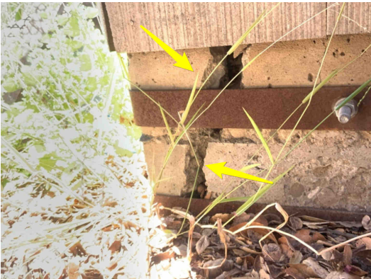
cracks and displacement at foundation stem wall
