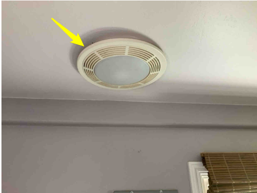
Fan cover found loose ceiling. Maintenance or upgrade recommended
