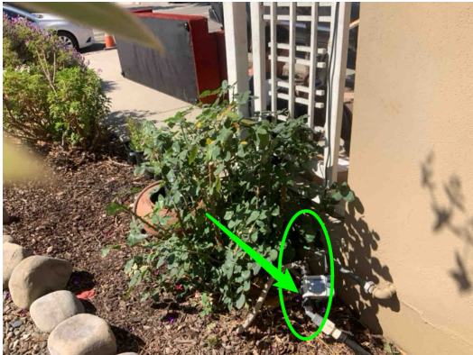
Main water shut off valve
