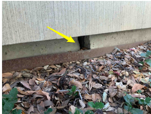
cracks and displacement at foundation stem wall
