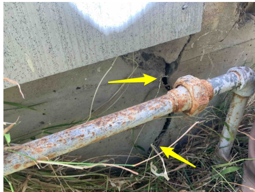
Some moderate cracks not repaired
