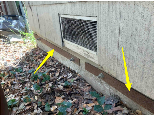
Past repair straps
