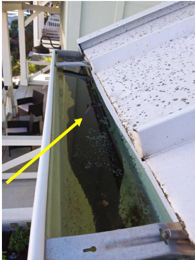
We observed standing water in some sections of the gutters which implies that it may not be properly sloped and should be evaluated and serviced.
