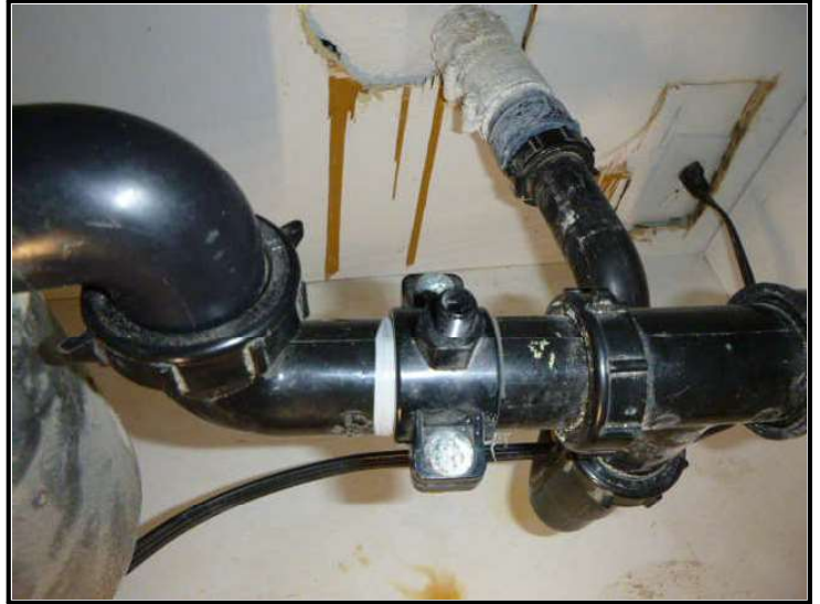
View of uncapped opening at drain.
