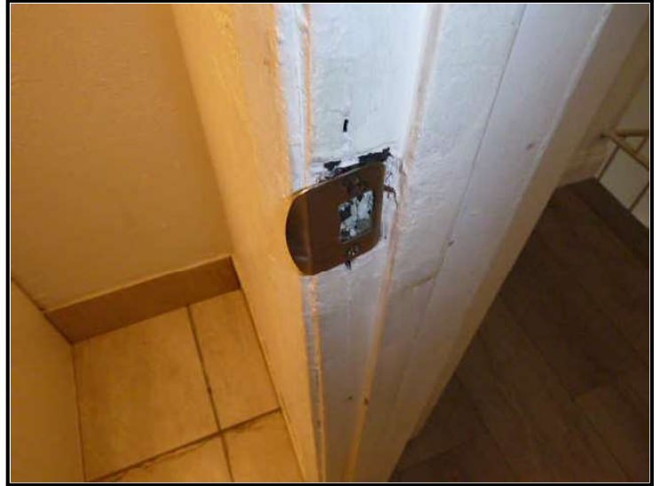
View of cracks/damaged door jamb in bathroom #2.
