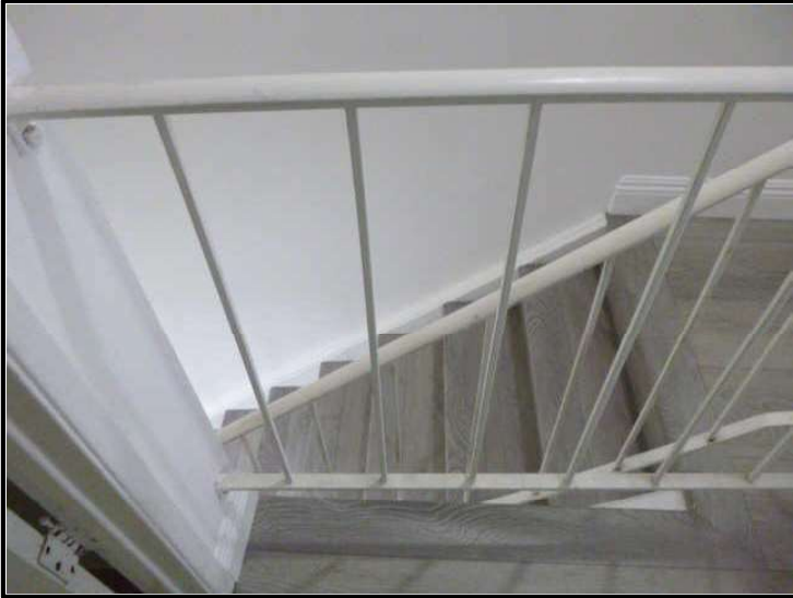
View of baluster spacing excessive.
