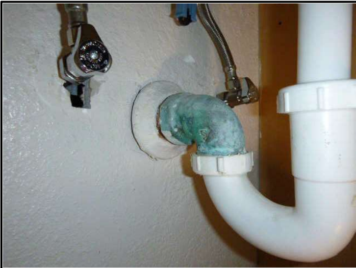
View of corrosion/rust at drain in bathroom #1.
