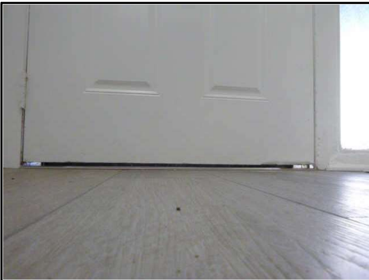
View of gaps at bottom of door in entry hall.
