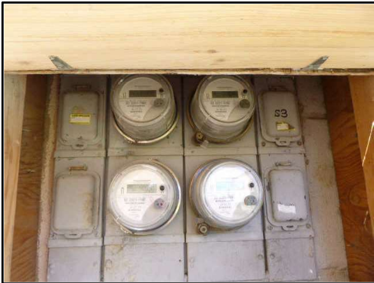
View of electric meter.
