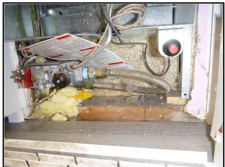
View of older gas line/no sediment trap.
