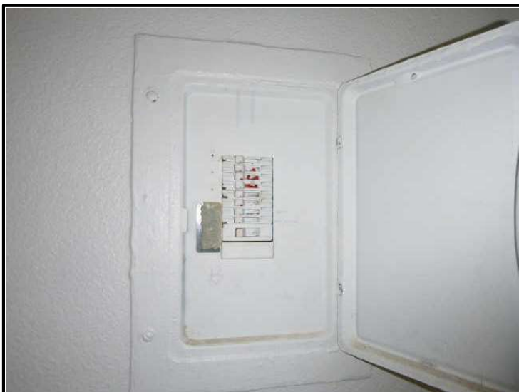
View of sub panel.
