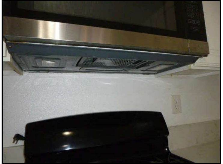
View of missing filter at stove hood.
