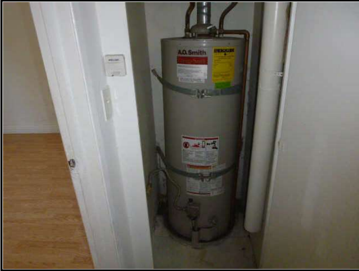
View of water heater not level.
