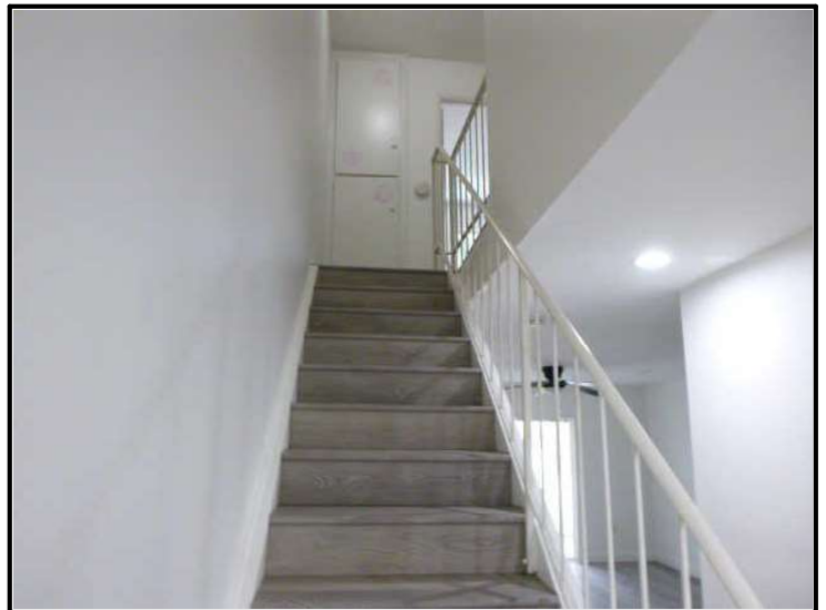
View of staircase, baluster spacing excessive.
