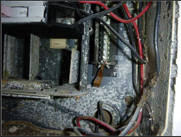
View of irregular installation at ground/neutral wiring at sub panel.
