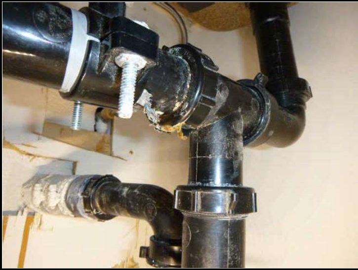
View of leaking/corrosion at drain.
