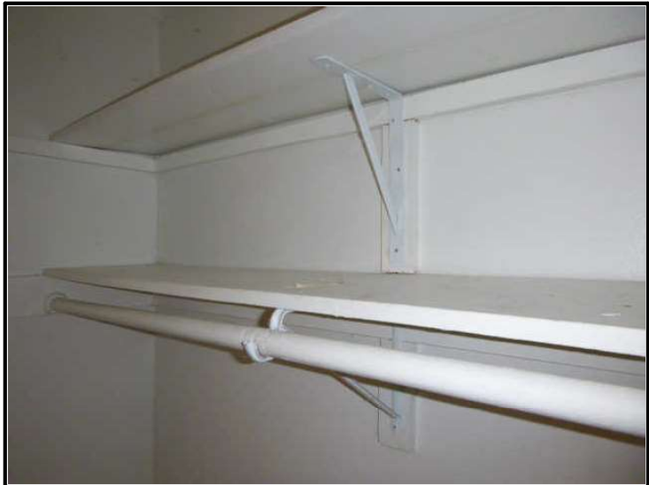
View of sagging shelf at closet in bedroom #2.
