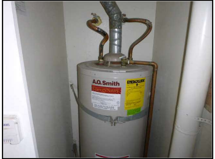
View of plumbing, rust noted.
