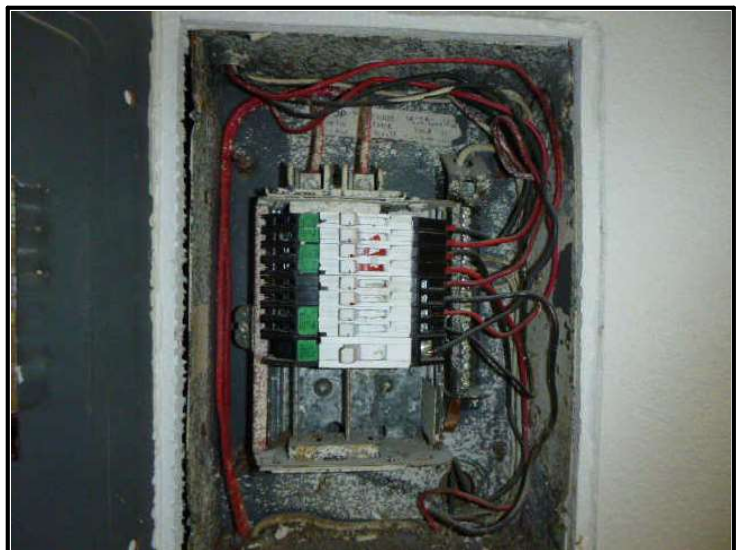
View of circuit breakers and wiring inside of sub panel.
