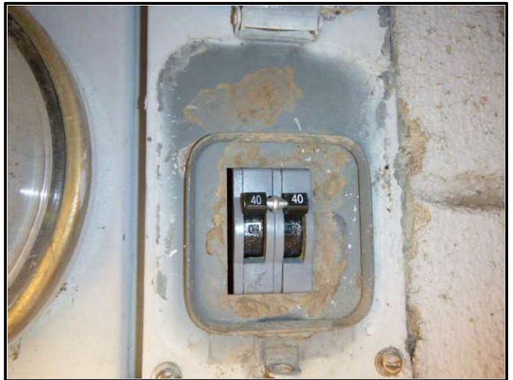
View of main breaker.
