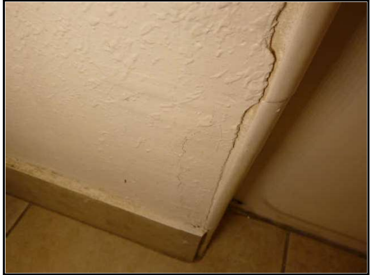
View of cracks, patching at wall in bathroom #2.
