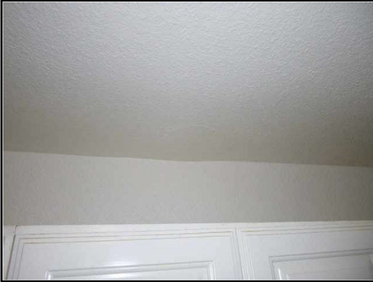
View of uneven area at ceiling.
