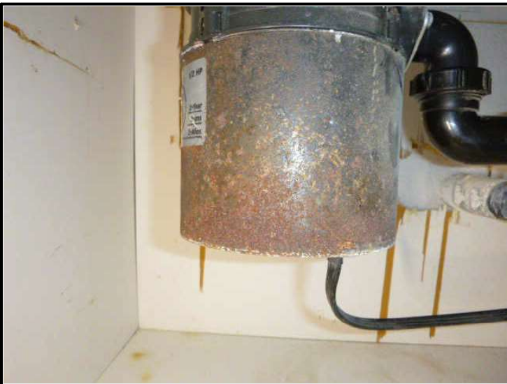
View of wear, heavy rust at garbage disposal casing.
