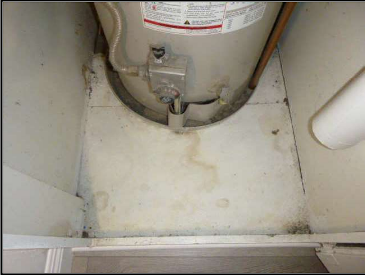
View of moisture stains/damage in enclosure.
