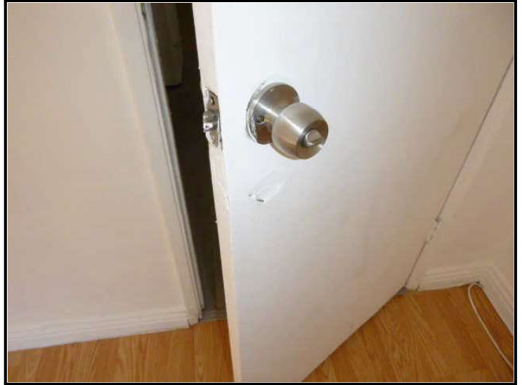
View of cracks, damage at door/jamb in bedroom #2.
