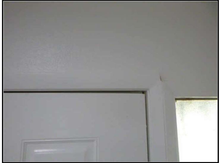
View of gaps at door, not square in jamb in entry hall.
