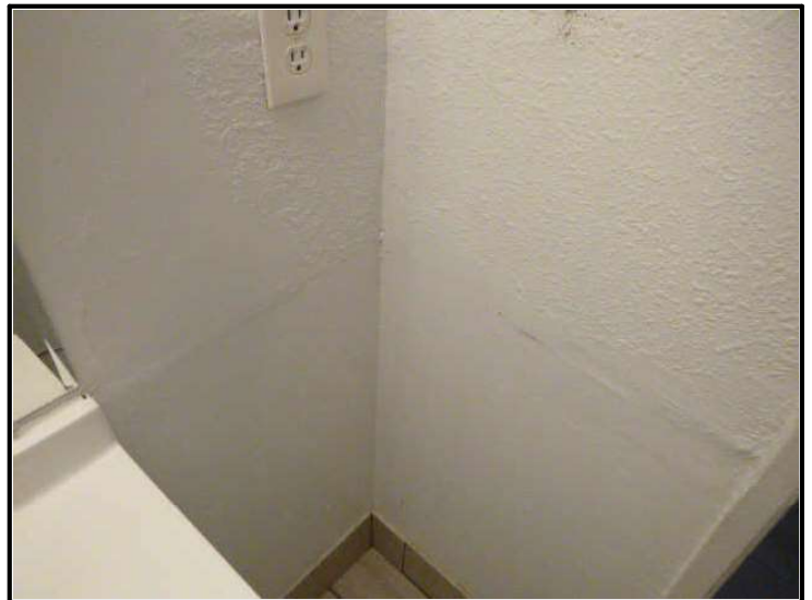
View of heavy patching at wall in bathroom #2.
