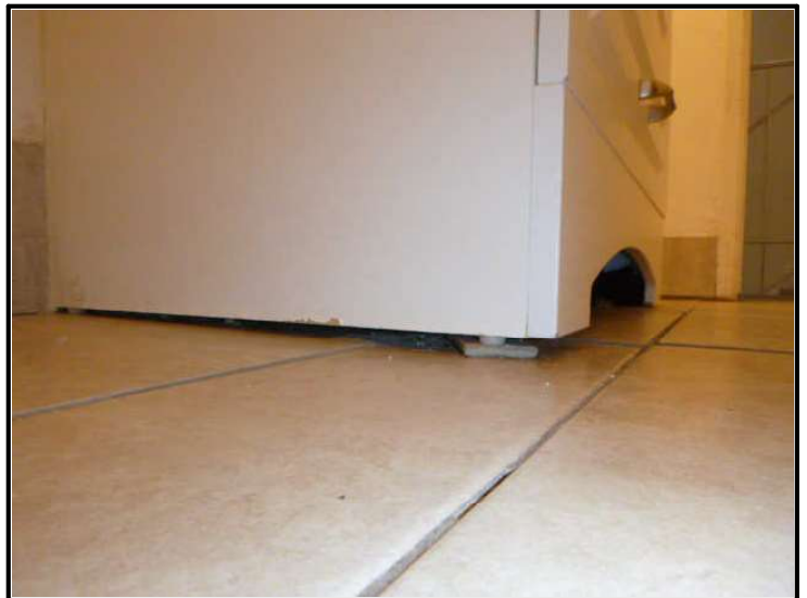
View of irregular installation at cabinet in bathroom #2.
