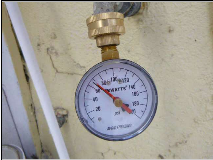
View of water test. Static 67 PSI.
