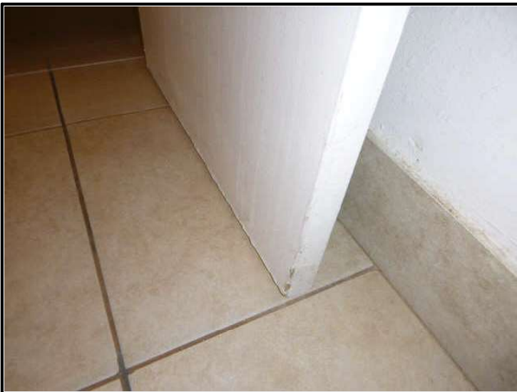
View of wear, blistered, moisture damage at door in bathroom #2.
