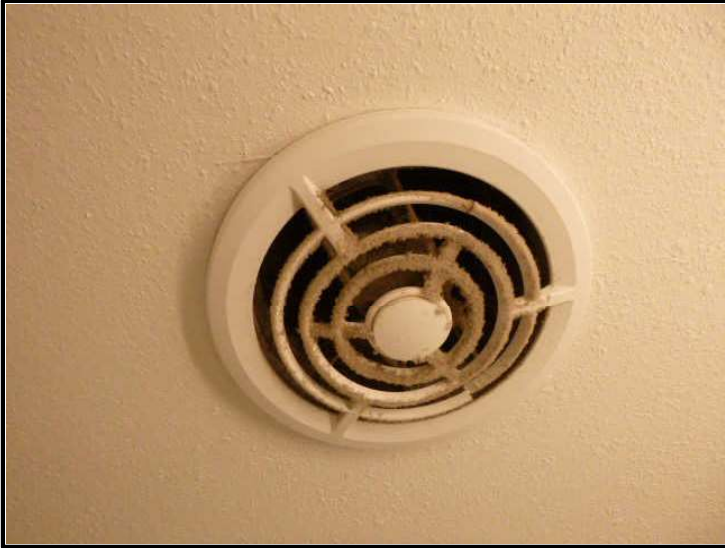
View of worn/dirty exhaust fan in bathroom #2.
