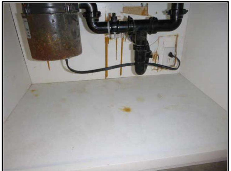
View of moisture damage at cabinet base.
