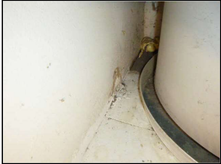
View of moisture stains/damage in enclosure.
