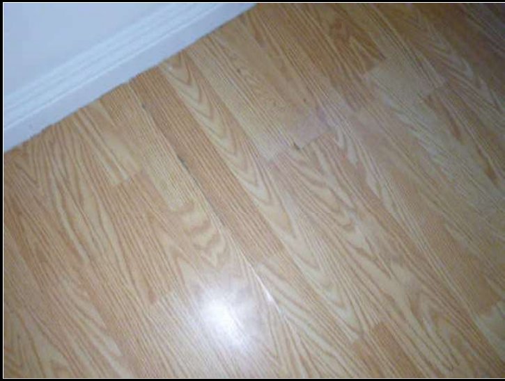
View of wear, chips, damage, moisture damage at floor in bedroom #1.
