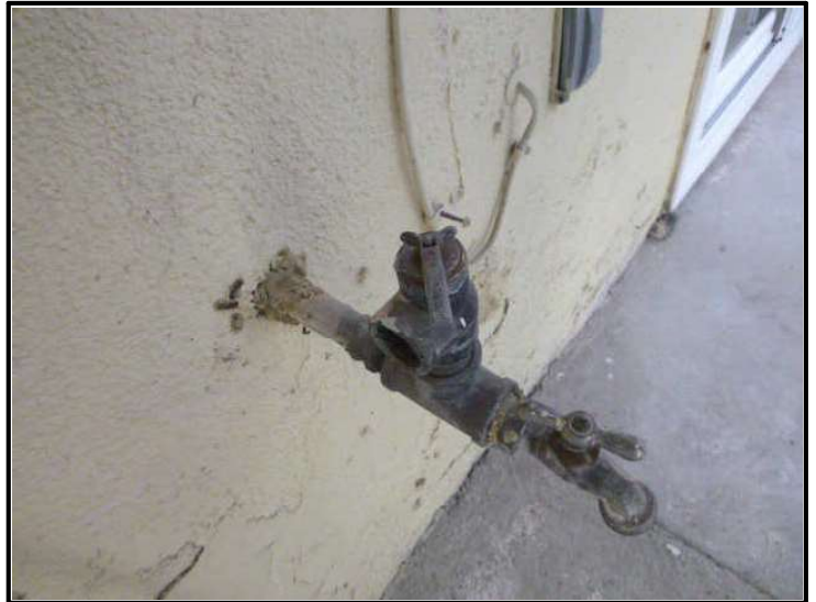
View of water service.
