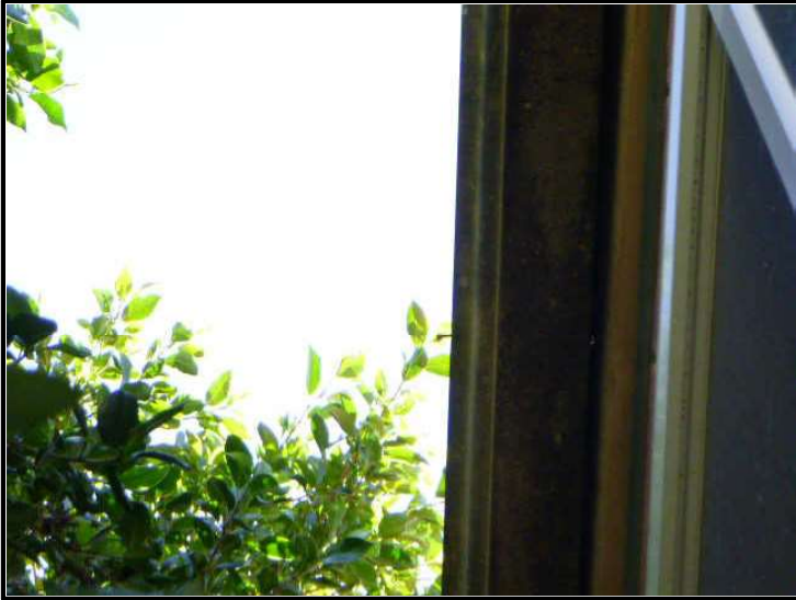
View of loose nail at gutters.
