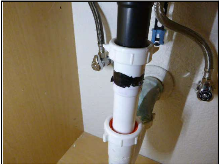
View of irregular glue on pipe, possible damaged pipe in bathroom #1.
