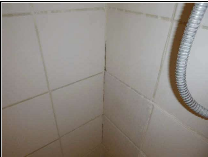
View of worn, mold like substance at shower enclosure in bathroom #2.
