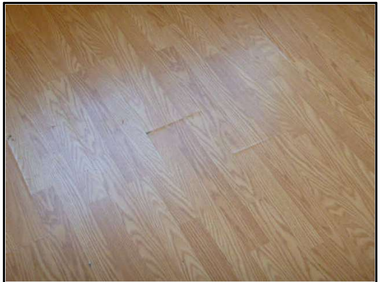
View of wear, chips, damage, moisture damage, uneven areas, loose material at floor in bedroom #2.
