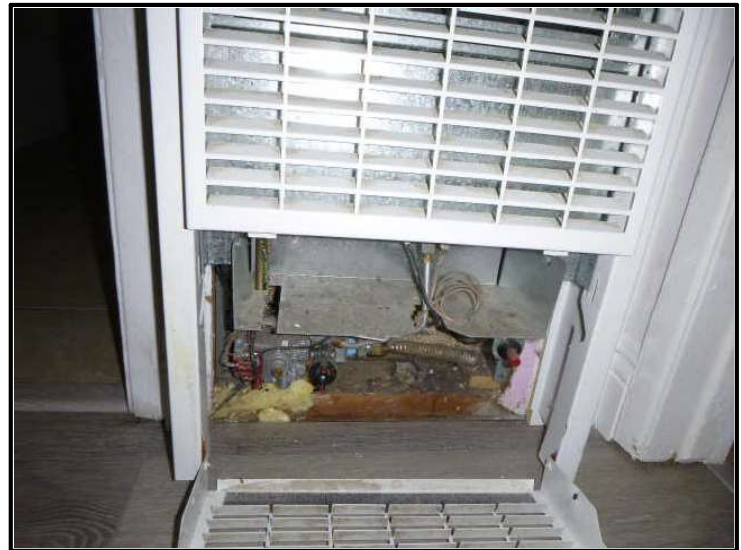
View of heater wall unit components. Pilot not lit.
