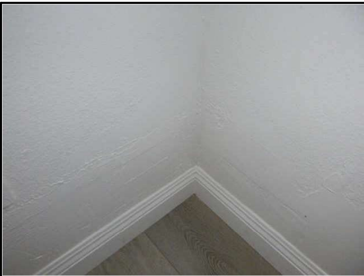
View of heavy/irregular patching at wall in living room.
