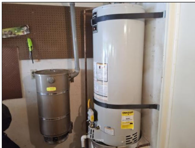
General View of the 50 Gallon Water Heater
