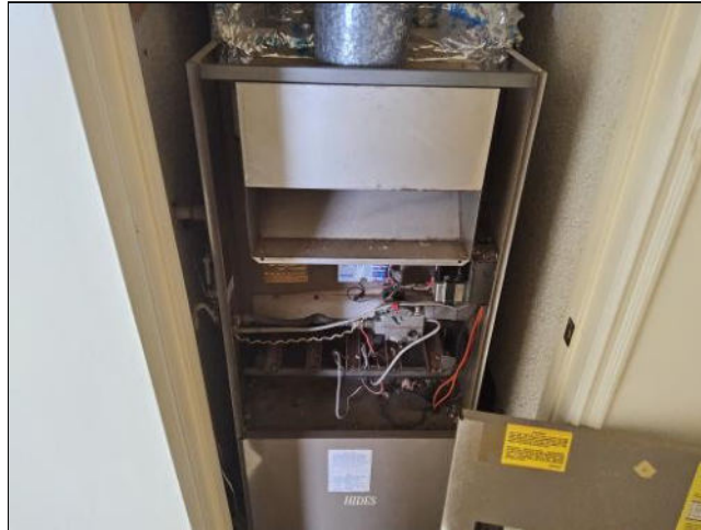
General View of the Heating System
