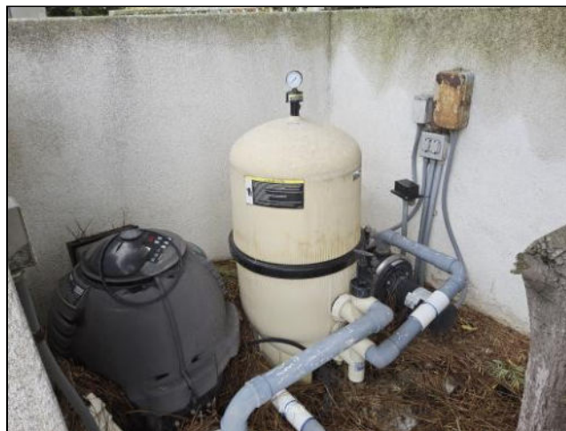
General View of the Pool Equipment Area
