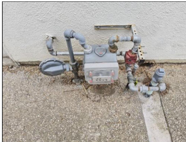
General View of The Gas Meter with Installed Seismic Gas Shutoff Valve
