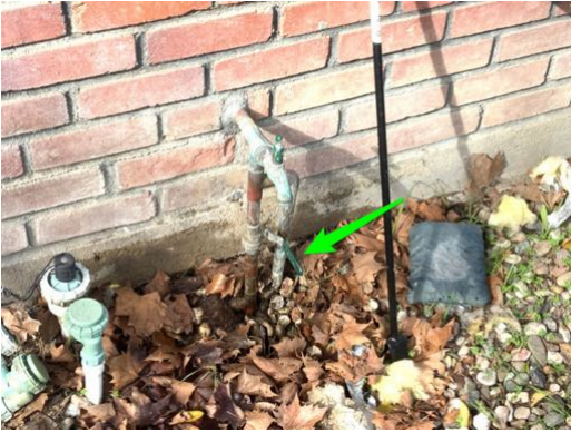
Main water shut off valve
