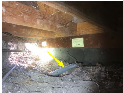
A Structural support post had fallen over
