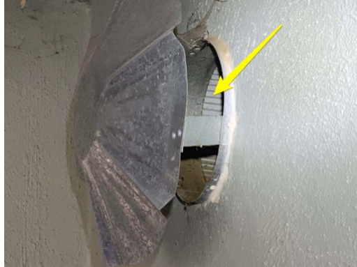
A proper screen cap is recommended to prevent critter intrusion
