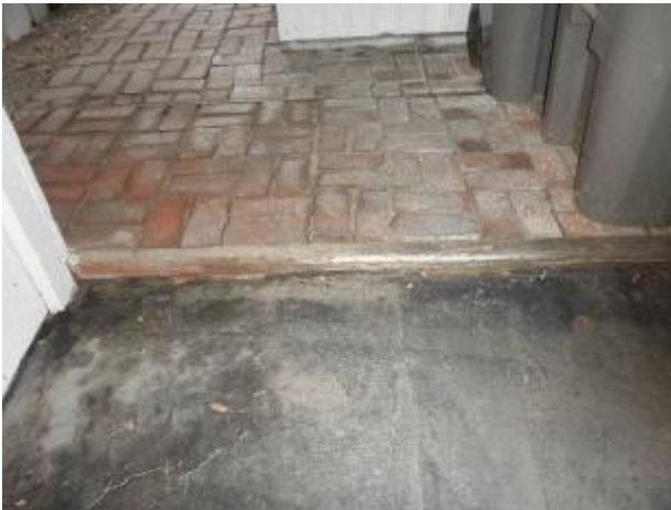
Tripping hazard at the interface of the carport asphalt and the brick walkway.
