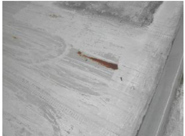
Example of rust damage to the metal roof.
