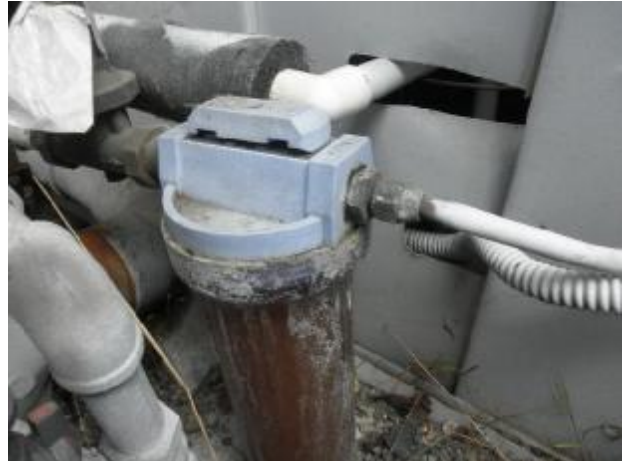
The cartridge filter needs to be replaced.
