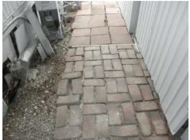
Dislodged bricks in the NW yard.
