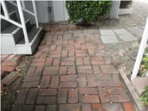
Dislodged bricks at the front entry walkway.
