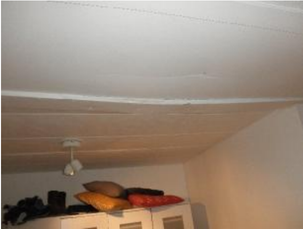
Ceiling sloped due to leak in the master bedroom.
