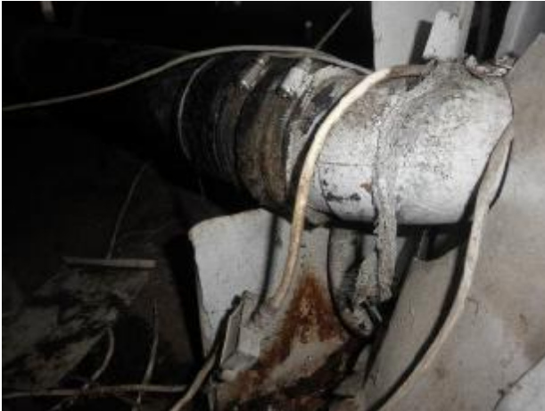
Leak at the 4" drain waster line.
