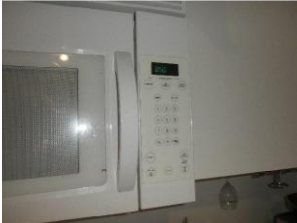
Control panel is loose at the microwave.
