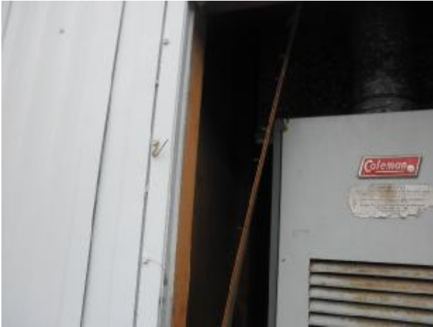
Loose wood paneling inside the furnace closet.
