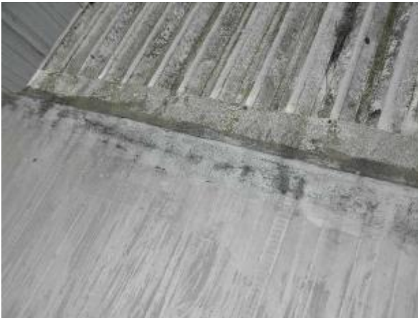
Deteriorated sealant at the perimeter.
