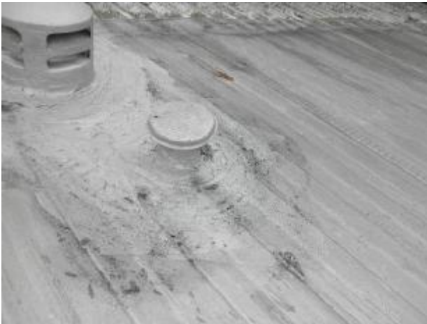
Waste vent pipes do not extend past the roof line.
