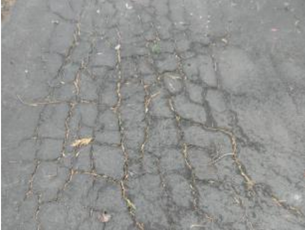
General cracking in the asphalt driveway.
