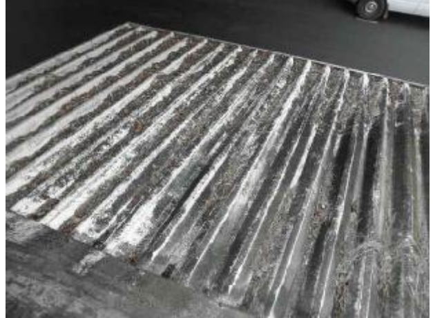
The patio roof is covered in debris.
