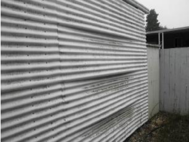
Parts of the Filon panels at the carport are warped.
