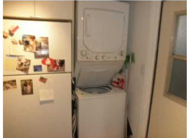
utility connection for the laundry units are blocked.
