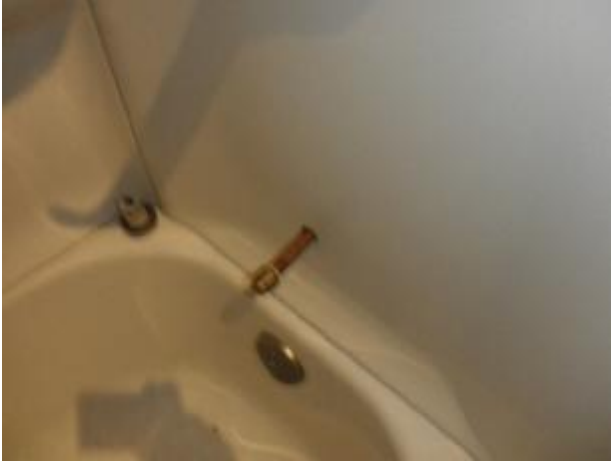
Tub spout missing in the bathroom.
