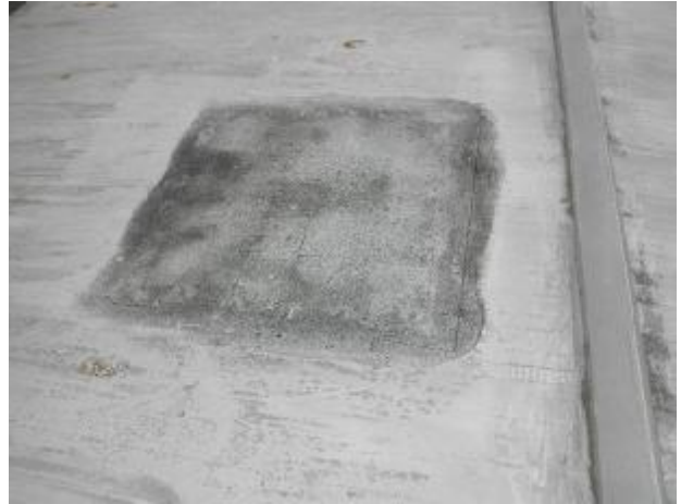
Large patch on the roof above the master bedroom.
