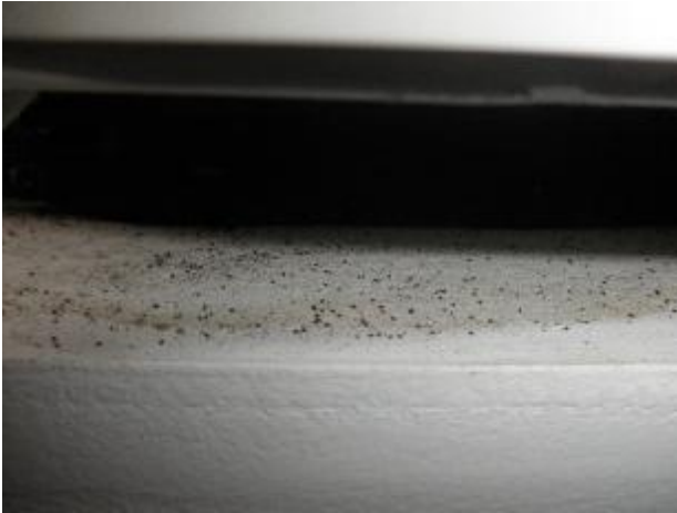
Possible termites at the window sill in the west bedroom.
