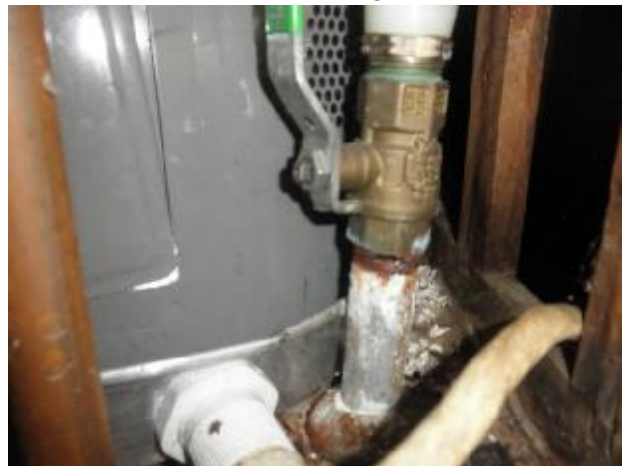
Leak at the cold water line connection to the water heater.
