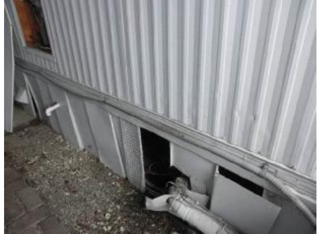
Example of the damaged skirting at the perimeter of the home.
