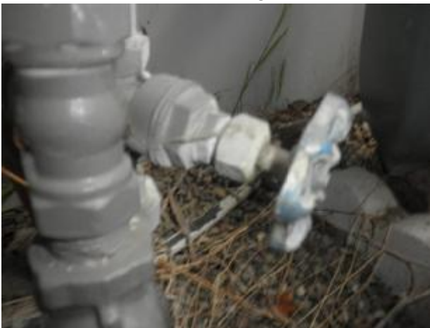
Leak at the main water shut off valve.
