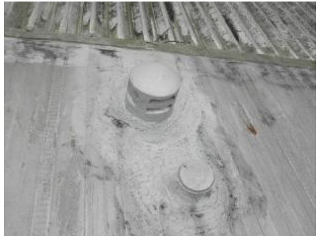
Sealant around the furnace exhaust flue.
