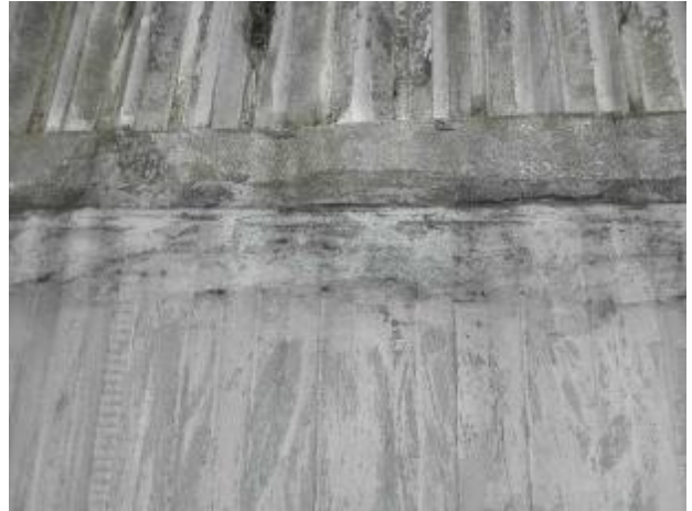
Deteriorated sealant at the perimeter.
