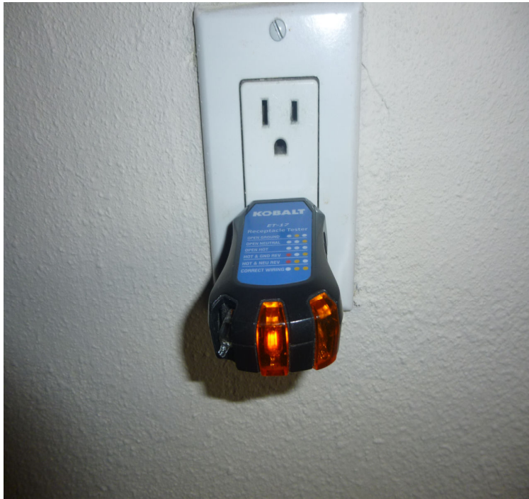
OPEN GROUND ON WALL OUTLETS IN GARAGE/OUTLETS ARE NOT GROUNDED BY TODAY'S STANDARDS RECOMMEND EVALUATION
