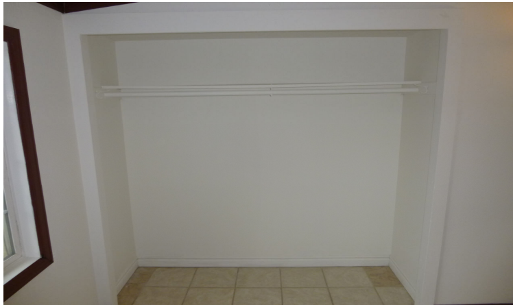
MISSING CLOSET DOORS IN MASTER BEDROOM REPLACE/ INSTALLMENT NEEDED
