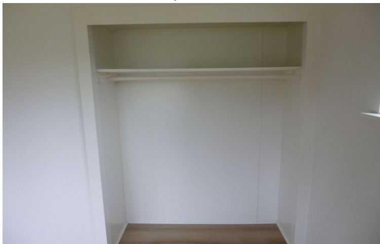
MISSING CLOSET DOORS IN LAST HALL BEDROOM ON RIGHT REPLACE/INSTALLMENT NEEDED
