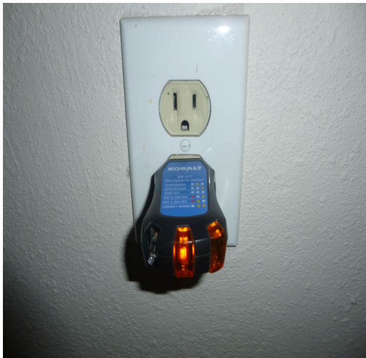
OPEN GROUND ON WALL OUTLETS IN GARAGE/OUTLETS ARE NOT GROUNDED BY TODAY'S STANDARDS RECOMMEND EVALUATION
