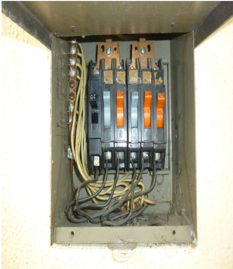
MISSING INSIDE BREAKER COVER AT MAIN ELECTRICAL PANEL REAR OF HOUSE INSTALLMENT NEEDED
