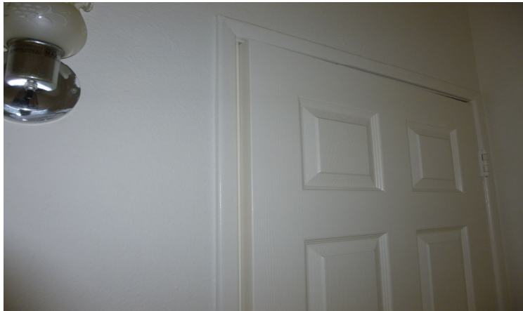
LAST HALL BEDROOM ON LEFT DOOR WONT CLOSE/LATCH PROPERLY REPAIR/ADJUSTMENT NEEDED
