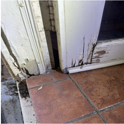
3a Fungus infection back door frame and door
