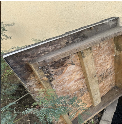
3-D Fungus infection subfloor entrance door
