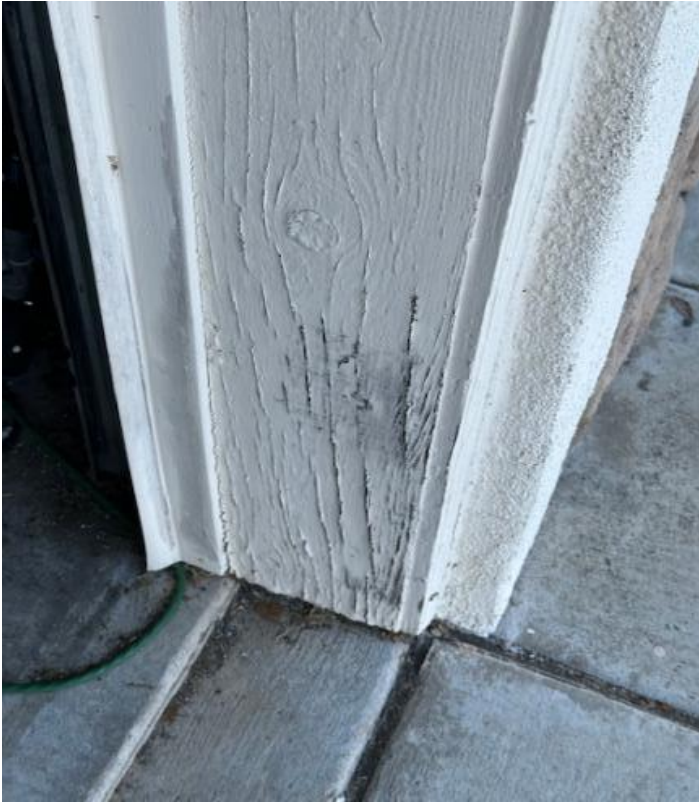
4A - WEATHERING/PEELING PAINT/CRACKING WOOD MEMBERS
