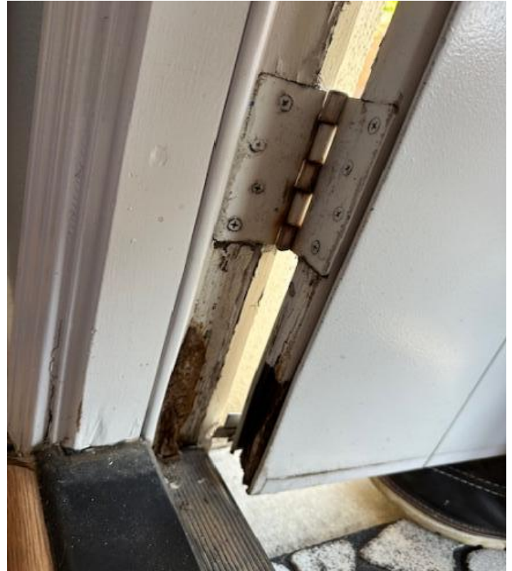
3D - FUNGUS DAMAGE TO THE BACK 1 LITE EXTERIOR DOOR
