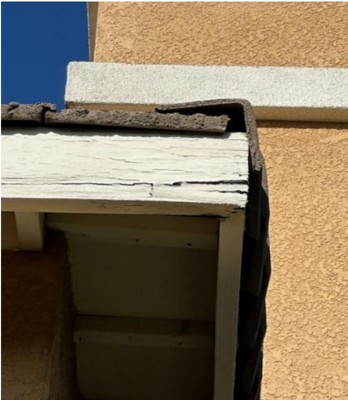
3A - FUNGUS DAMAGE TO THE FASCIA
