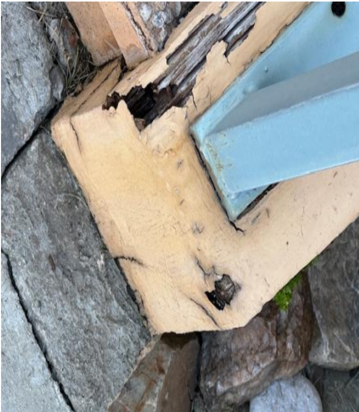
3C - FUNGUS DAMAGE TO THE STAIR STRINGER
