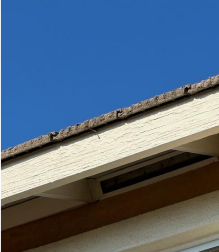
4A - WEATHERING/PEELING PAINT/CRACKING WOOD MEMBERS
