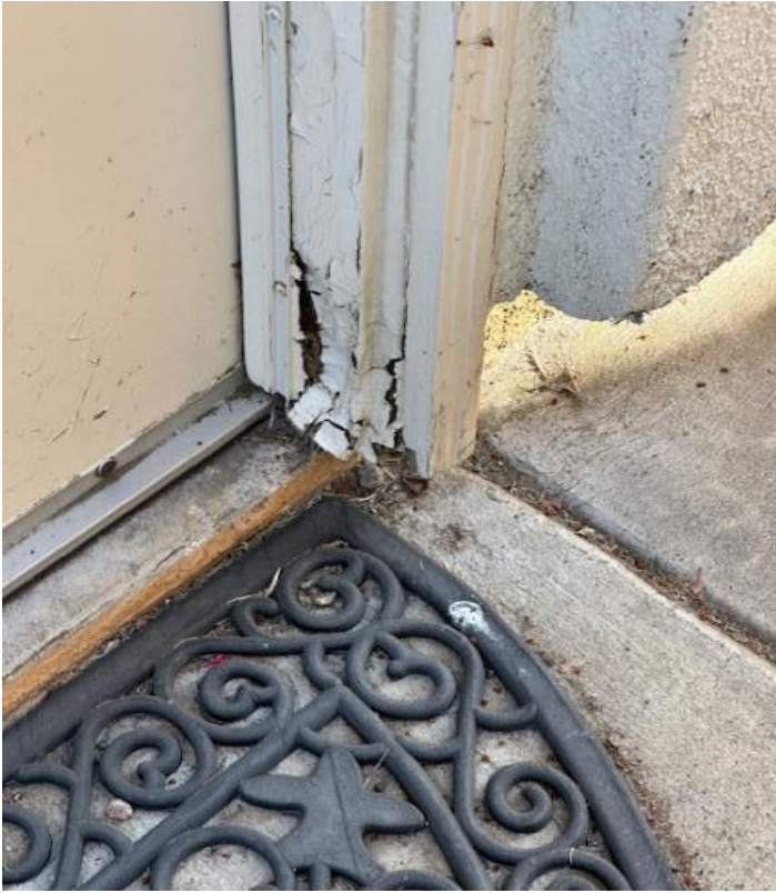
3B - FUNGUS DAMAGE TO THE GARAGE MAN DOOR JAMB
