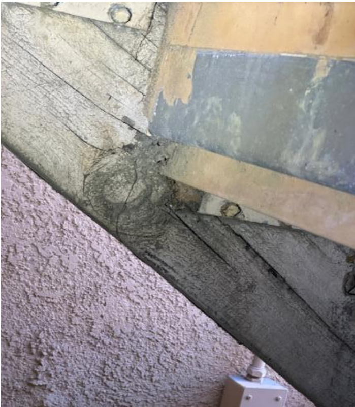
3C - FUNGUS DAMAGE TO THE STAIR STRINGER (UNDER STAIRS VIEW)
