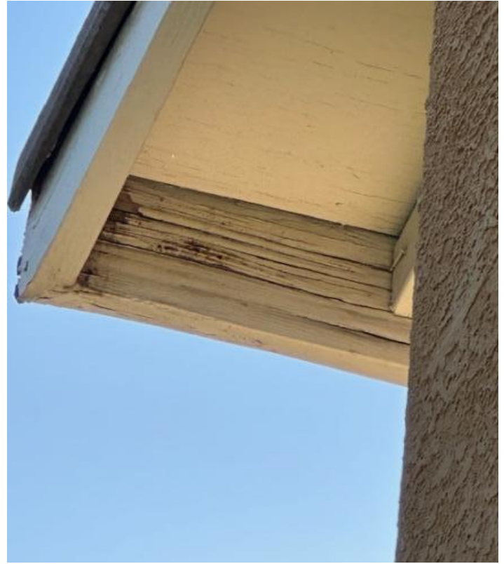
3A - FUNGUS DAMAGE TO THE FASCIA
