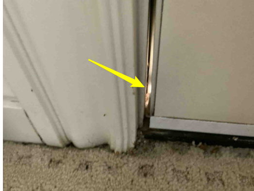
Some visible daylight between the door and the door jam
