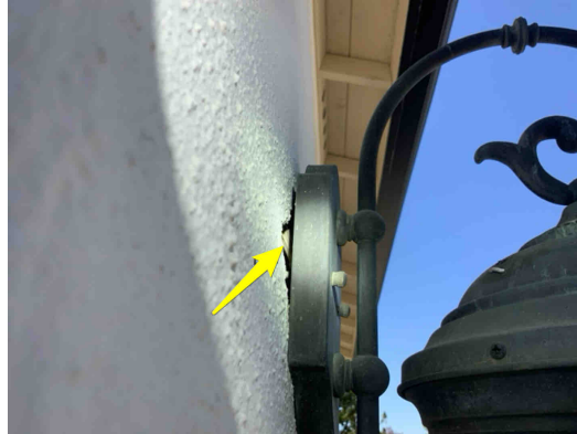
Exposed electrical wires, subject to water intrusion deterioration
