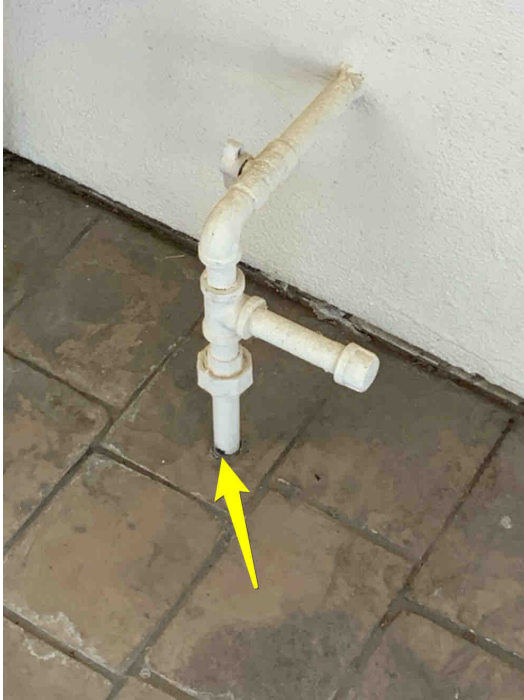
Not sleeved through the concrete
