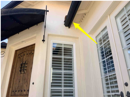
A loose and displaced roof tile above the water damaged area.
