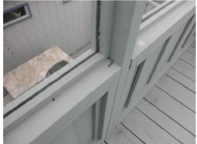
Example of the moisture damage at the backyard wood deck and stairs.
