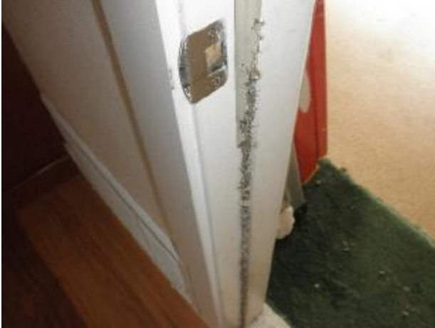
Weather stripping damaged at the garage fire door.
