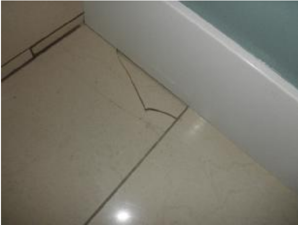
Broken floor tile in the master bathroom.
