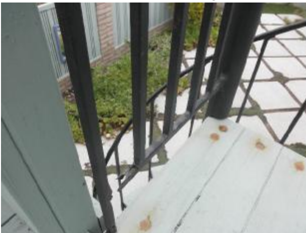
Rust damage to the railing at the top of the spiral stairs.
