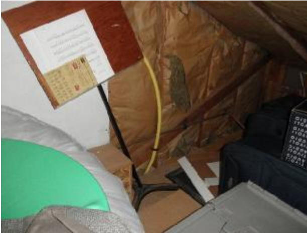
Yellow coated CSST piping in the attic.
