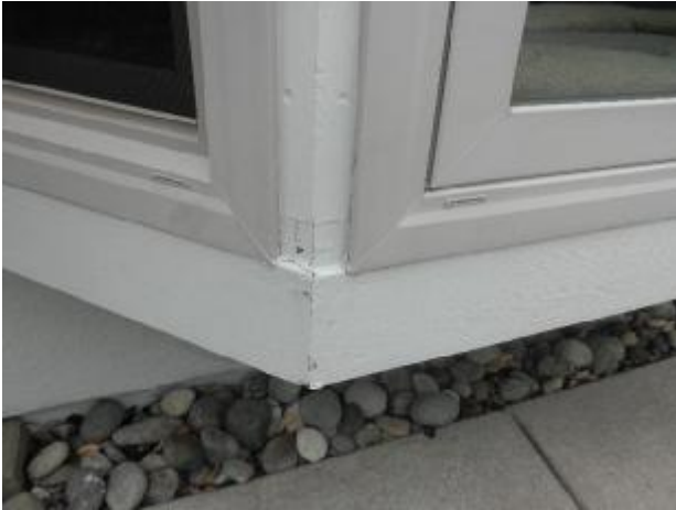
Moisture damage to the wood trim below the bay window.
