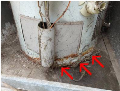
ROTTED WATER HEATER NOTED
