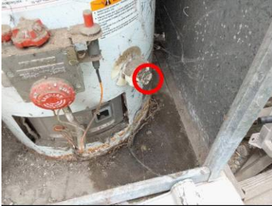
LEAKING DRAIN VALVE NOTED
