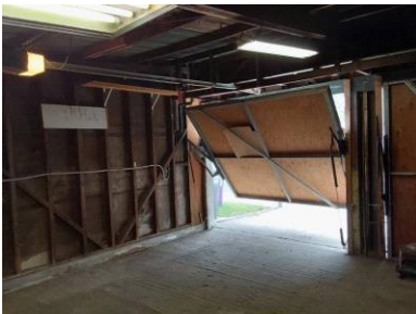
GARAGE DOOR OPENER ADJUSTMENTS NEEDED
