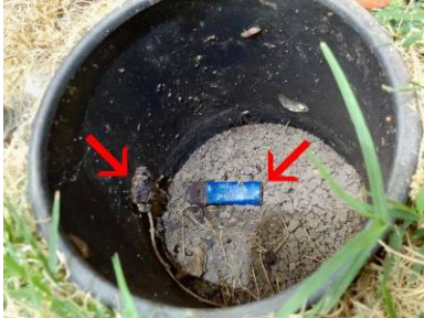
CUTOFF VALVE REPLACEMENT NEEDED
