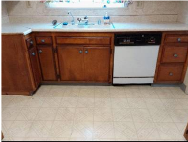
CABINET FINISH REPAIR/REFINISHING NEEDED
