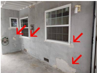
EXTERIOR WALL REPAIR/REFINISHING NEEDED
