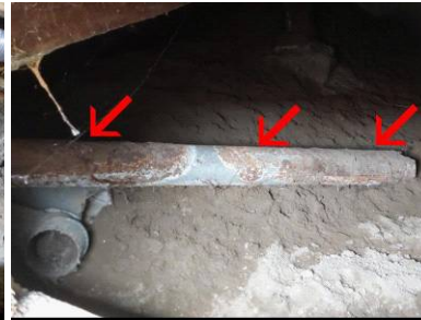
OLD WASTE PIPE REMOVAL NEEDED
