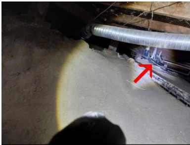
ADDITIONAL PIPE HANGERS ARE NEEDED
