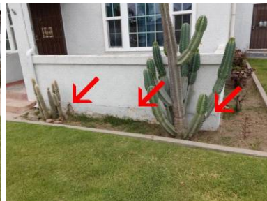
EXTERIOR WALL REPAIR/REFINISHING NEEDED
