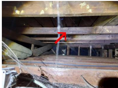
CRACKED ROOF RAFTER NOTED
