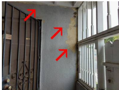
EXTERIOR WALL REPAIR/REFINISHING NEEDED
