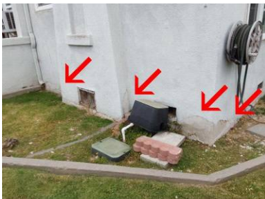
EXTERIOR WALL REPAIR/REFINISHING NEEDED
