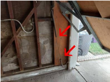
BROKEN DOOR SPRINGS NOTED
