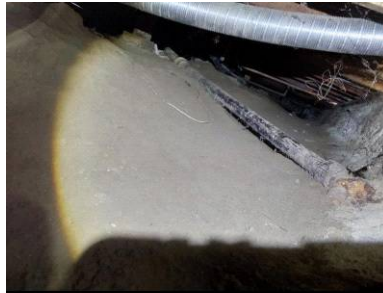
OLD WASTE PIPE REMOVAL NEEDED
