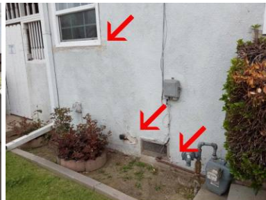
EXTERIOR WALL REPAIR/REFINISHING NEEDED
