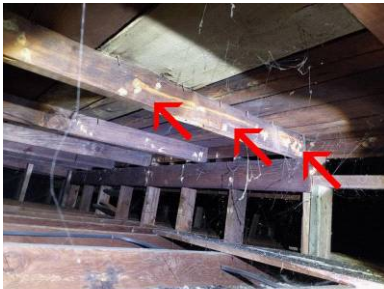
TERMITE DAMAGE NOTED
