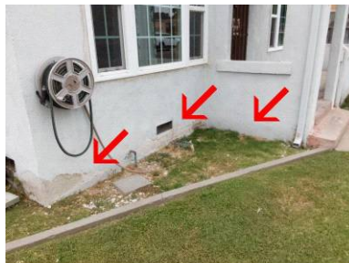
EXTERIOR WALL REPAIR/REFINISHING NEEDED
