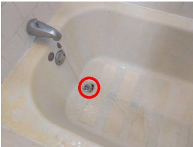
DAMAGED TUB FINISH NOTED
