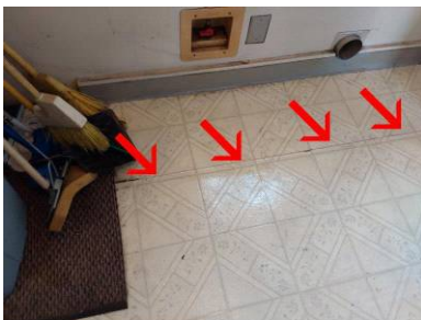
FLOOR COVERING REPAIRS ARE NEEDED
