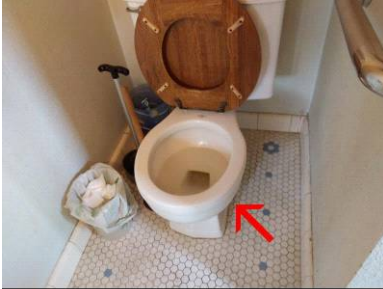
LOOSE TOILET NOTED
