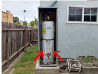
WATER HEATER SAFETY STRAPS REQUIRED.
