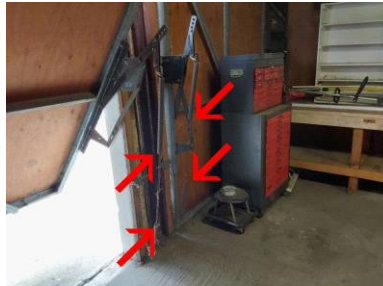
BROKEN DOOR SPRINGS NOTED
