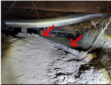
OLD WASTE PIPE REMOVAL NEEDED
