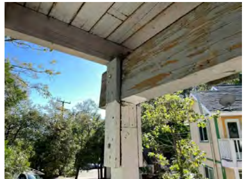
South/ Spliced post, Not properly bracketed.
