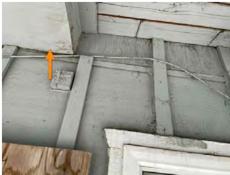
Cant see under the sheeting under the room addition
