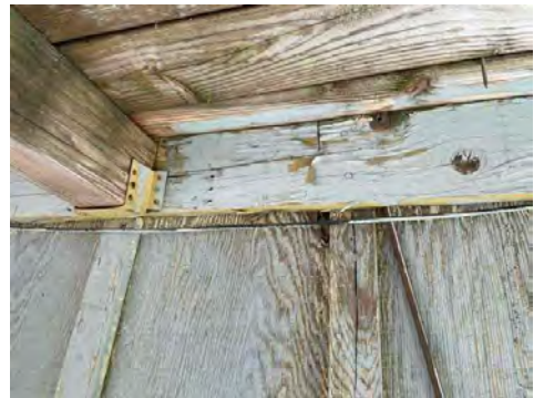
South ledger board not secured to home correctly
