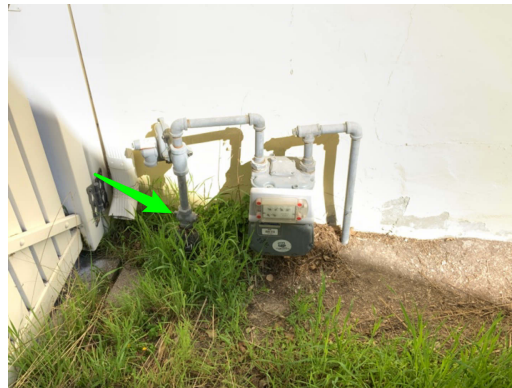
Main gas shut off valve
