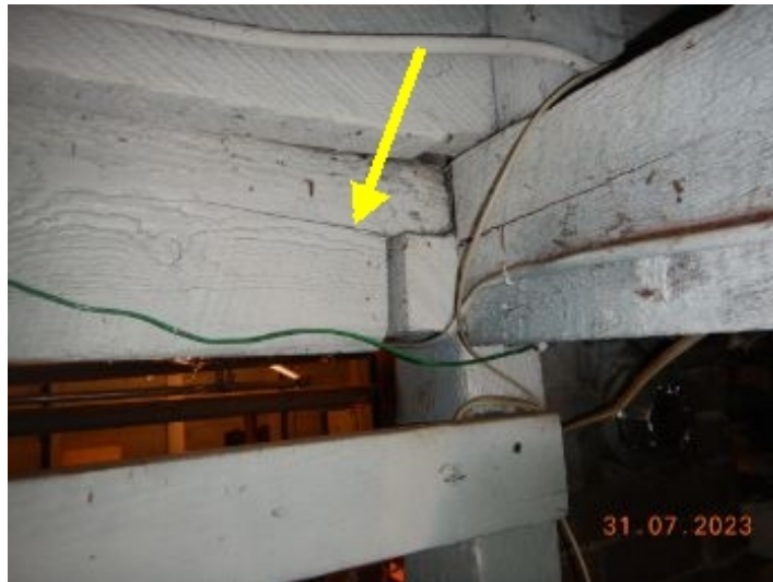
Crack in girder
