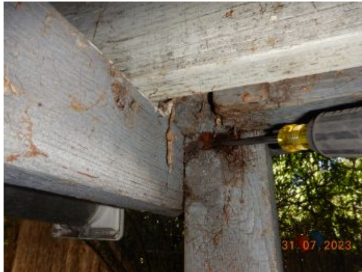
Wood decay at top of support post
