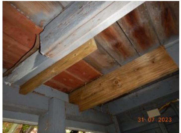
Spliced floor joist
