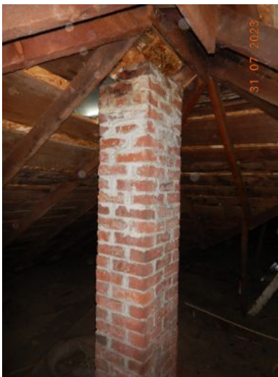
Unsupported chimney chase
