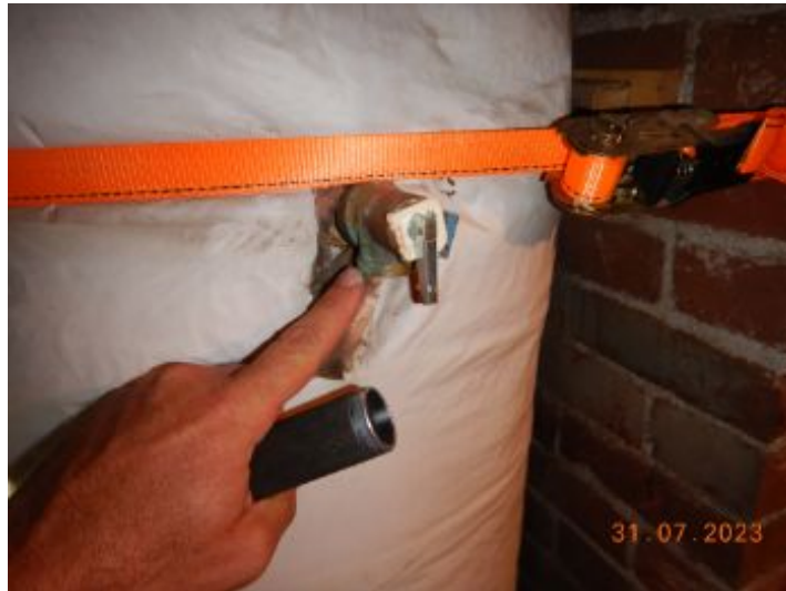
Missing T&P valve
