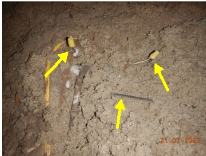
Example of knob and tube wiring
