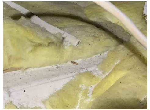
Electrical Wire Not Capped
