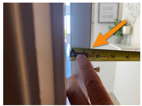
Not A Fire Rated Door
