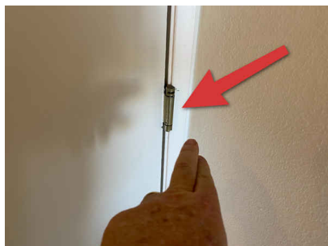
Tension Hinge Deficiency
