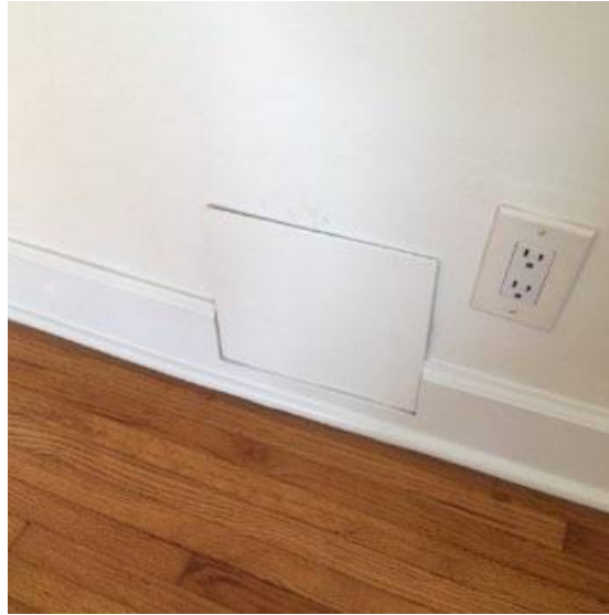
Photo 161-4 Plumbing access was sealed shut. Recommend having a qualified person repair as plumbing is easily accessible.
