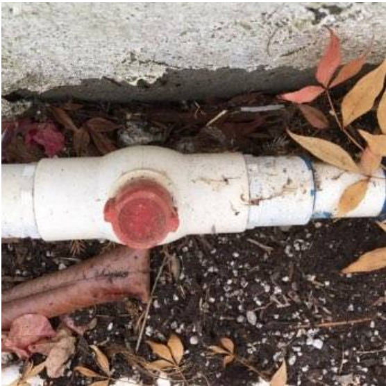
Photo 108-3 Handle was damaged at sprinkler plumbing line.
