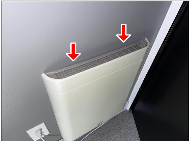
4.0 Item 1(Picture) Heating/Central Air
