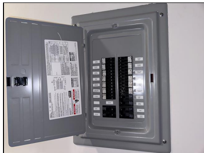
6.4 Item 1(Picture) Electrical System
