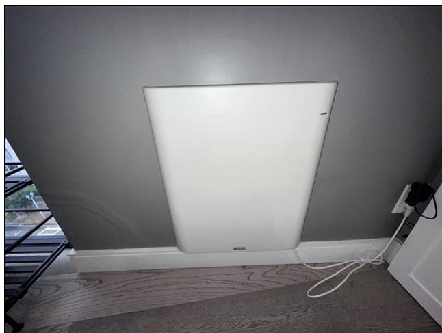
4.0 Item 2(Picture) Heating/Central Air
