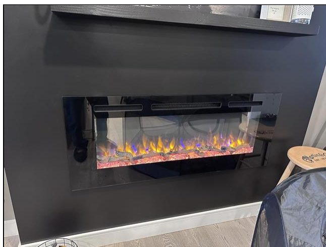
4.0 Item 3(Picture) Heating/Central Air
