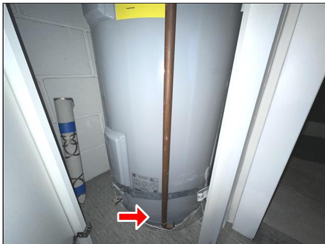
Item 1 - Item 1(Picture) Plumbing System
