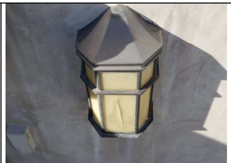
Cracked Light Cover at Rooftop
