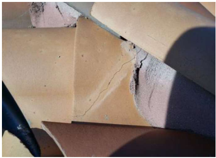
Cracked Tile at Roof
