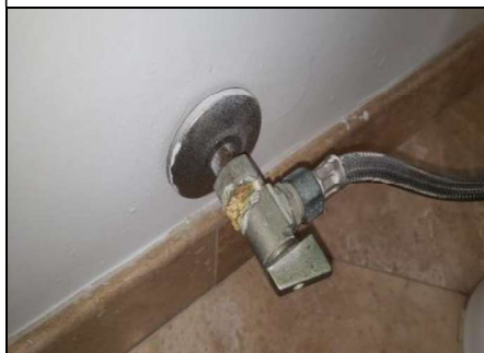
Corrosion at Water Shut Off Valves.
