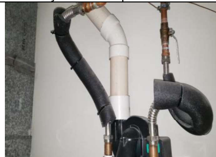
Improper PVC Flue at Water Heater
