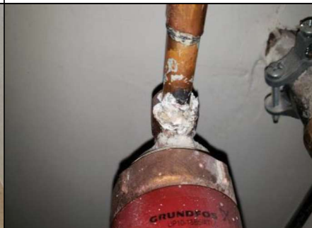
Corrosion at Water Supply Lines
