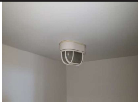
Inoperable Pantry Light
