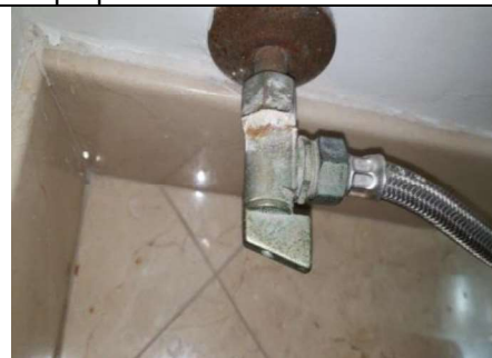
Corrosion at Water Shut Off Valves.
