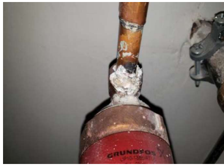
Corrosion at Water Supply Lines
