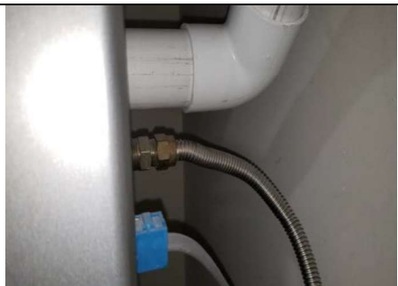
Furnace Fuel Line Missing Drip Leg
