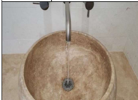
Low Water Flow at Bathroom Sink
