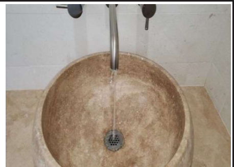
Low Water Flow at Bathroom Sink
