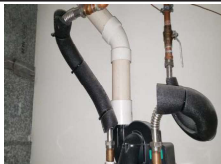
Improper PVC Flue at Water Heater
