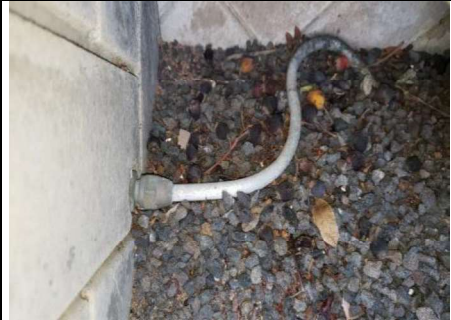
Improper Gas Line for Fireplaces
