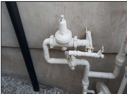
Water Shut Off
