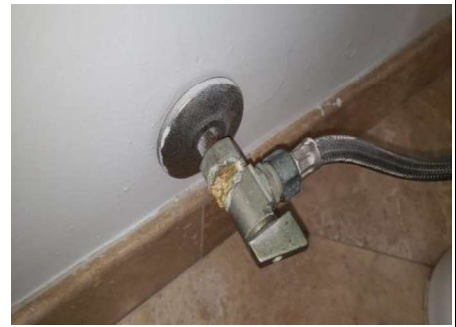
Corrosion at Water Shut Off Valves.
