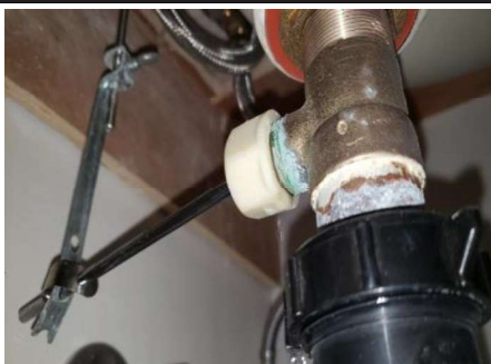
Leak at Bathroom Sink Drain
