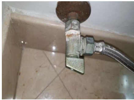
Corrosion at Water Shut Off Valves.
