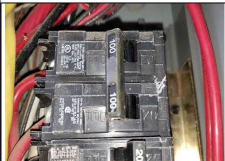
100 Amp Breaker in Off Position
