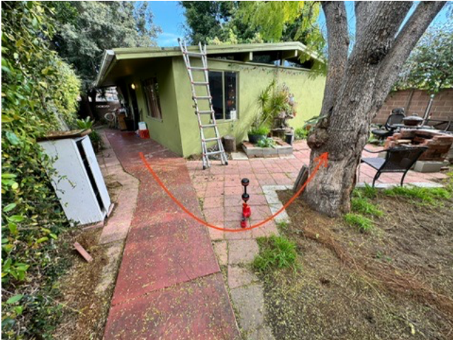
Continued path of sewer line. Good location for a cleanout to be installed under tool 3' deep.
