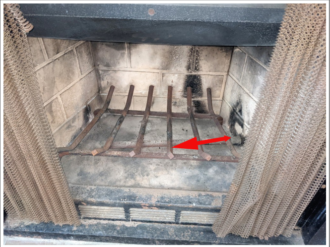
Fireplace, improper size grate, damper not opening fully
