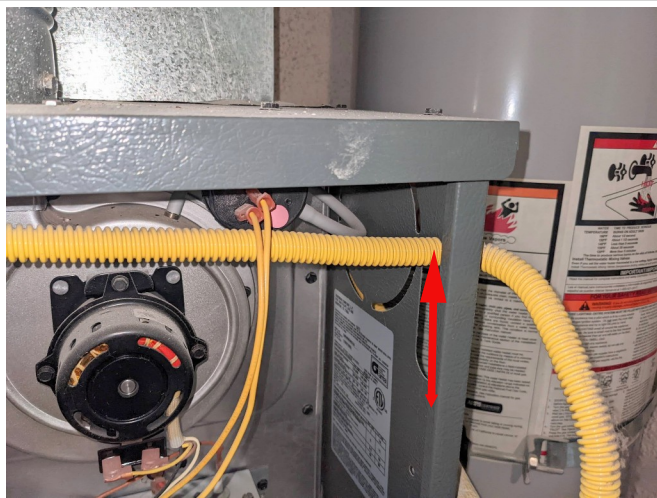
Gas piping incorrect to furnace
