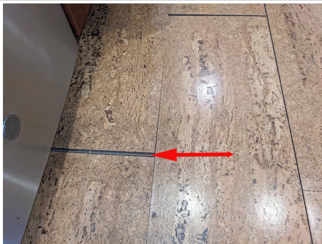
Kitchen flooring joint separations
