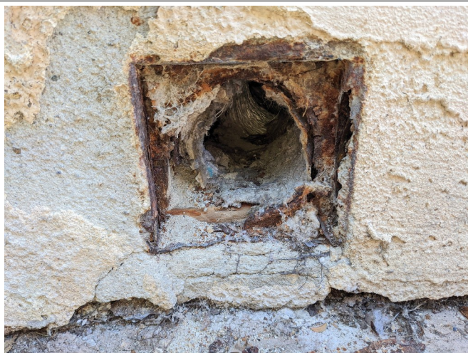
Missing dryer vent termination
