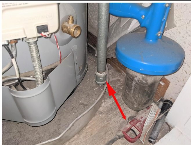
Water heater TPR drain pipe end cannot be threaded
