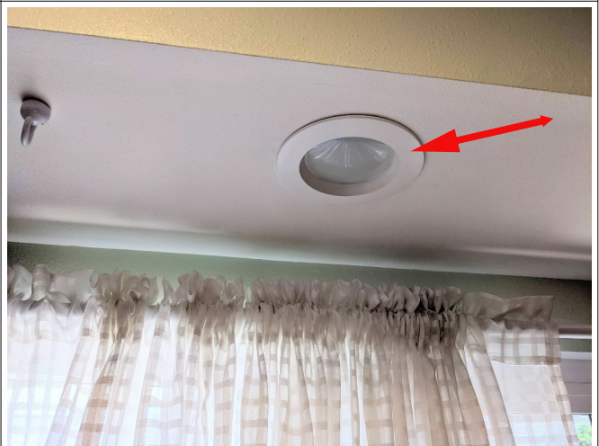
Kitchen light inoperable
