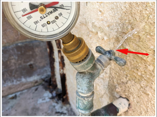
Hose bib leaking
