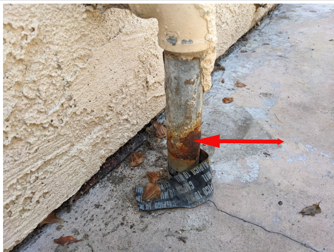
Rust at gas piping
