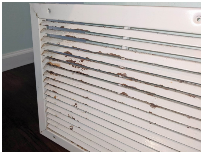
Furnace air intake grill rusting
