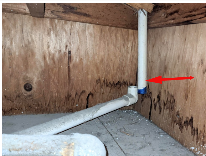
Water heater overflow drain pipe not connected
