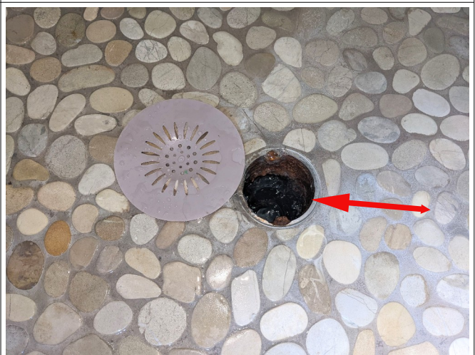
Master shower missing metal drain cover
