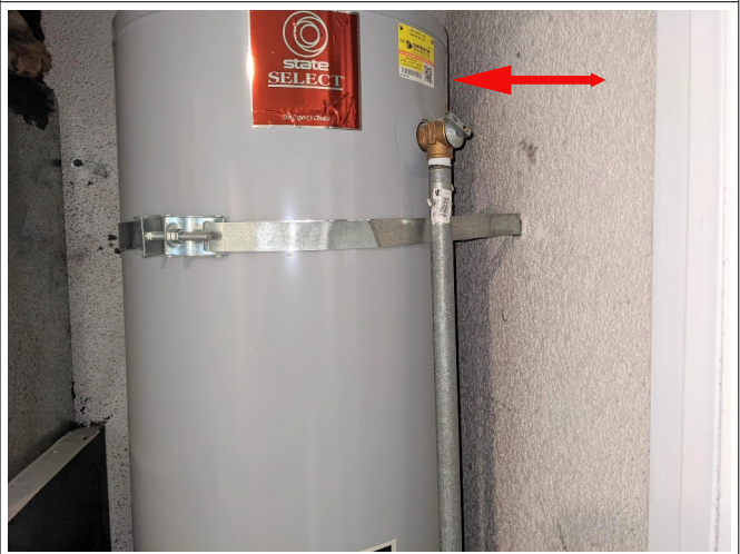
Water heater lacks wood blocking to wall
