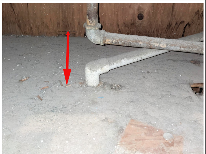
Dust/debris build up under furnace
