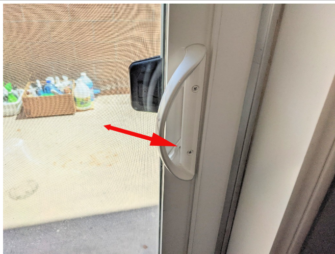
Sliding door does not lock
