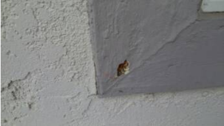
There is damage to the wood trim that should be evaluated by a termite inspector.
