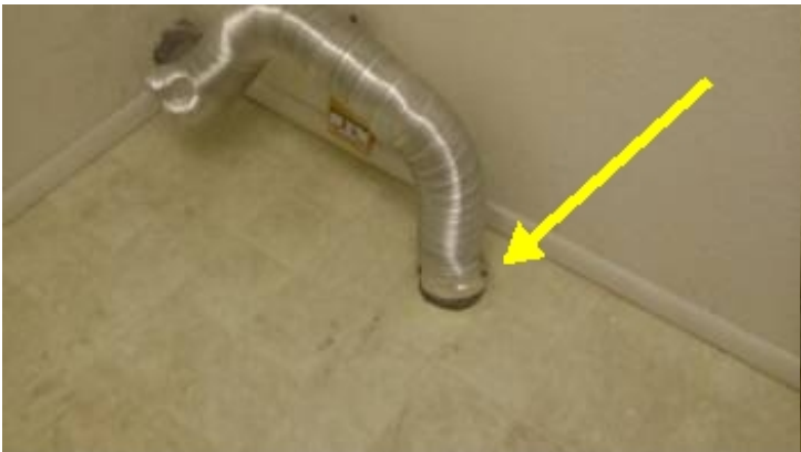
The dryer vent is routed through an inaccessible substructure and should be serviced.
