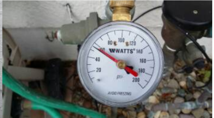
A functional pressure regulator is in place on the plumbing system.
