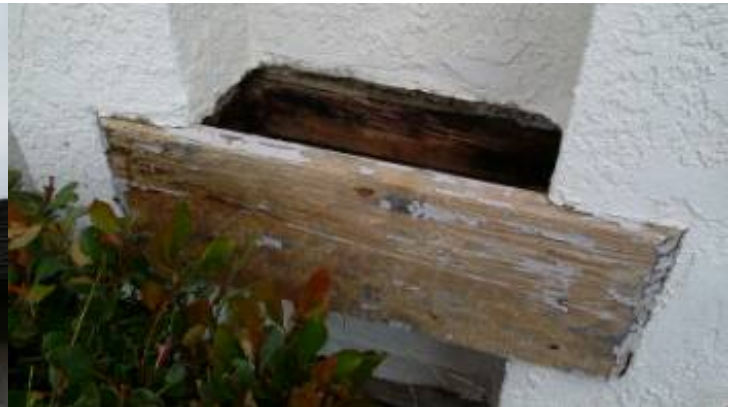
There is damage to the wood trim that should be evaluated by a termite inspector.
