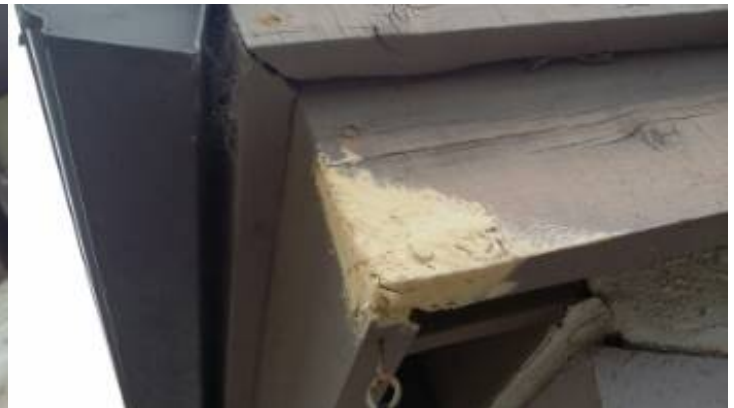
The termite report should confirm moisture, dry rot or insect damage to the fascia board and or eaves of the roof.
