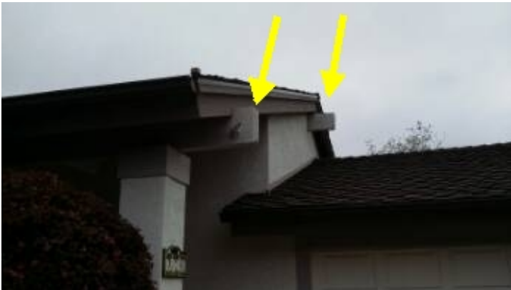
There is moisture damage or dry rot to the wood trim and or fascia on the upper roof area, which is typically not inspected by the pest inspector. The pest control company should be alerted so as to inspect and include these repairs in their estimate.
