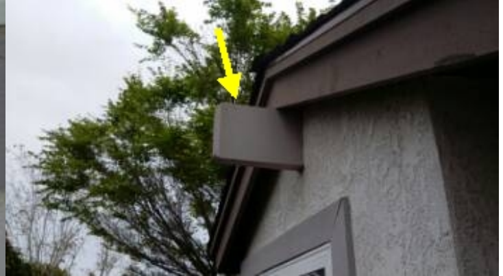
There is moisture damage or dry rot to the wood trim and or fascia on the upper roof area, which is typically not inspected by the pest inspector. The pest control company should be alerted so as to inspect and include these repairs in their estimate.
