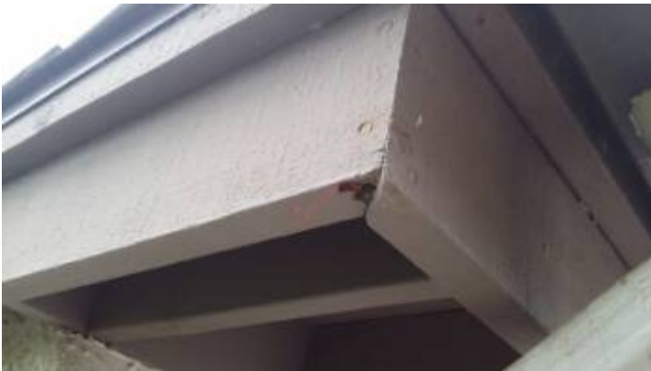
There is damage to the wood trim that should be evaluated by a termite inspector.
