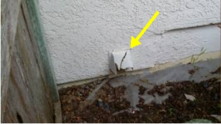
Damaged dryer vent
