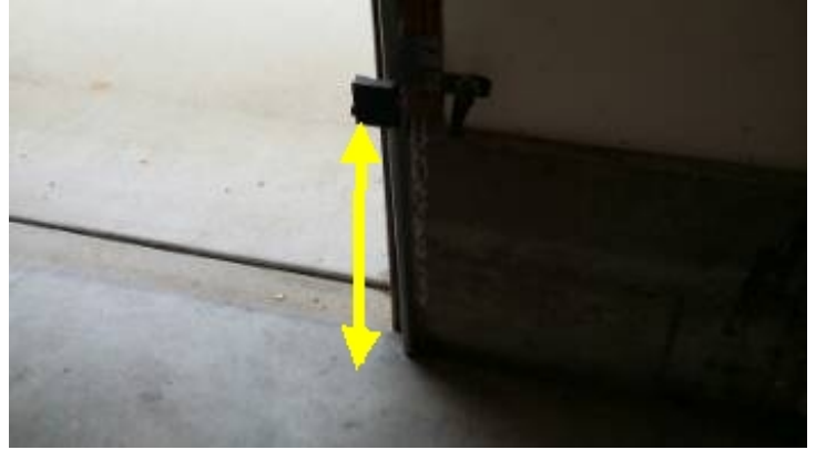
The infra red auto-reversing sensor mechanisms are functional but located higher than the recommend six inches above grade.
