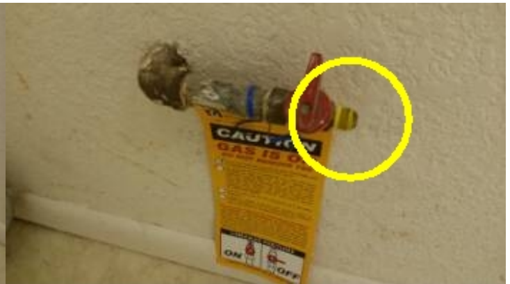
A gas supply valve is installed but needs an approved connector to connect gas to the dryer, which is not required and you should have one already installed if you have a gas dryer. Gas valve is required to be capped when not in use.
