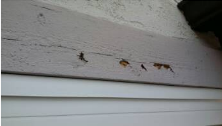
The termite report should confirm moisture, dry rot or insect damage to the fascia board and or eaves of the roof.
