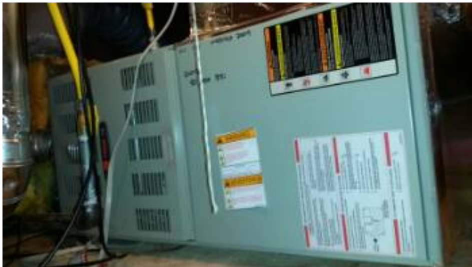
Central heat is provided by a forced-air furnace that is located in the attic.
