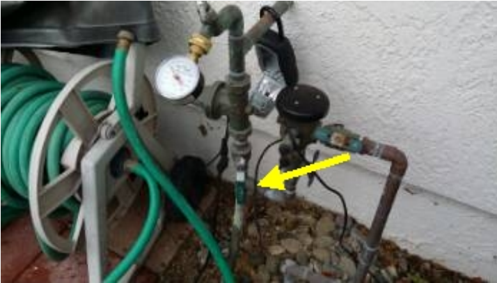
The main water shut-off valve is located at the right side of the house.
