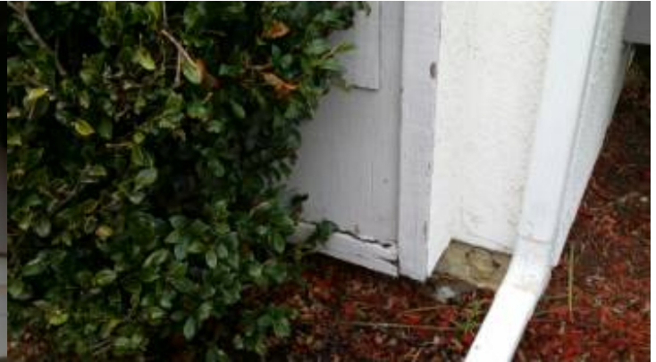
There is damage to the wood trim that should be evaluated by a termite inspector.
