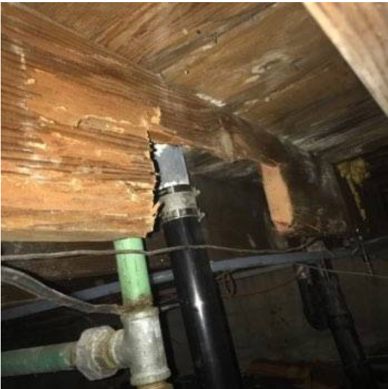
Photo 46-3 One or more joists were notched or had holes cut in them in such a way as to significantly weaken the joist(s)
