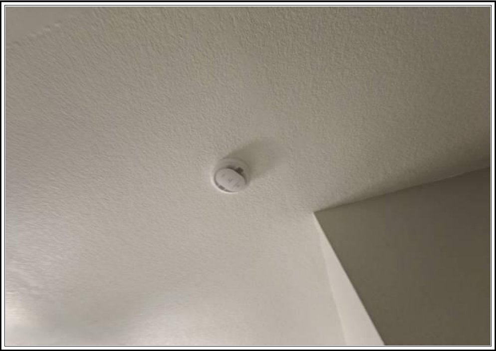
Smoke and Carbon Monoxide Detector
