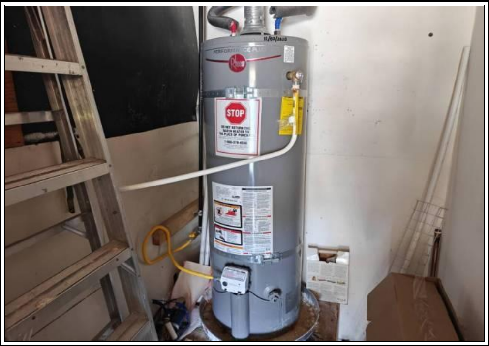
Water Heater Double Strapped
