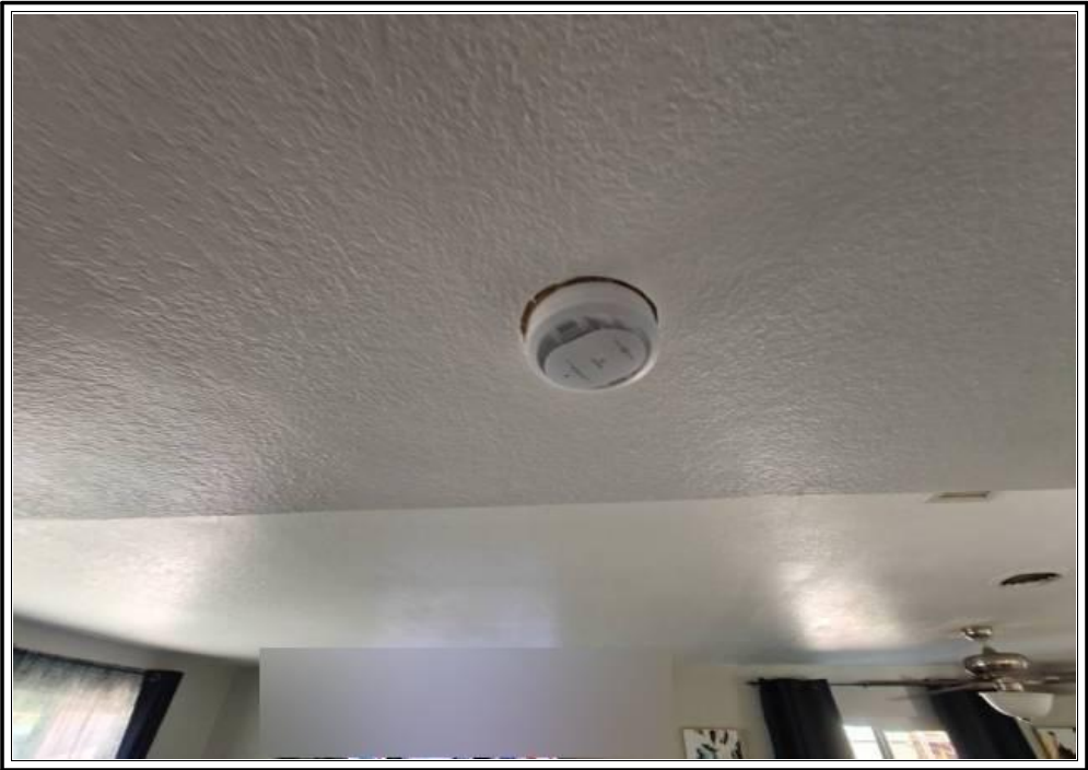
Smoke and Carbon Monoxide Detector
