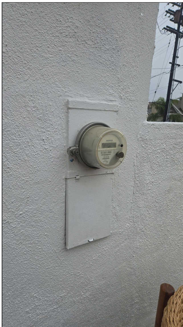
4.1 Item 1 (Picture) Electric meter and main distribution panel
