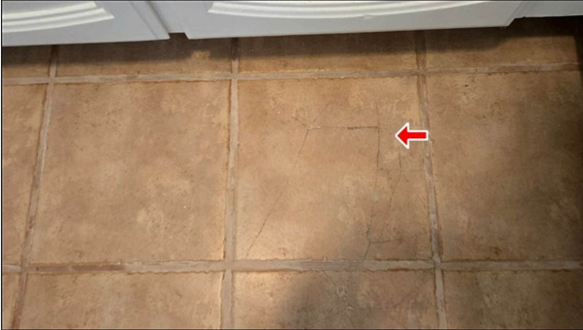
3.2 Item 1 (Picture) Kitchen floor tile, hairline cracks
