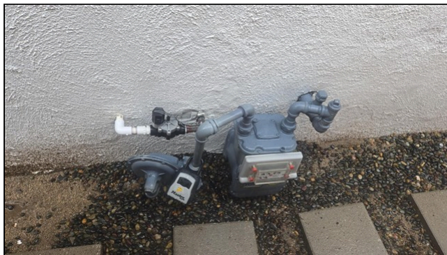
5.1 Item 1 (Picture) Gas meter and main shut off
