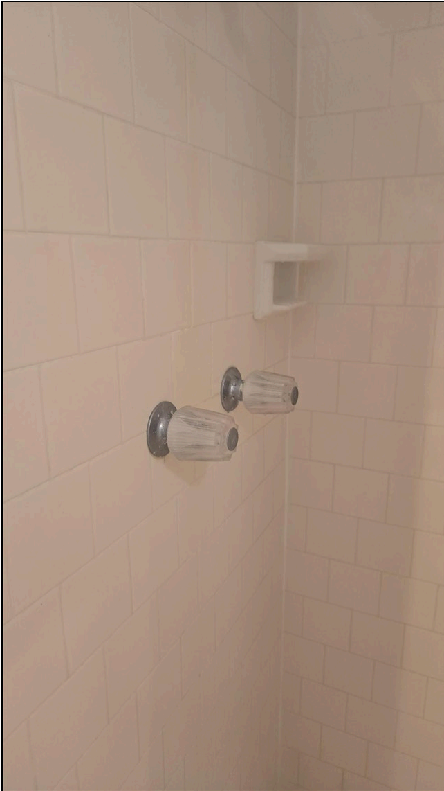
5.4 Item 3 (Picture) Dated water supply, lower level hall bathroom
