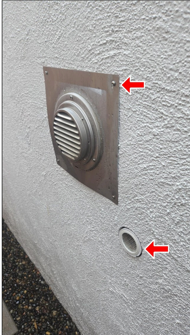
1.0 Item 1 (Picture) Gaps, missing seal, exterior wall
