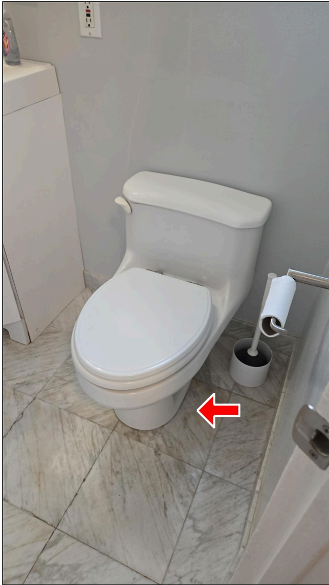
5.6 Item 1 (Picture) Loose toilet, upper hall bathroom
