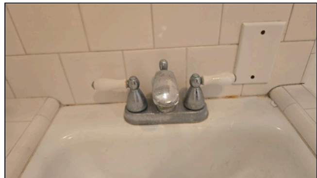
5.4 Item 2 (Picture) Dated water supply, lower level hall bathroom
