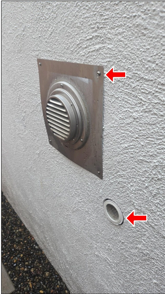
1.0 Item 1 (Picture) Gaps, missing seal, exterior wall
