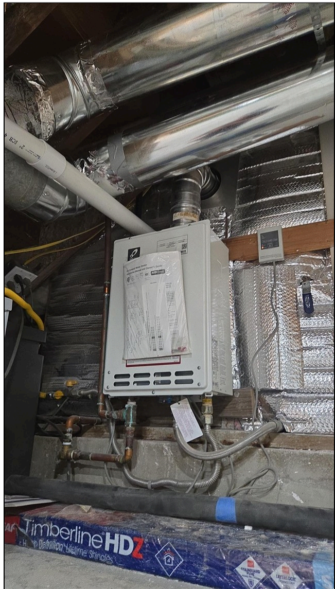
5.2 Item 1 (Picture) Tankless water heater
