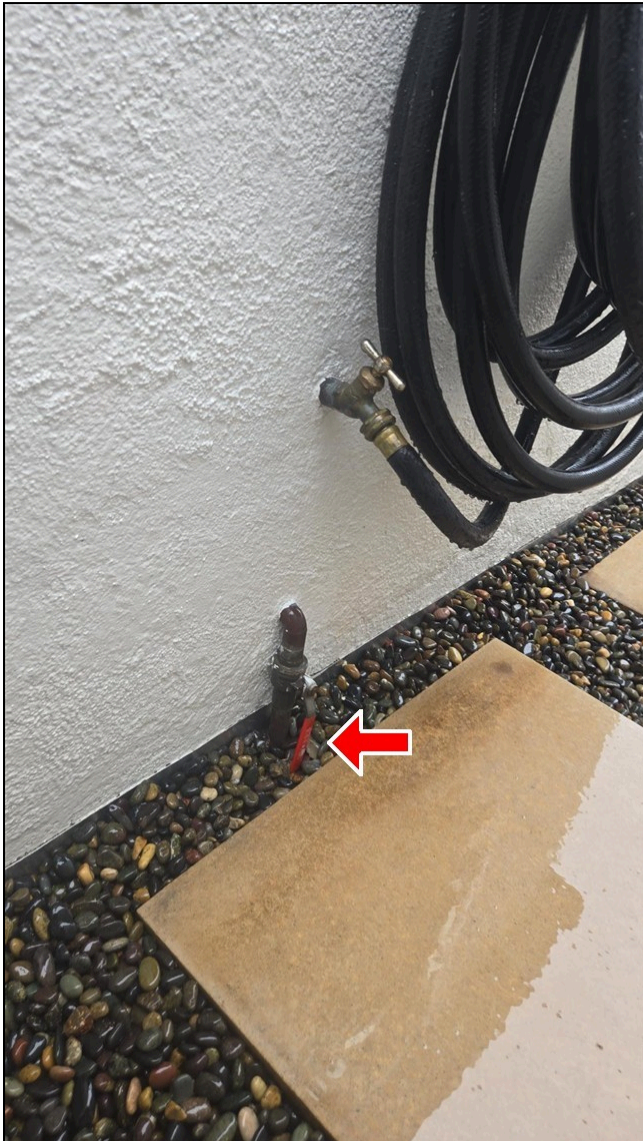
5.0 Item 1 (Picture) Main water shut off
