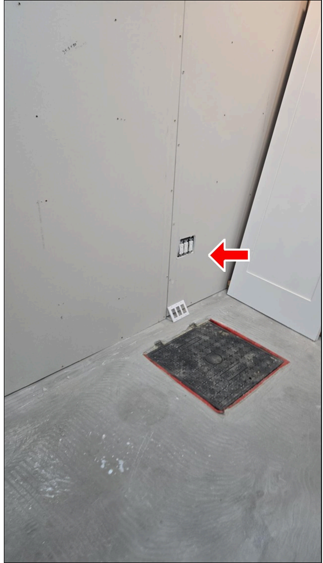
4.4 Item 2 (Picture) Missing cover plates, basement
