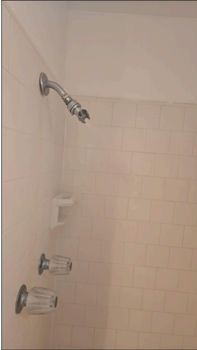
5.4 Item 4 (Picture) Lower level bathroom shower head missing
