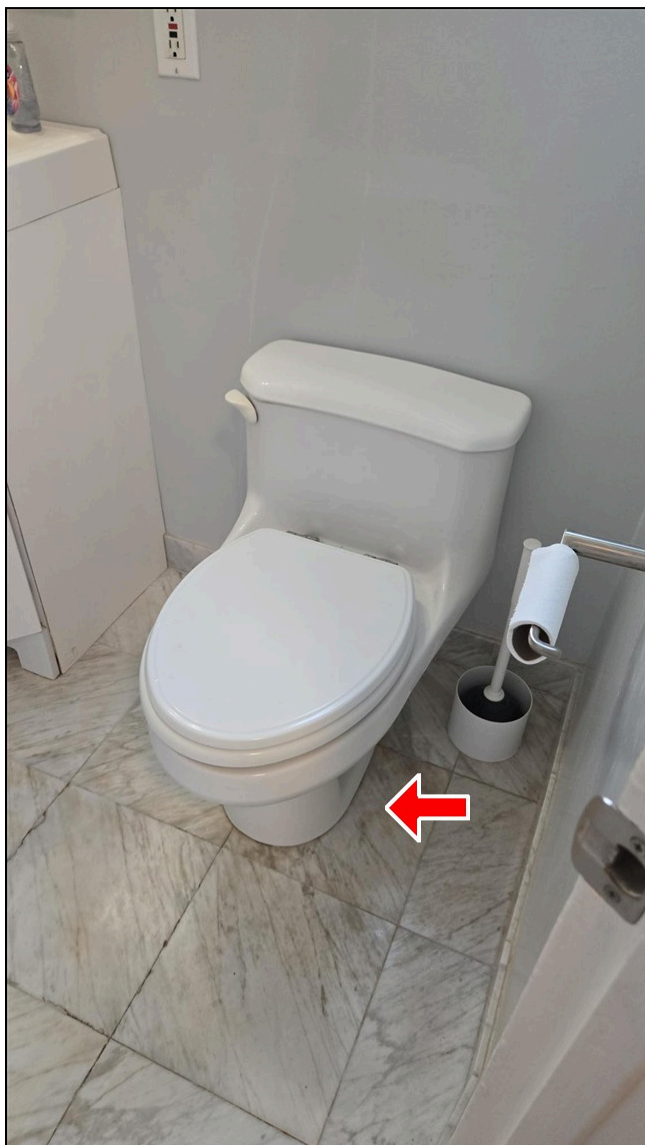
5.6 Item 1 (Picture) Loose toilet, upper hall bathroom
