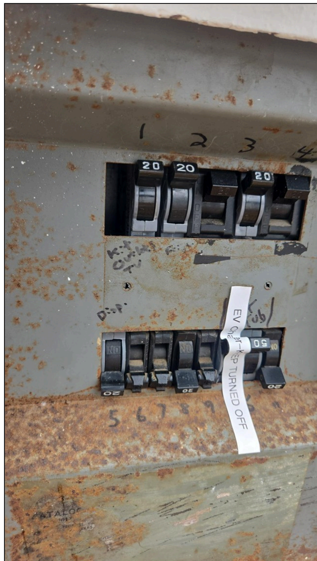
4.2 Item 1 (Picture) Missing labels, main distribution panel
