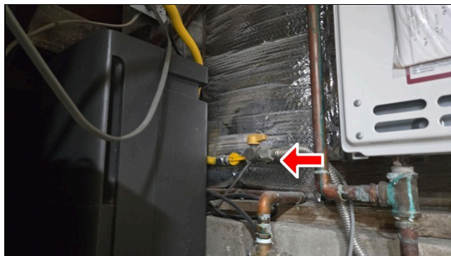
5.7 Item 1 (Picture) Heat system/water heater gas line
