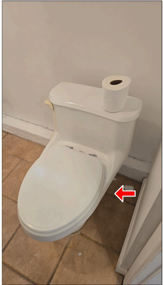
5.6 Item 2 (Picture) Loose toilet, lower level hall bath
