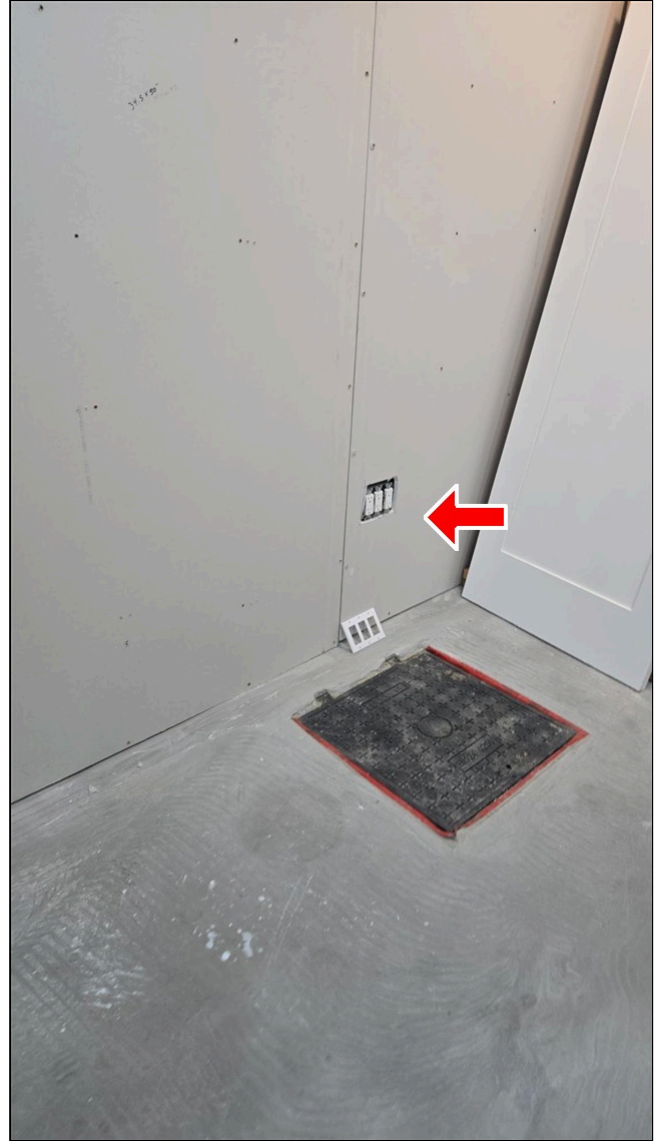
4.4 Item 2 (Picture) Missing cover plates, basement
