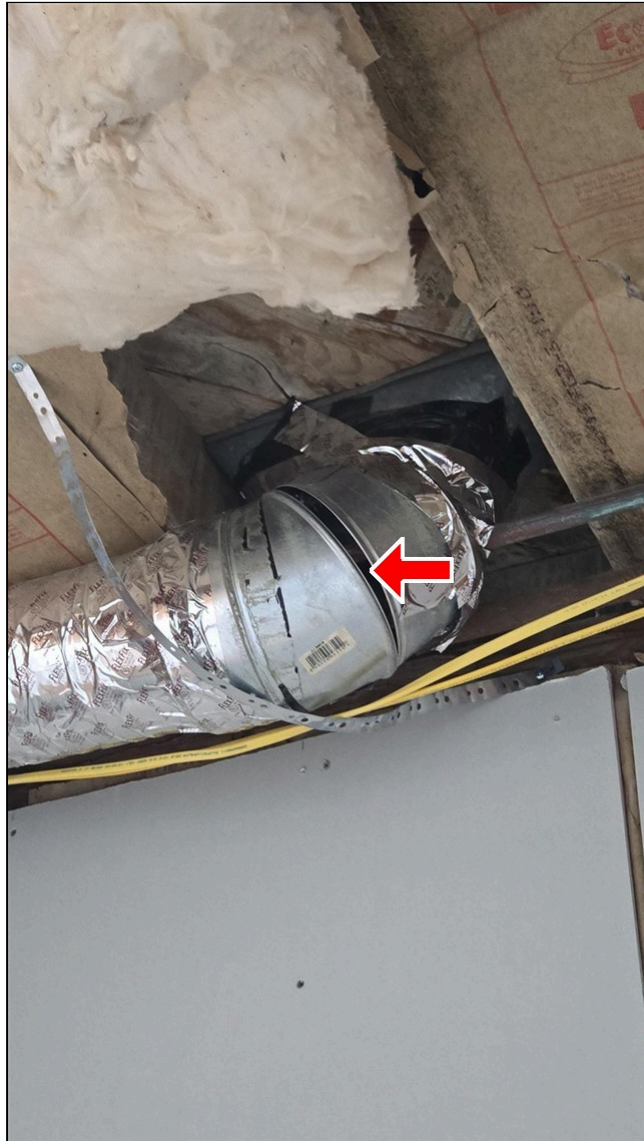
7.3 Item 1 (Picture) Detached ducting, basement
