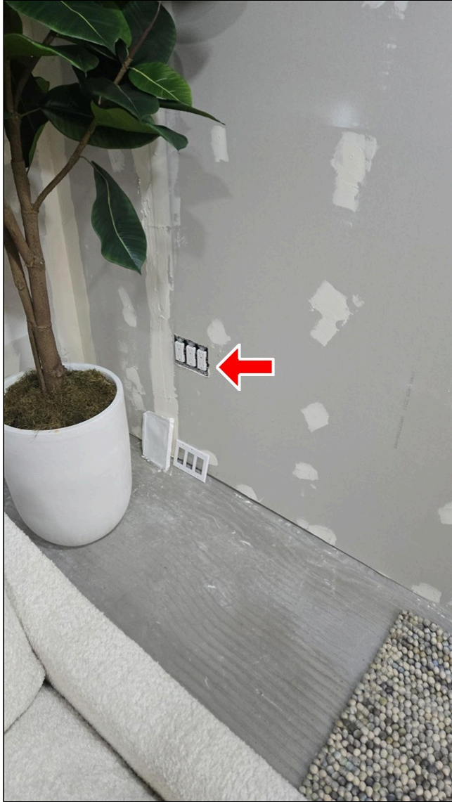
4.4 Item 1 (Picture) Missing cover plates, basement
