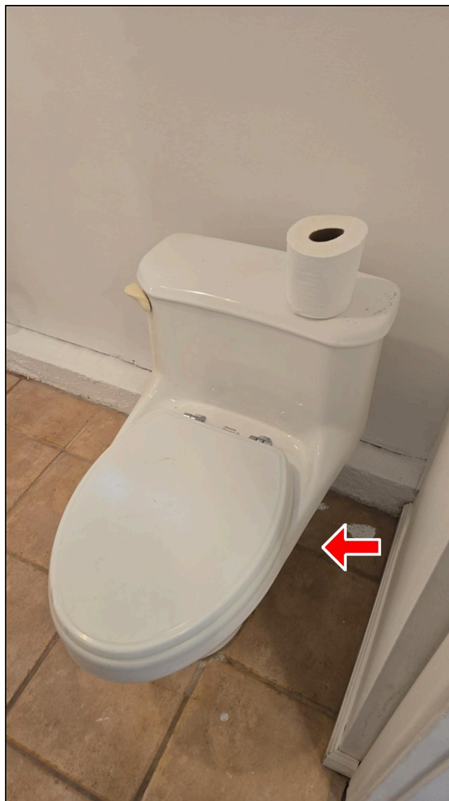
5.6 Item 2 (Picture) Loose toilet, lower level hall bath
