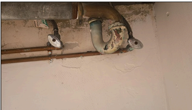
5.4 Item 1 (Picture) Dated angle valves, lower level hall bathroom
