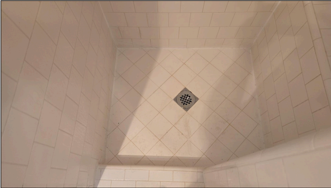
3.3 Item 1 (Picture) Lower level hall bath shower walls
