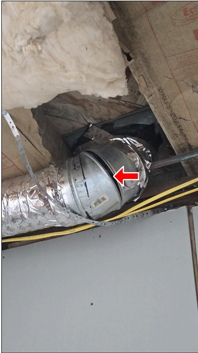
7.3 Item 1 (Picture) Detached ducting, basement
