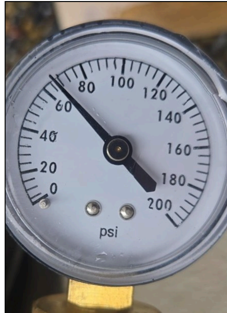
5.0 Item 2 (Picture) Water pressure
