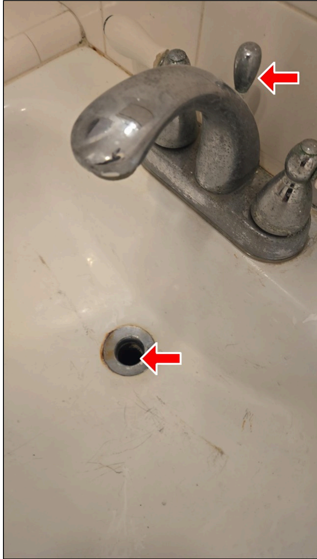
5.6 Item 3 (Picture) Missing drain stop, lower level hall bathroom sink
