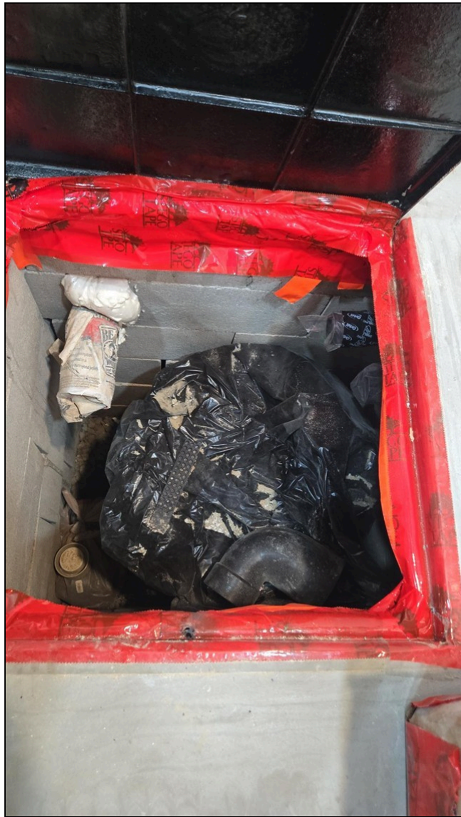
5.8 Item 1 (Picture) Injection/sump pump location, basement
