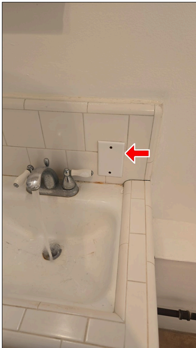
4.5 Item 2 (Picture) Missing GFCI outlet, lower level hall bathroom
