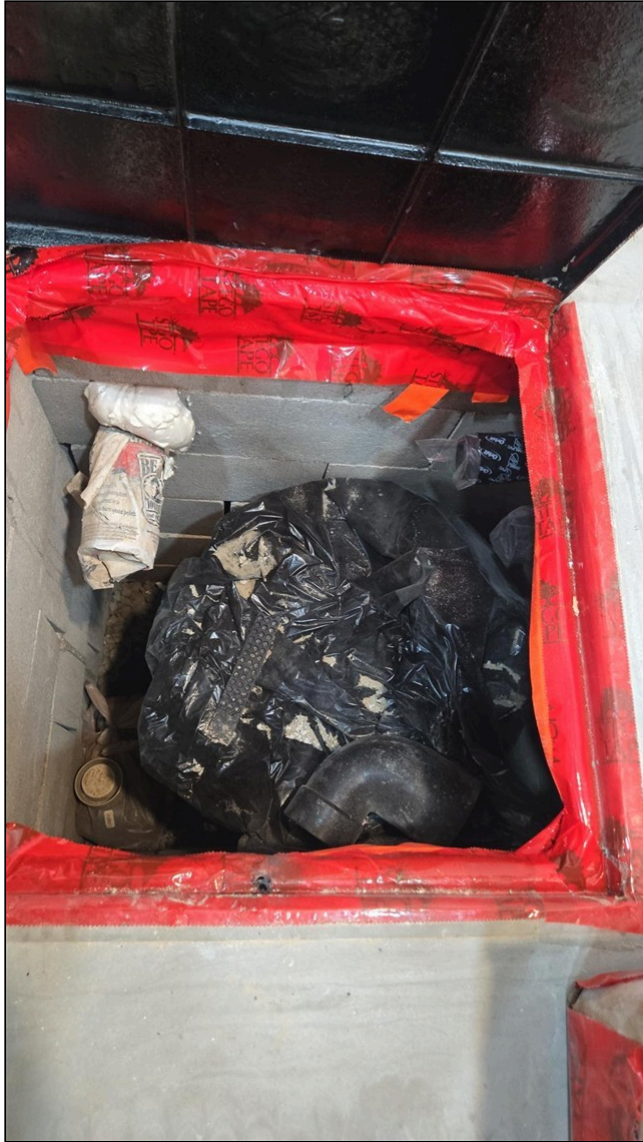
5.8 Item 1 (Picture) Injection/sump pump location, basement
