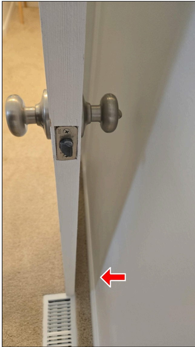
3.6 Item 2 (Picture) Missing door stop
