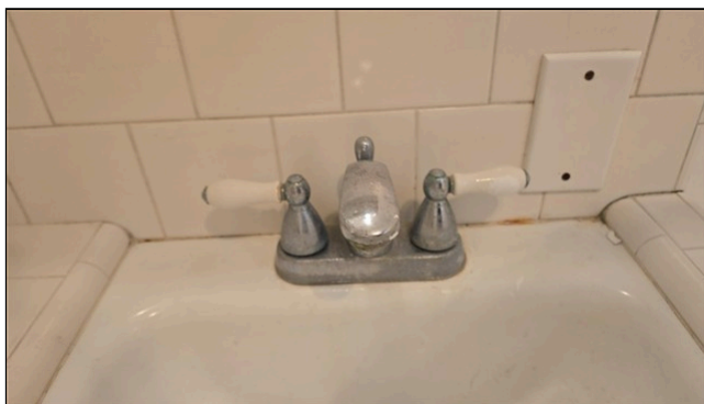
5.4 Item 2 (Picture) Dated water supply, lower level hall bathroom
