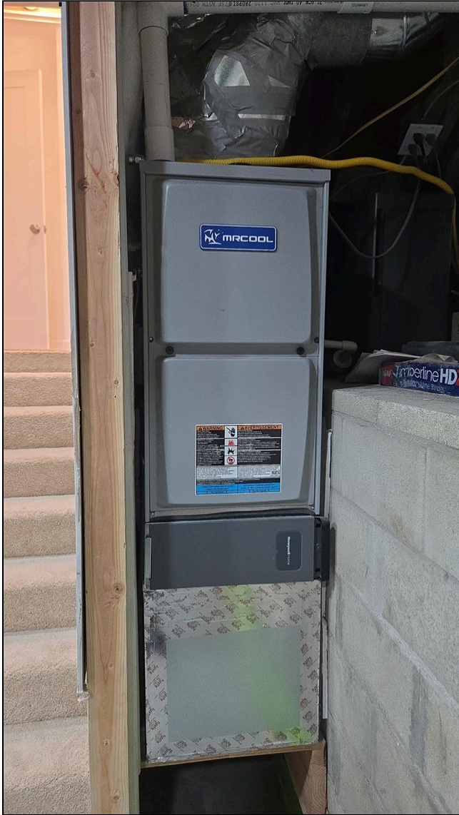
7.0 Item 1 (Picture) Heat system
