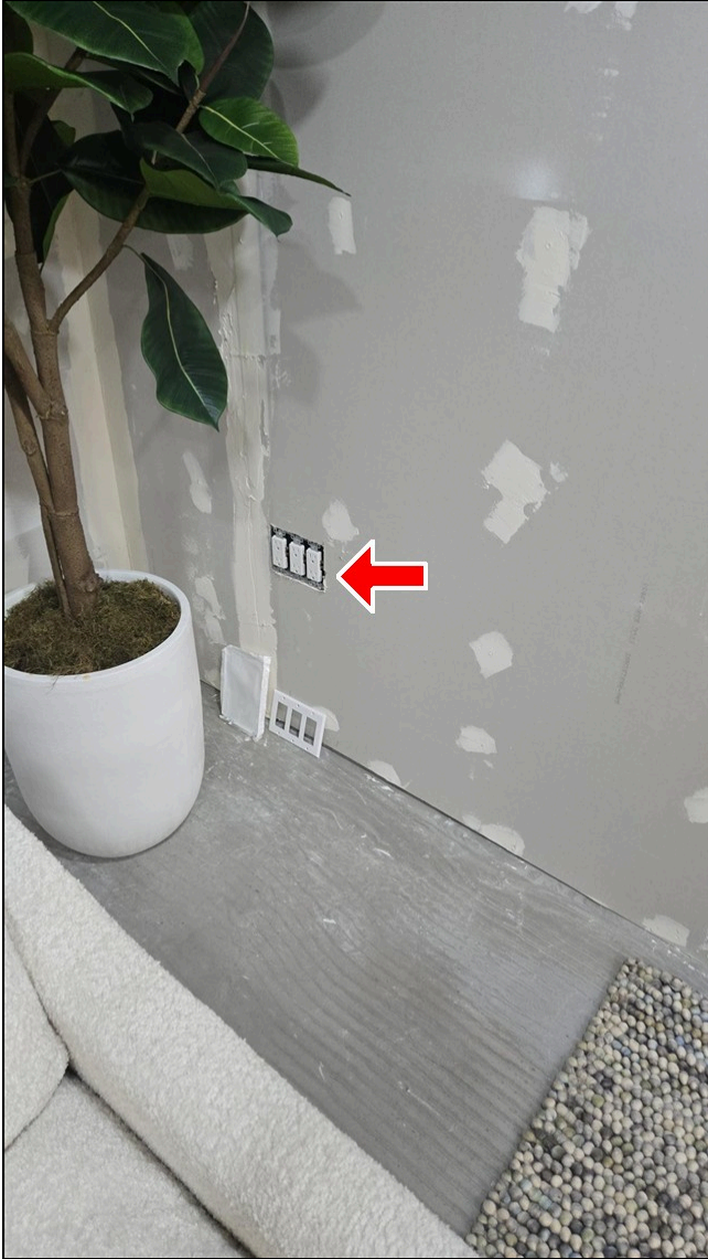
4.4 Item 1 (Picture) Missing cover plates, basement
