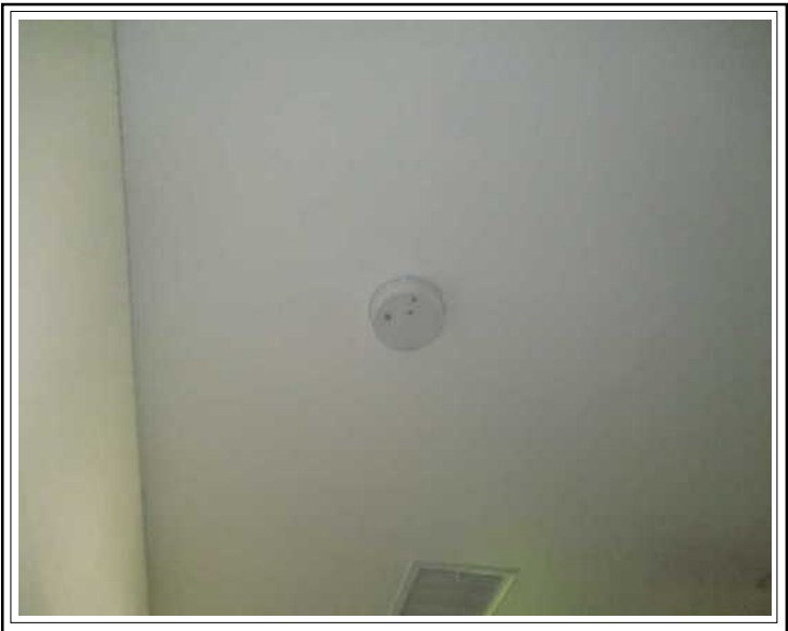
SMOKE/CARBON MONOXIDE DETECTOR BEDROOM#4
