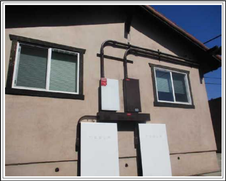
SOLAR PANEL CONTROLS AND BATTERIES
