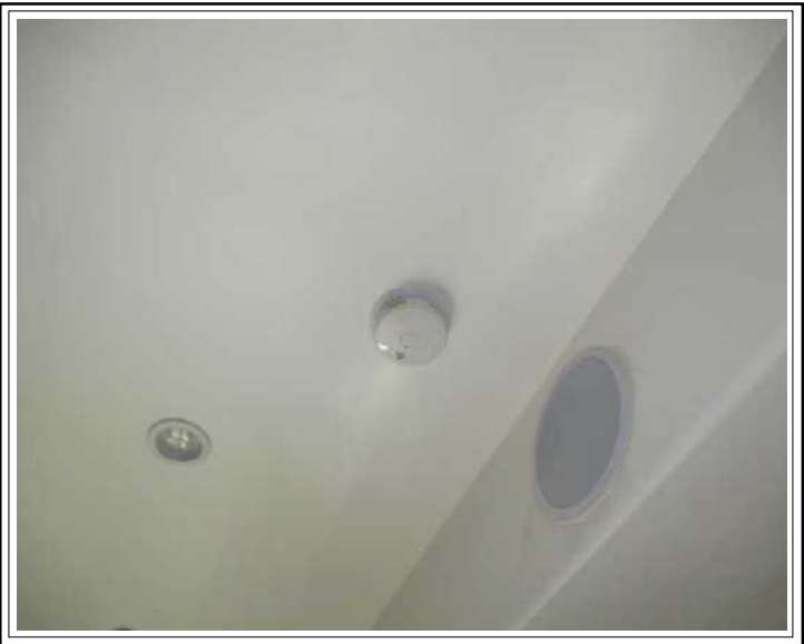
SMOKE/CARBON MONOXIDE DETECTOR BEDROOM#3
