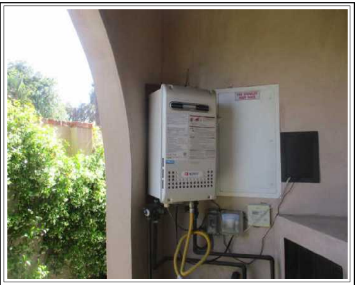
2ND TANKLESS WATER HEATER
