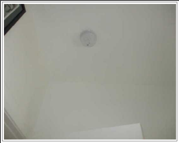
SMOKE/CARBON MONOXIDE DETECTOR BEDROOM#1
