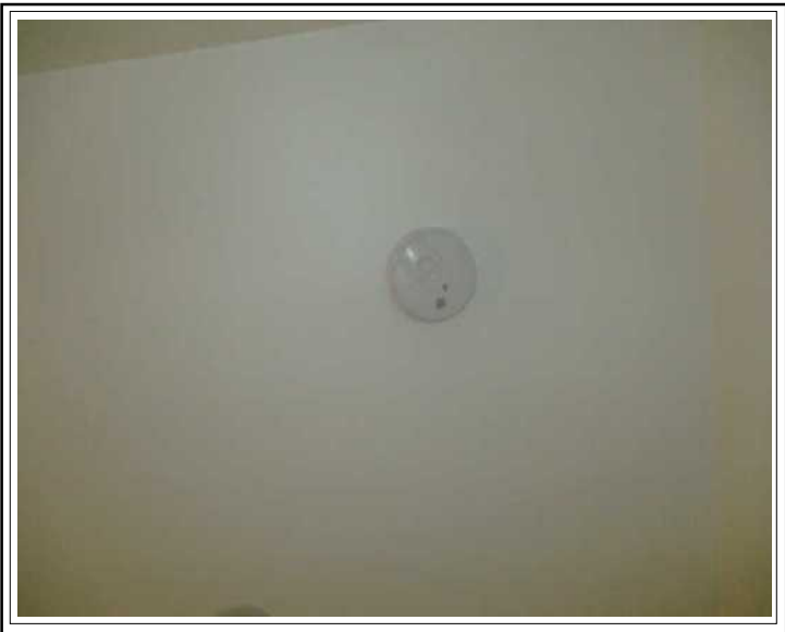
SMOKE/CARBON MONOXIDE DETECTOR BEDROOM#2
