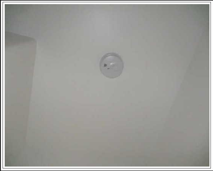
SMOKE/CARBON MONOXIDE DETECTOR FAMILY ROOM
