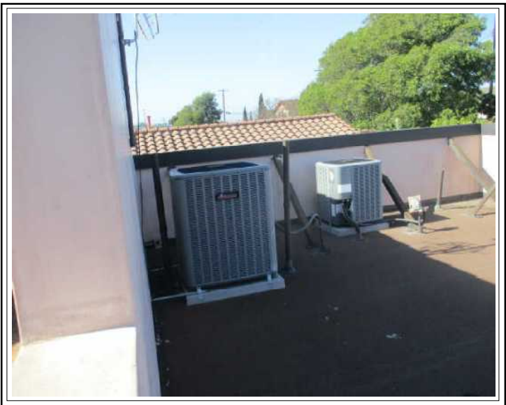
2 AIR CONDITIONING UNITS
