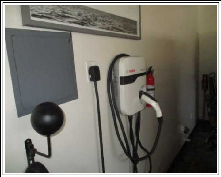
CAR CHARGER IN GARAGE
