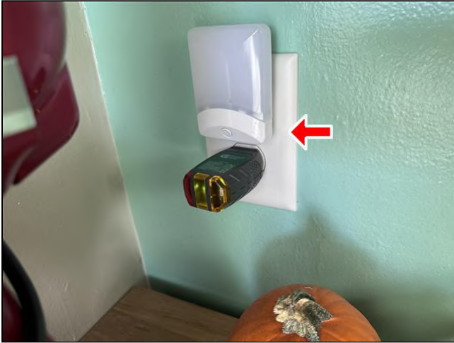
Item 58 - Item 1(Picture) Electrical System
