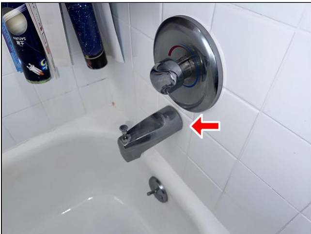
Item 44 - Item 1(Picture) Plumbing System
