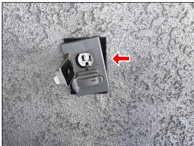
6.2 Item 7(Picture) Electrical System
