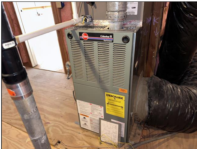
4.0 Item 2(Picture) Heating/Central Air
