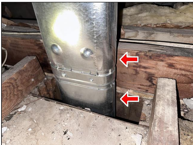
4.3 Item 1(Picture) Heating/Central Air
