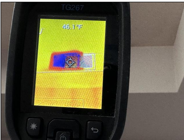
Item 36 - Item 1(Picture) Heating/Central Air
