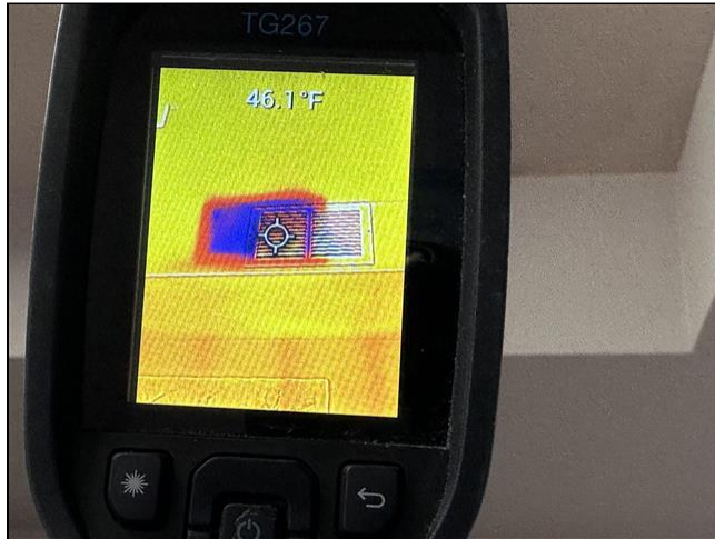
4.7 Item 1(Picture) Heating/Central Air
