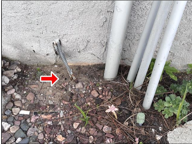
6.0 Item 3(Picture) Electrical System
