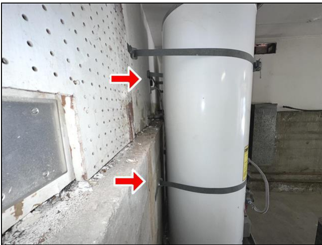
Item 48 - Item 1(Picture) Plumbing System
