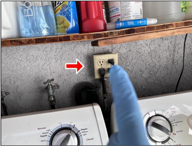
Item 61 - Item 1(Picture) Electrical System
