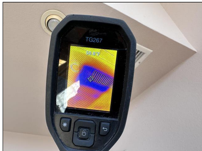
Item 36 - Item 2(Picture) Heating/Central Air
