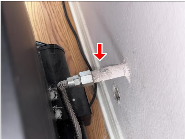
Item 51 - Item 1(Picture) Plumbing System
