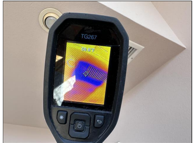
4.7 Item 2(Picture) Heating/Central Air
