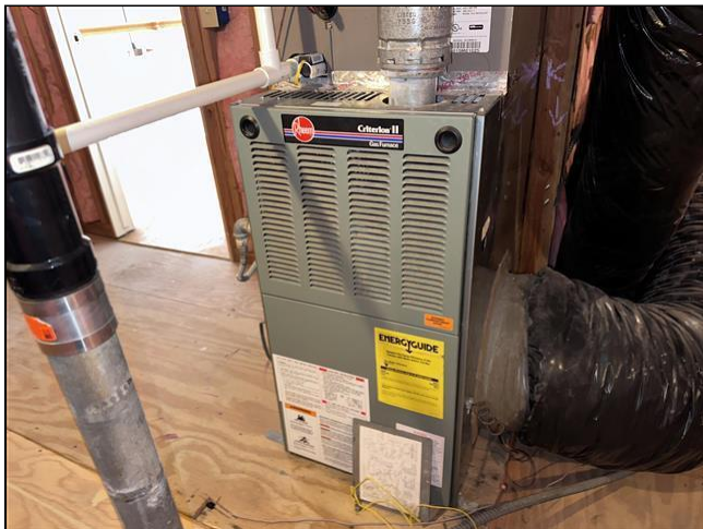
4.0 Item 6(Picture) Heating/Central Air
