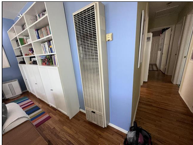
4.0 Item 4(Picture) Heating/Central Air
