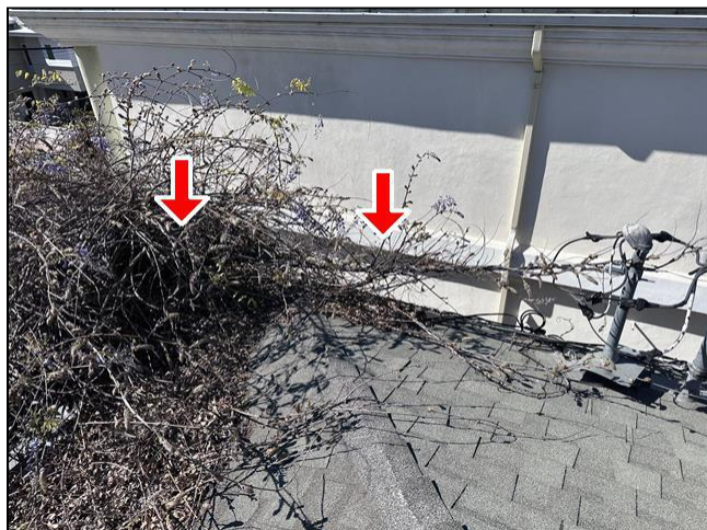
6.0 Item 2(Picture) Electrical System
