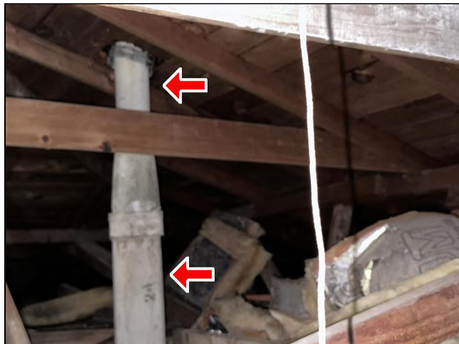
4.3 Item 3(Picture) Heating/Central Air
