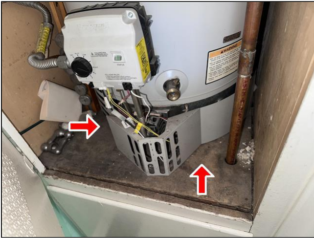
Item 47 - Item 1(Picture) Plumbing System
