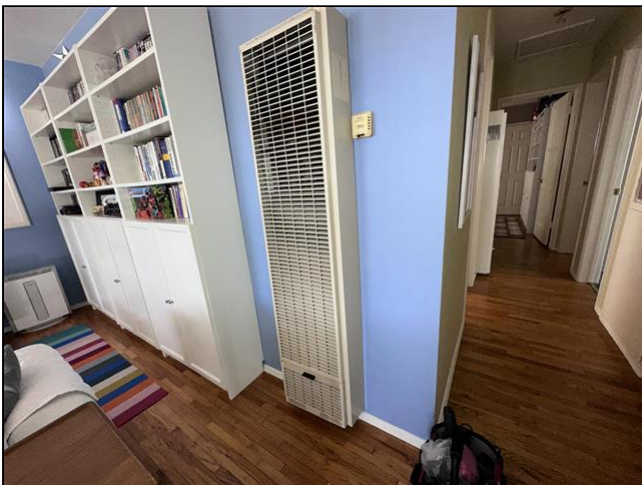
Item 32 - Item 1(Picture) Heating/Central Air
