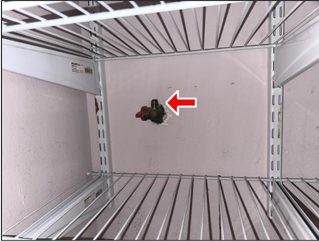
Item 50 - Item 1(Picture) Plumbing System
