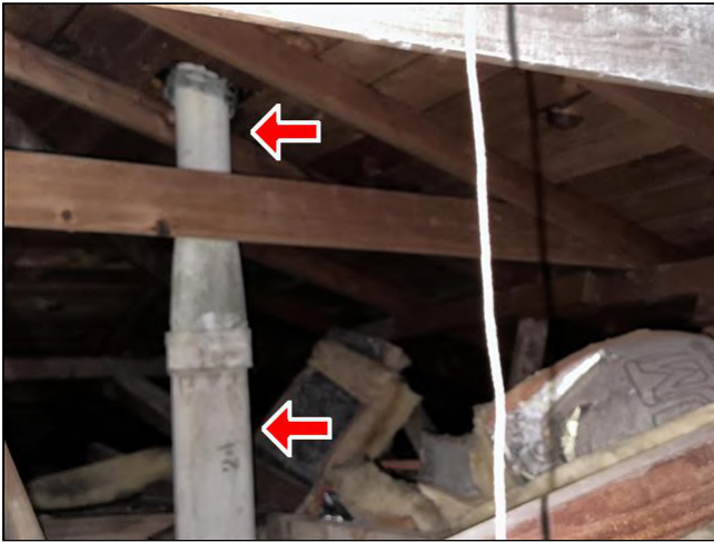
Item 35 - Item 1(Picture) Heating/Central Air Cooling and Air Handler Equipment
