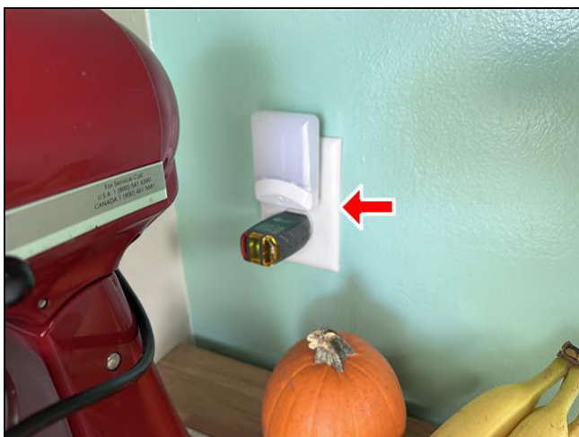
Item 57 - Item 1(Picture) Electrical System
