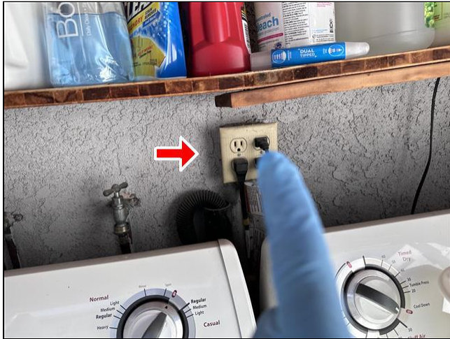
6.2 Item 5(Picture) Electrical System
