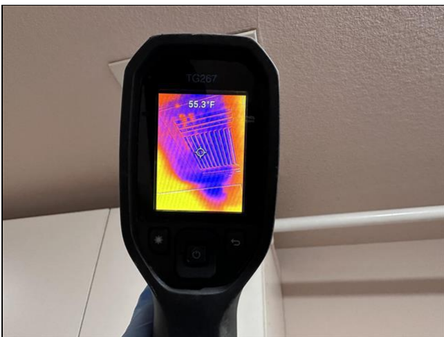
Item 36 - Item 3(Picture) Heating/Central Air
