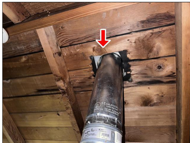
4.3 Item 2(Picture) Heating/Central Air
