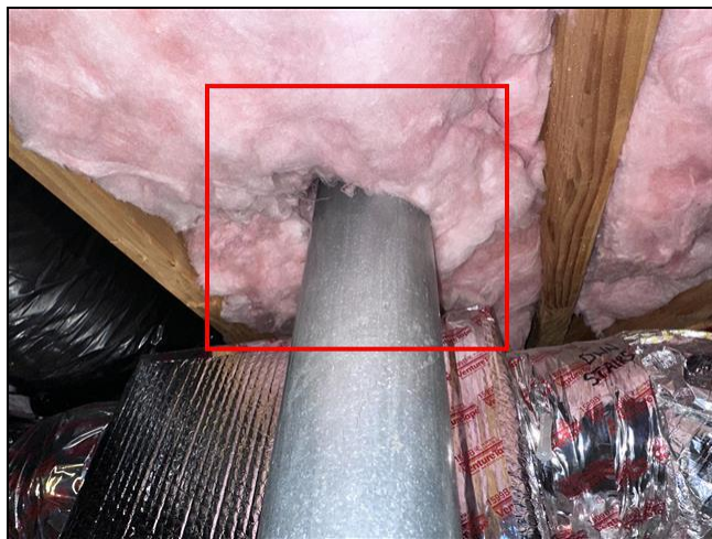
4.3 Item 4(Picture) Heating/Central Air
