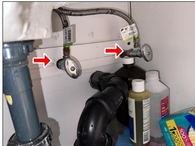
Item 44 - Item 2(Picture) Plumbing System
