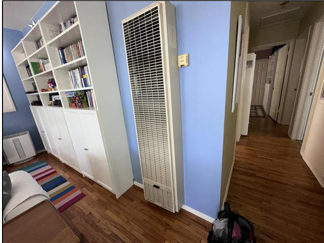
4.0 Item 1(Picture) Heating/Central Air
