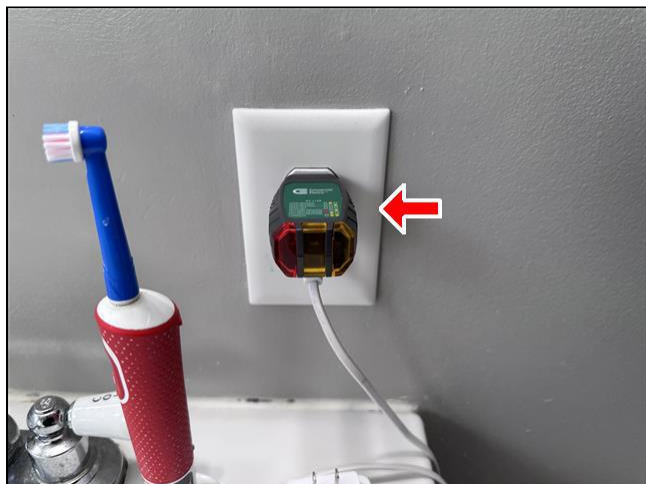
6.2 Item 4(Picture) Electrical System
