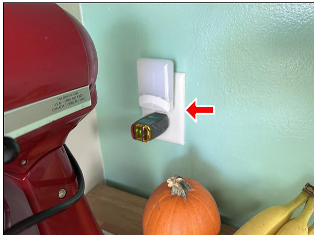
6.2 Item 1(Picture) Electrical System
