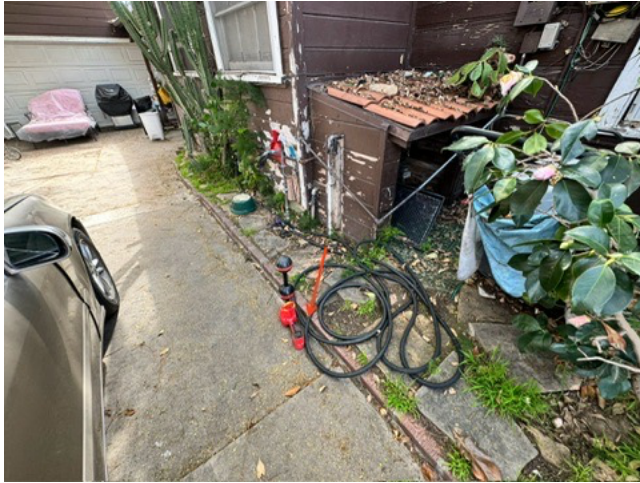
Location where the cast iron pipe exits the house and then transitions into a clay material pipe. Good location for a clean out to be installed under tool.
