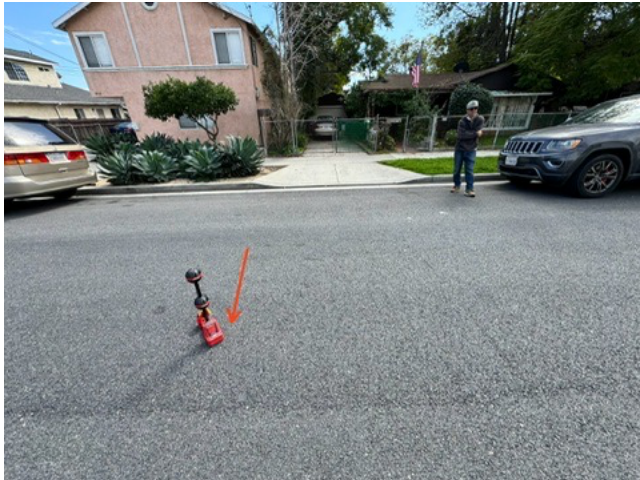
Connection to city sewer under tool.
