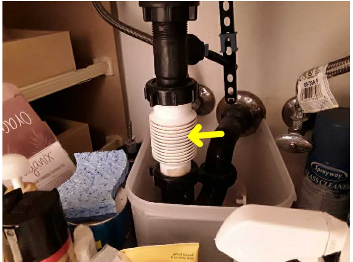
The sink employs an unconventional flexible drainpipe that could contribute to blockages.
