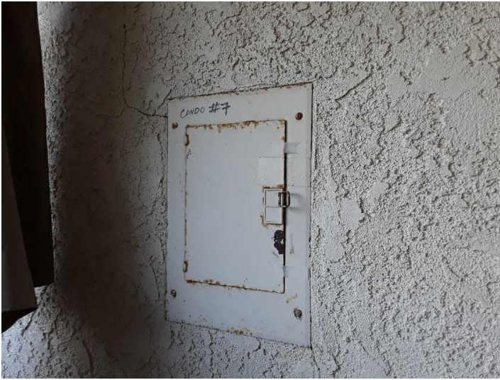
The sub panel is located at the right exterior side of the home.
