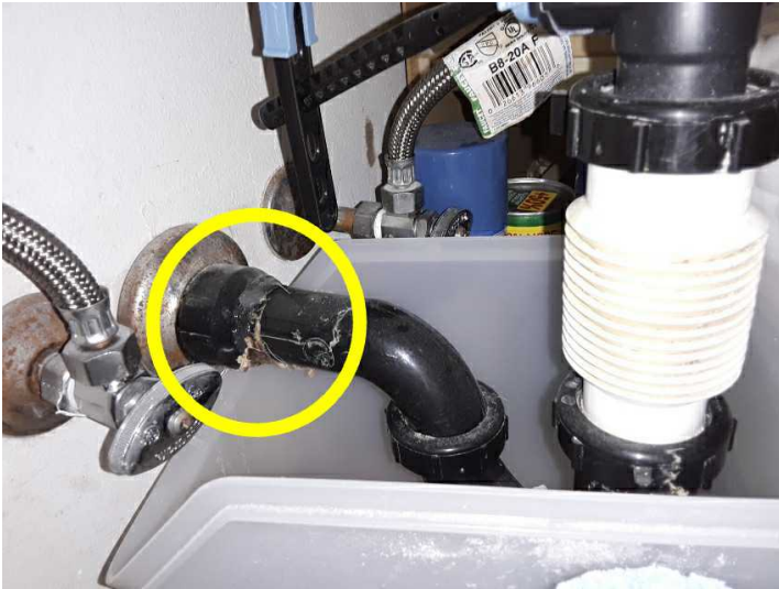
There is a leak at the trap arm below the sink, which should be repaired by a qualified plumbing contractor.
