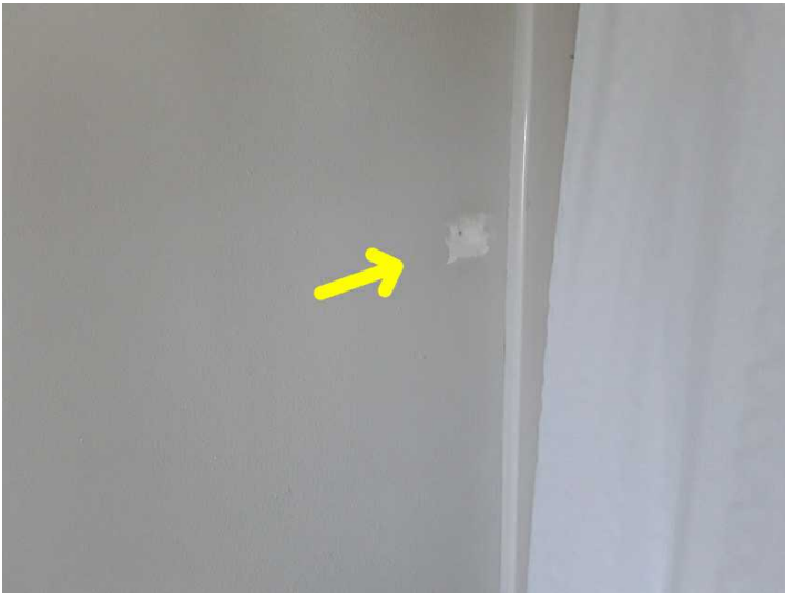
There is moisture damaged drywall adjacent to the tub or shower, which is not uncommon but should be repaired.
